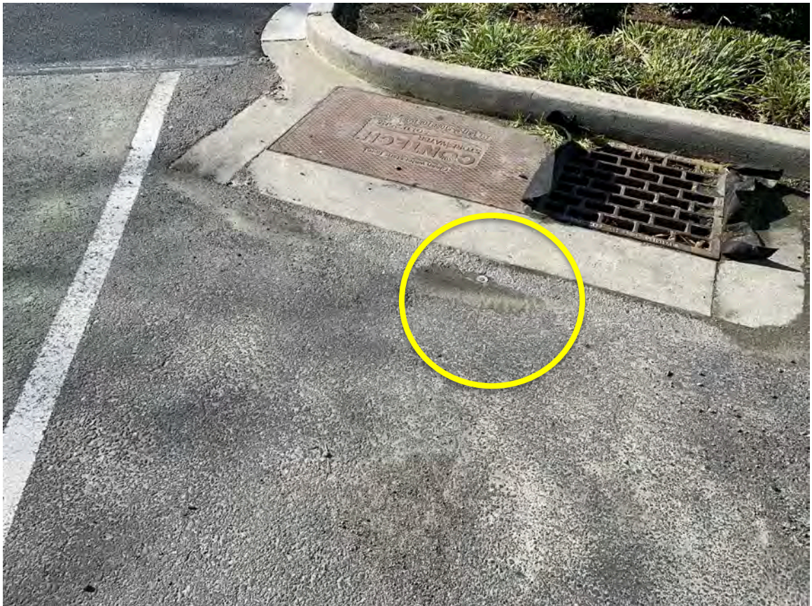
Photograph 5: Pavement Cap Marker "C". Offset from the corner by 4-feet due to utility vault.
