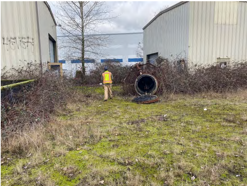
Picture 22 Concrete containment area south of building 2 (left) and abandoned process equipment between buildings 2 and 3 on CleanCare Property
