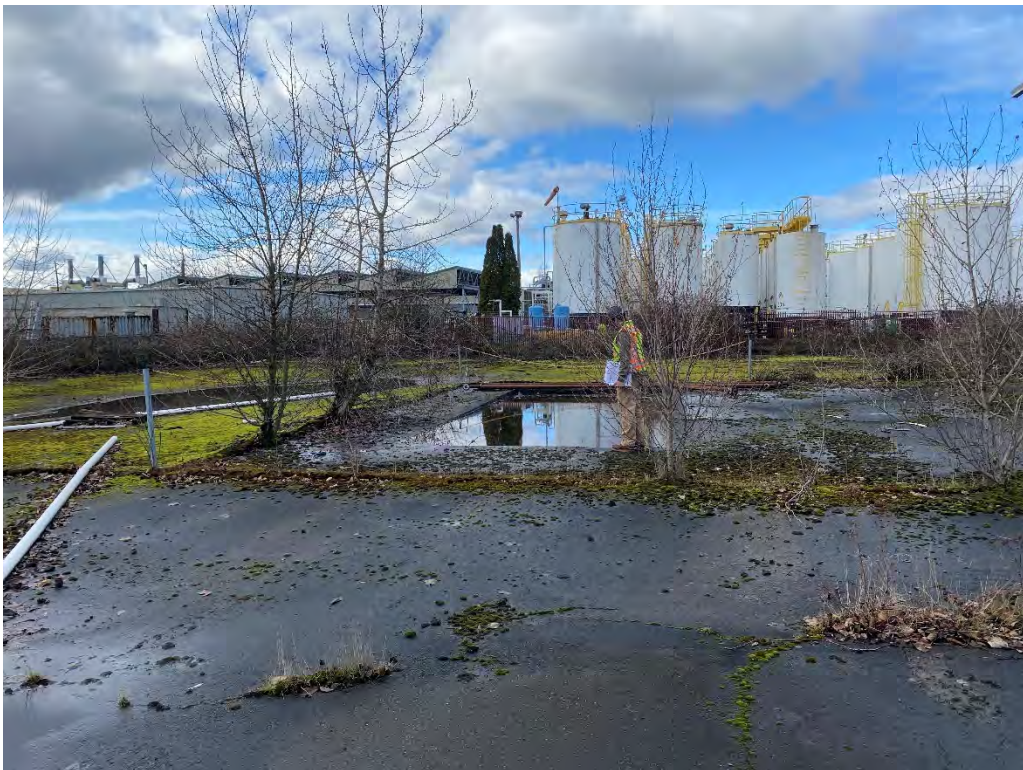
Picture 36 Ponded stormwater in concrete containment area south of former process area on CleanCare Property, Burlington Environmental tank farm in background
