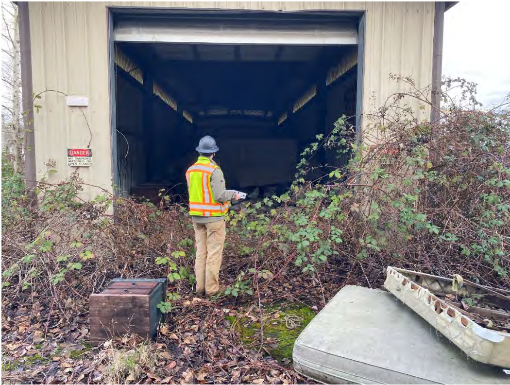
Picture 25 Debris inside and outside south end of building 3 on CleanCare Property
