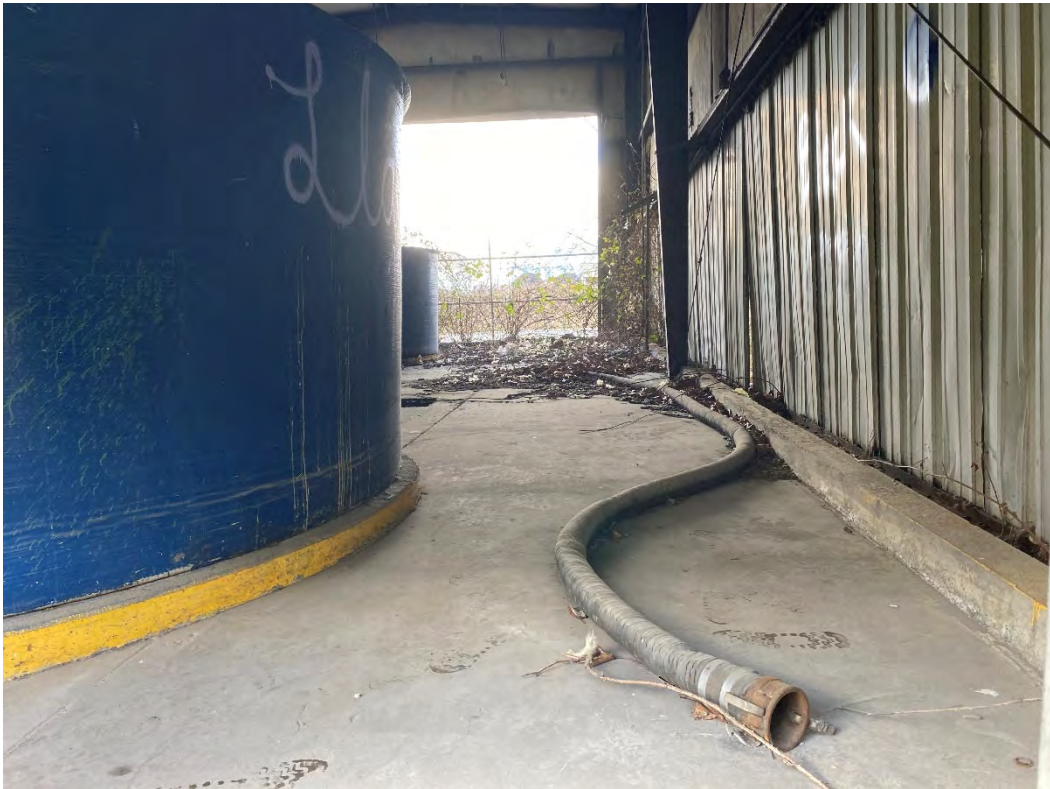
Picture 24 Abandoned fiberglass tanks inside building 2 on CleanCare Property
