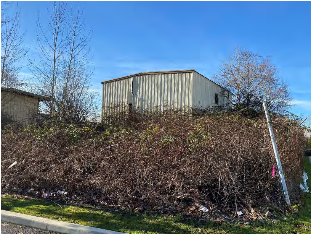
Picture 41 Looking west from 1514 Taylor Way Property toward CleanCare Property, building 3 in background, fencing missing
