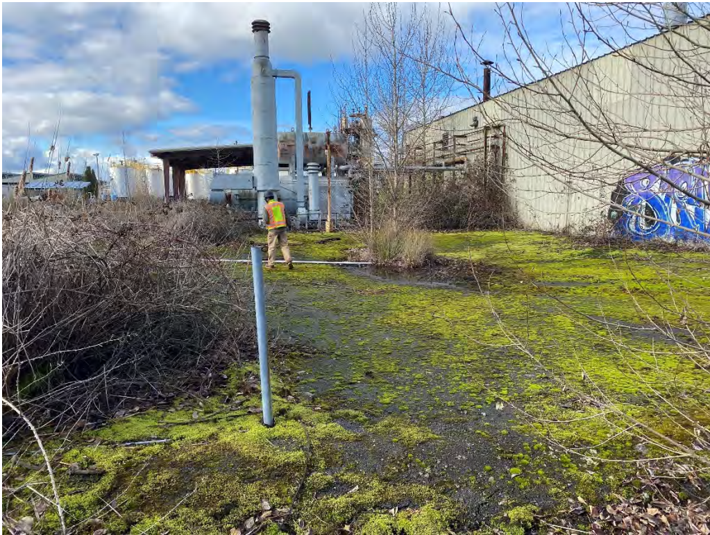
Picture 35 Asphalt depression south of building 1 and north of containment area shown in Picture 34 on Cleancare Property
