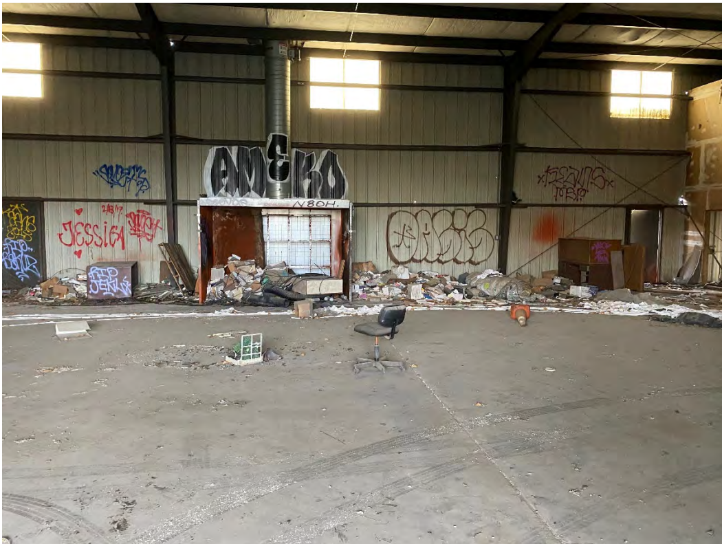
Picture 28 Debris and vandalism inside building 1 on CleanCare Property
