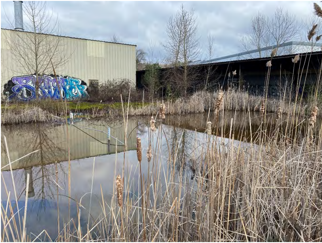
Picture 33 Former concrete containment area south of building 1 full of stormwater on CleanCare Property
