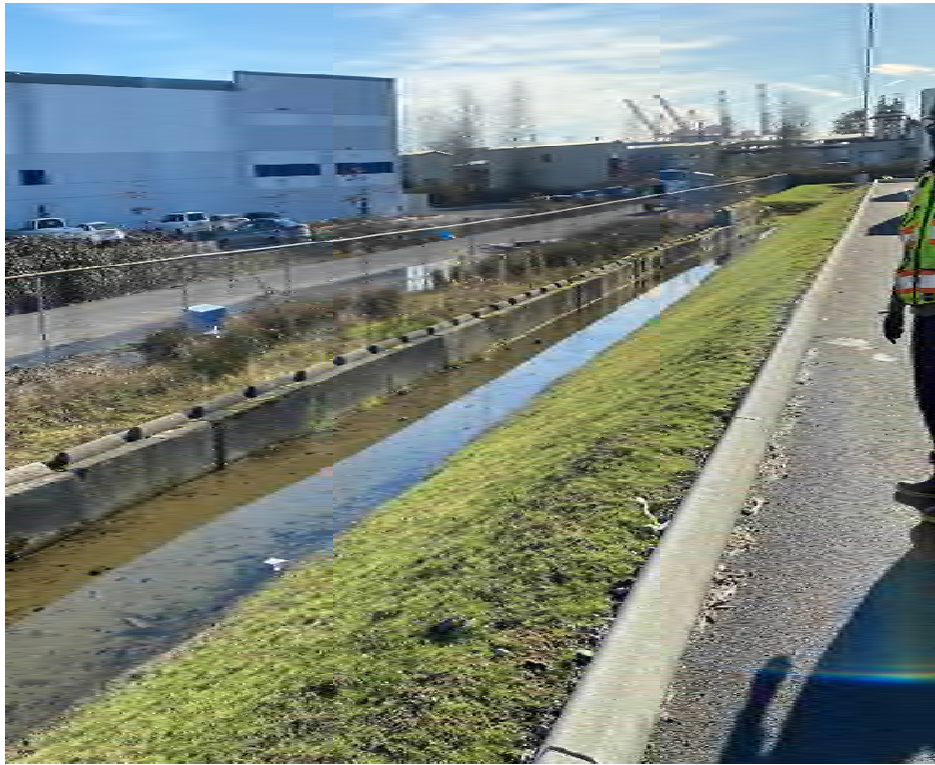
Picture 9 Pondered stormwater along eastern property line, adjacent to northern trailer parking lot on Burlington Environmental Property
