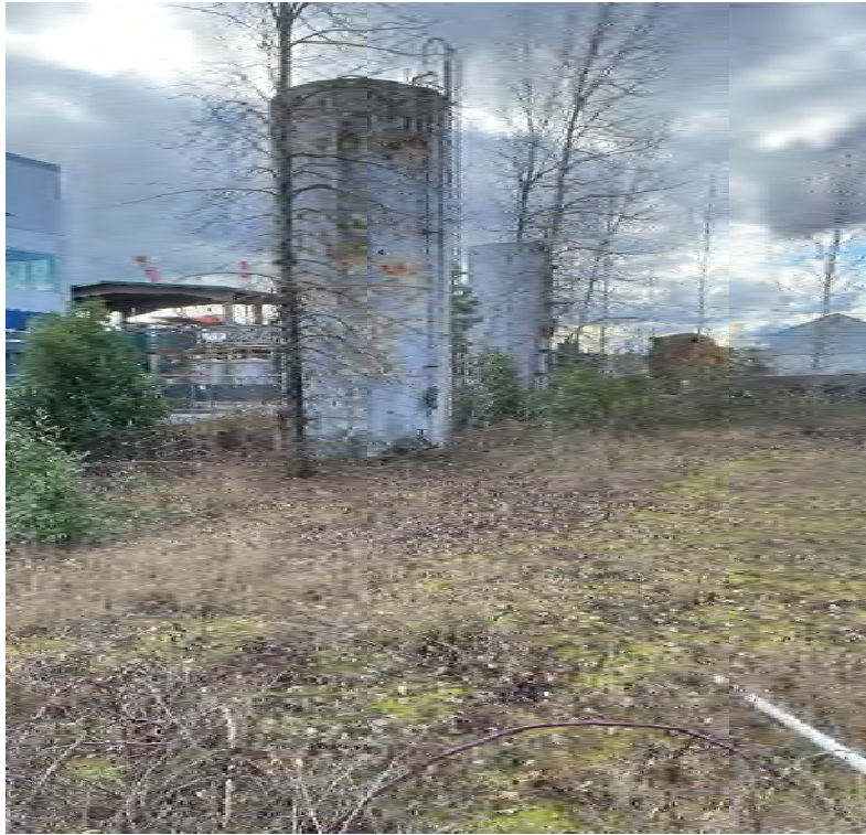
Picture 17 Abandoned tanks on south end of CleanCare Property
