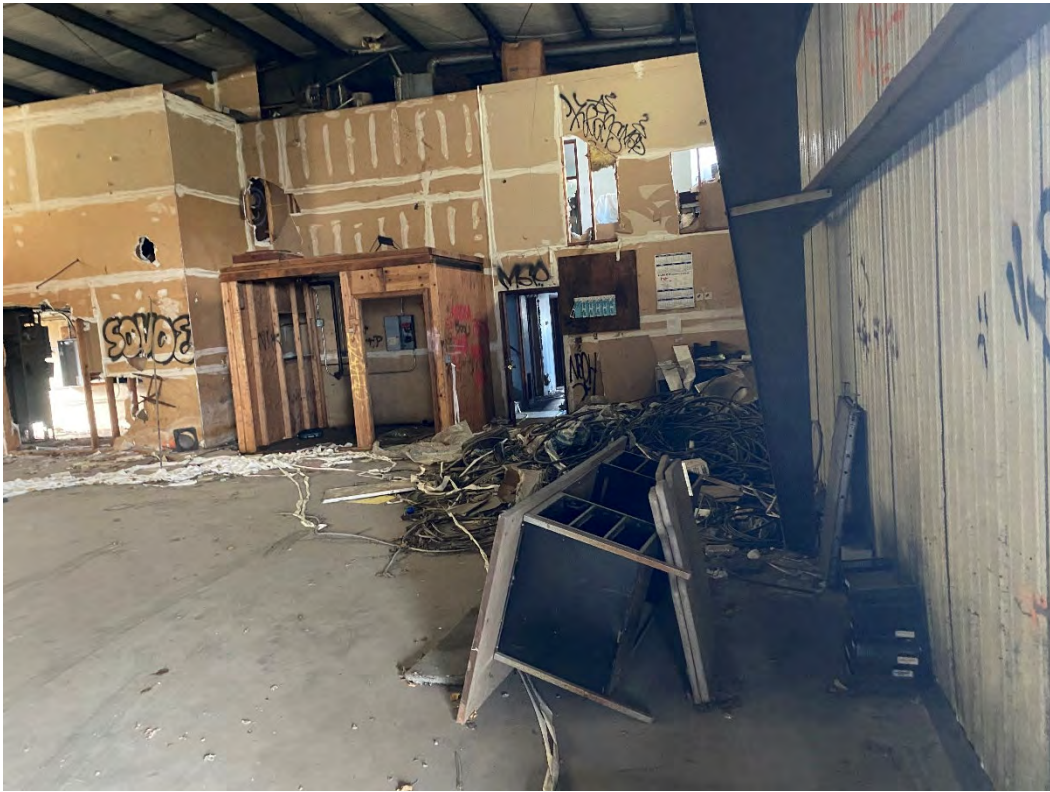
Picture 27 Debris and vandalism inside building 1 on CleanCare Property.
