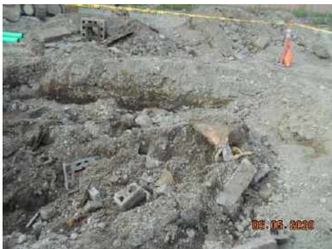
Photograph 15. Discovery of buried construction debris (analytically characterized as asbestos containing material) within the southern portion of the site discovered during sanitary sewer installation.
