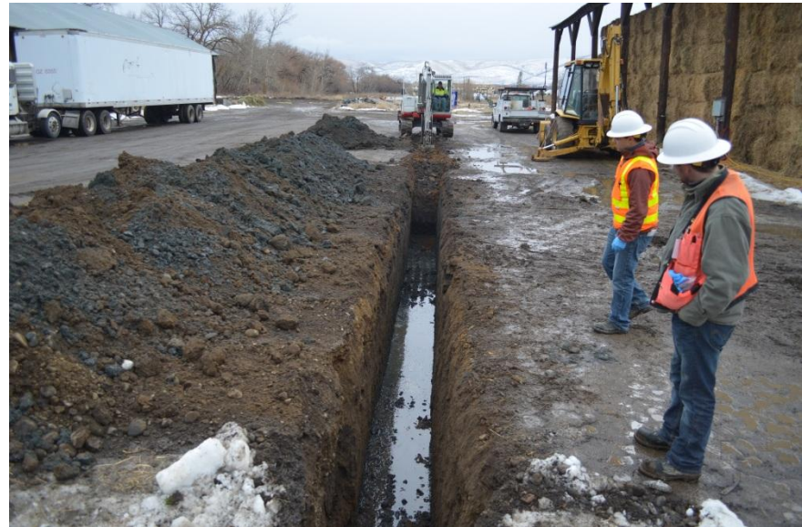
The primary north-south trench excavation extended from the UST basin on the north to the south end of the center hay barn.
