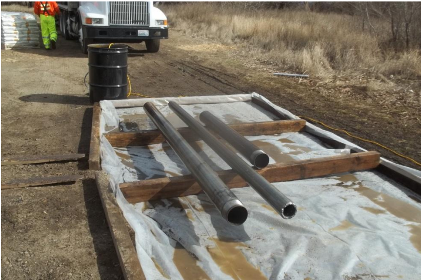
Tooling decontamination area established by Cascade Drilling for washing of boring casing.
