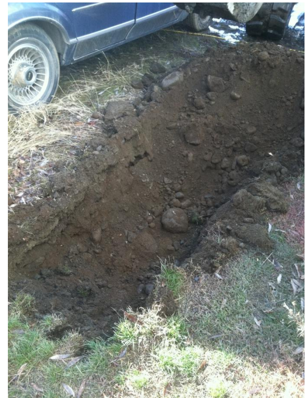
Localized trench excavation completed north of the canopy cover on the east side of the scale house/residence.
