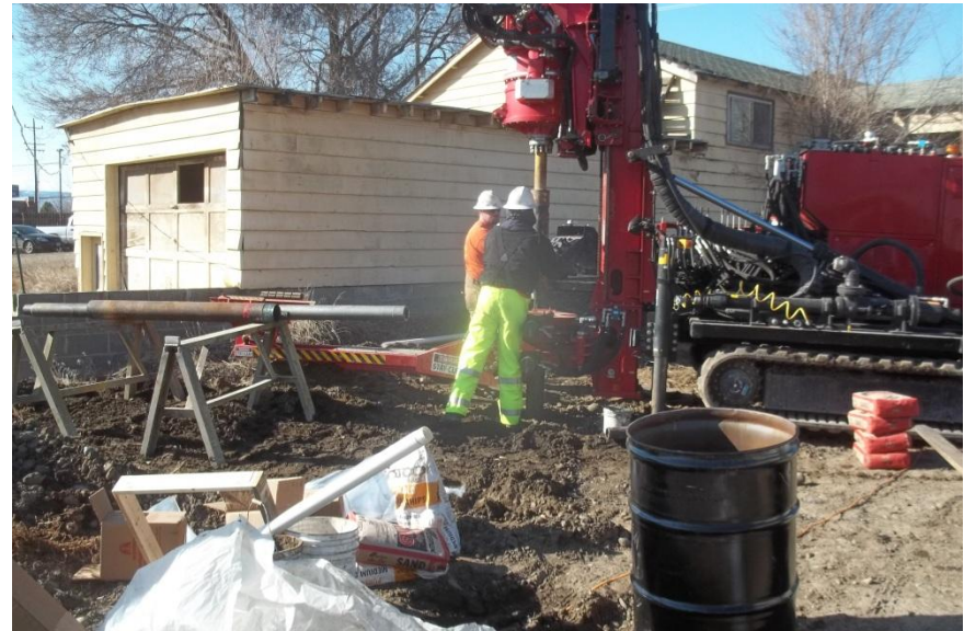
Completion of the boring for MW-02 located southeast of the scale house/residence and within the approximately UST basin.
