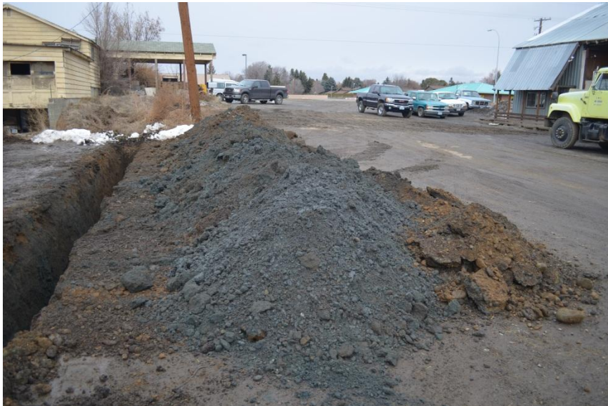
Excavated soils through the former UST basin and south of the telephone pole were heavy discolored with a noticeable odor.
