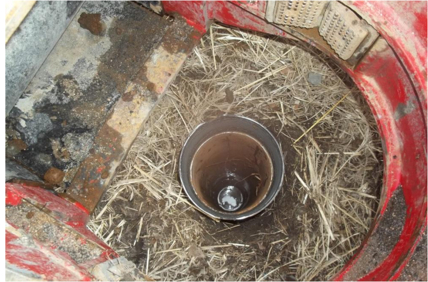
Visible casing for one of the boreholes with groundwater present in the casing and prior to installation of PVC casing.
