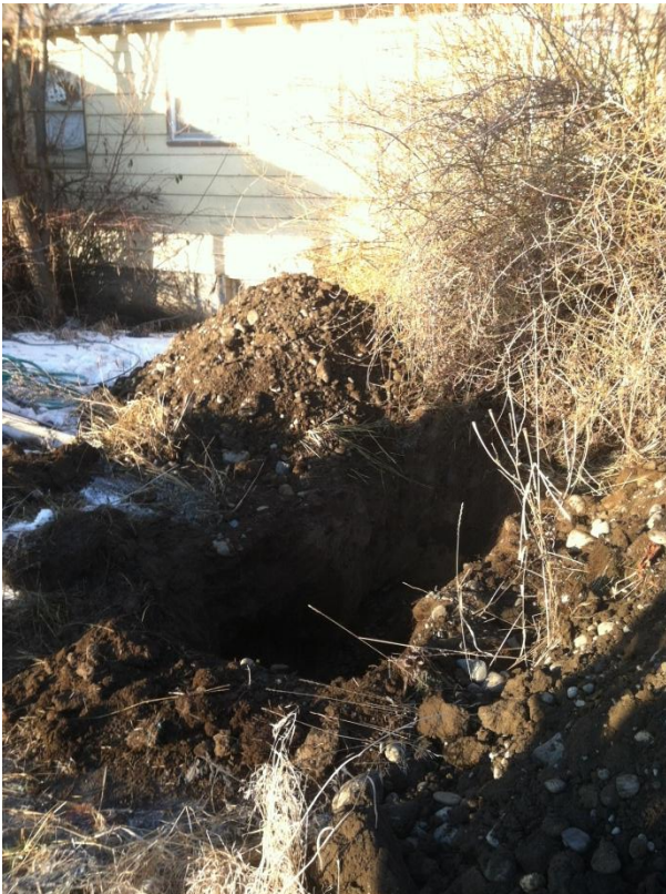
First trench excavation, beginning at the scale house/residence and continuing east towards the shop building.
