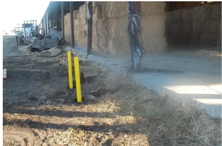
Monitoring Well 05 with bollards placed for protection prior to well development and completion of the concrete mounting pedestal.
