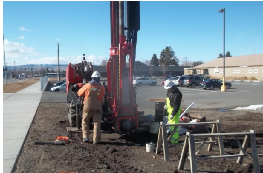
Completion of the boring for Monitoring Well 01, located north and offsite on private property.
