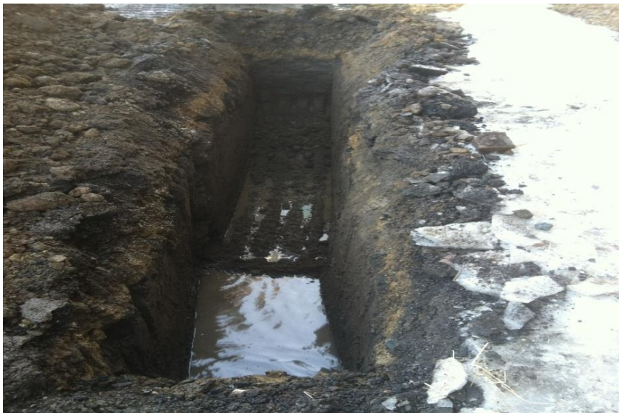
Groundwater accumulation was visible in portions of the site during excavation activities.
