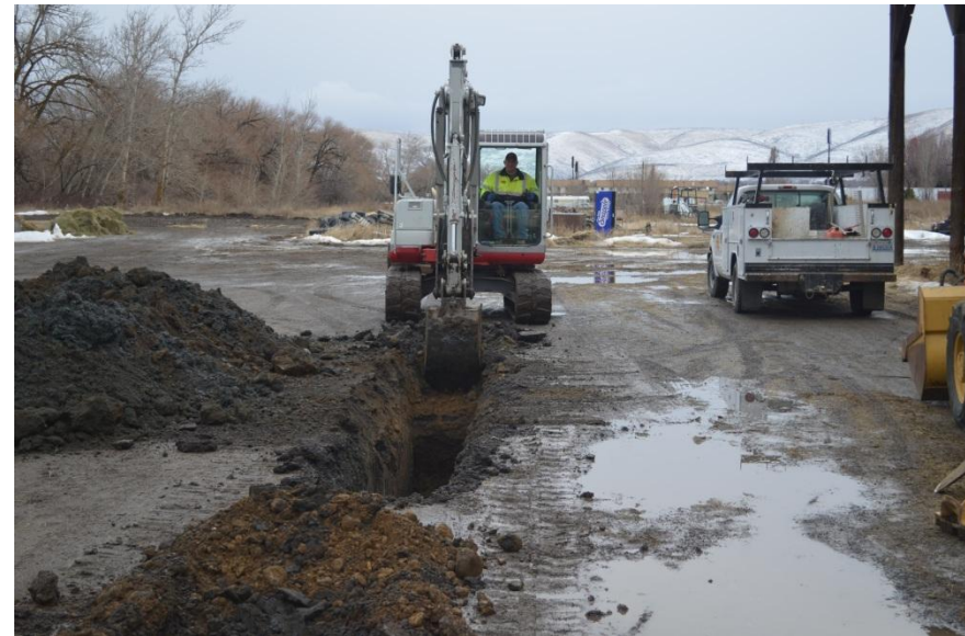
South extent of the trench excavation that extended from the UST basin on the north to the south end of the center hay barn.
