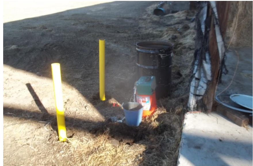
Well development utilized a peristaltic pump for purging of water from each monitoring well.
