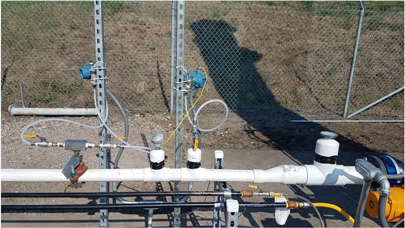
October 2, 2020 – Rosemount flow transmitters
