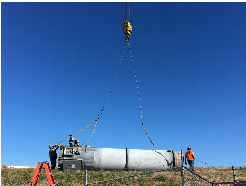
September 28, 2020 – connecting flare to lift cables prior to placement on truck for transport
