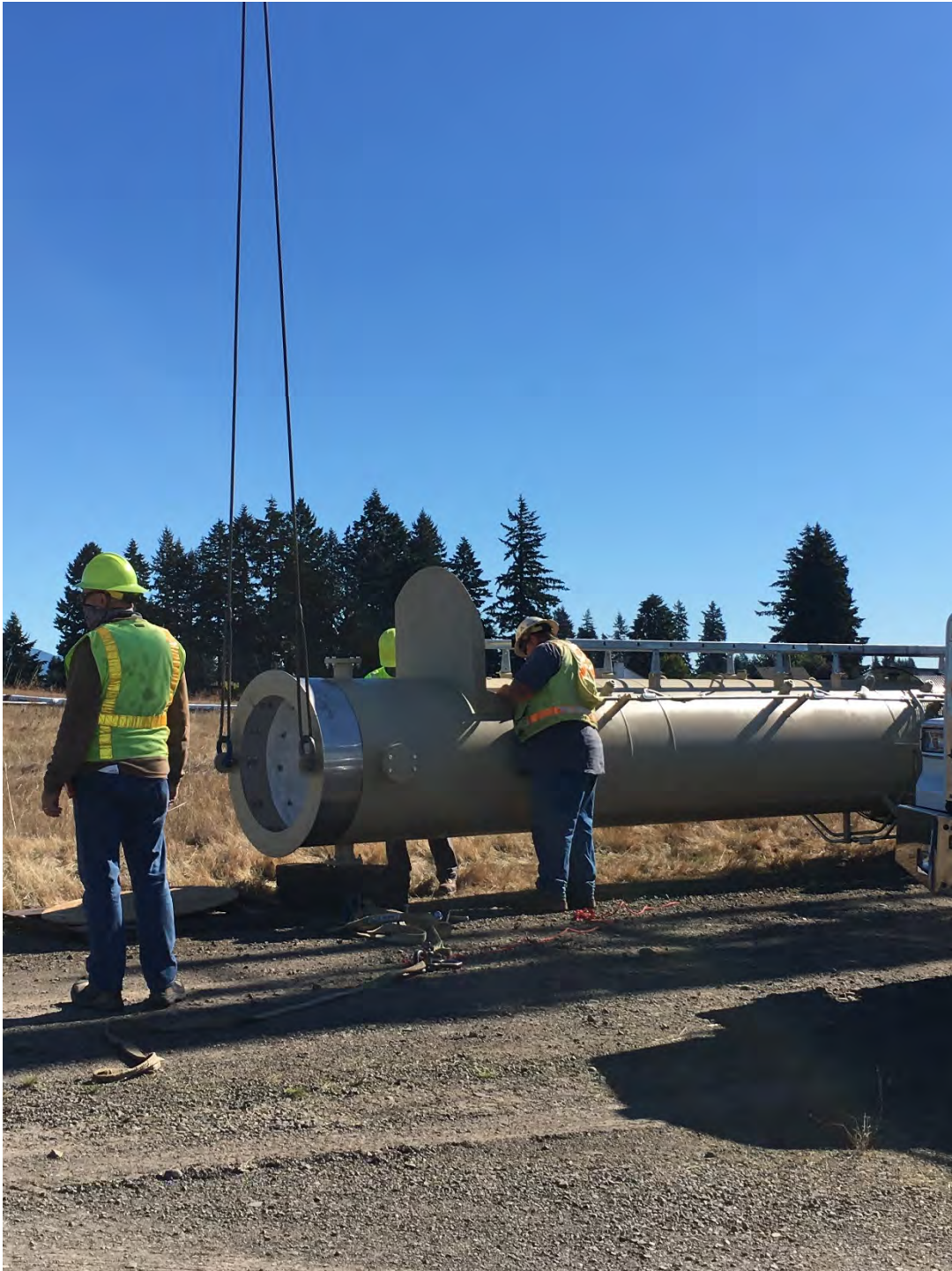
September 28, 2020 – connections to lifting lugs and getting ready to lift flare to flare pad
