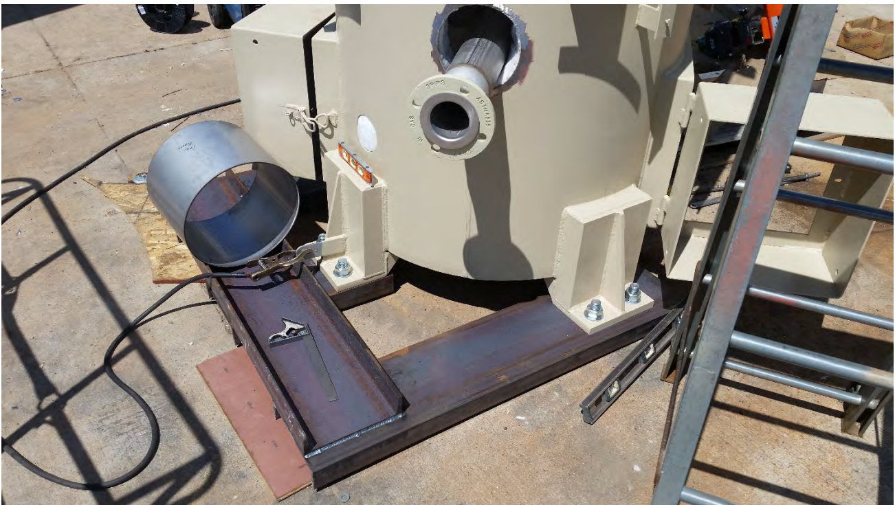
August 25, 2020 – Flare feet bolted to shipping stand and burner inlet placed prior to welding at Perennial manufacturing facility
