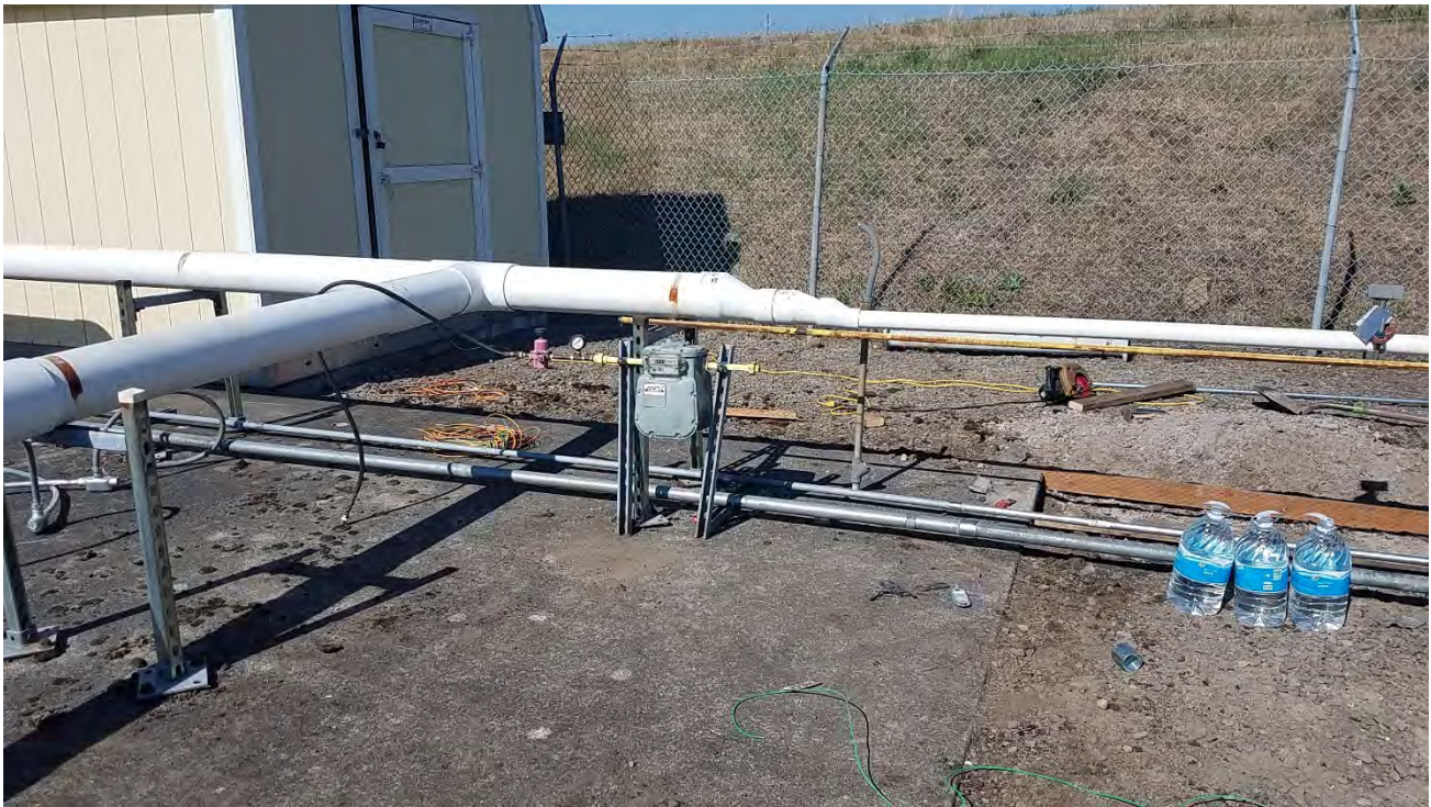
September 30, 2020 - GCCS piping to flare inlet
