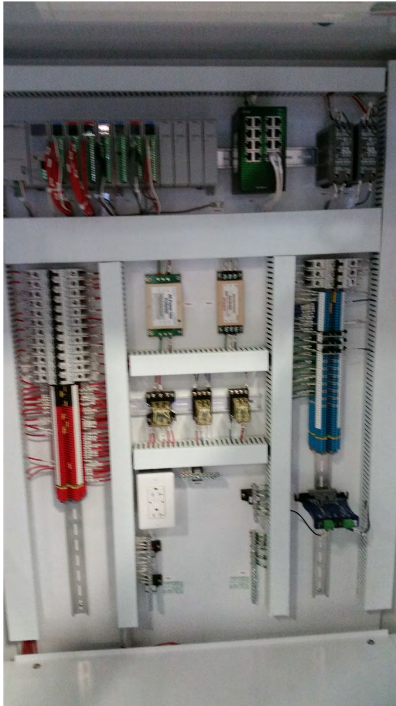
September 24, 2020 – Inside flare control panel prior to shipment at Perennial manufacturing facility
