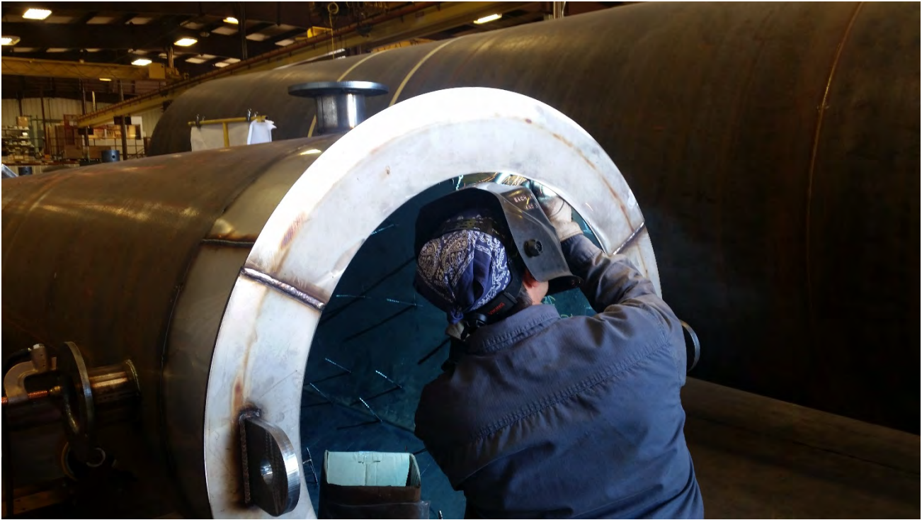
August 20, 2020 – installation of flare installation pins during construction at Perennial manufacturing facility
