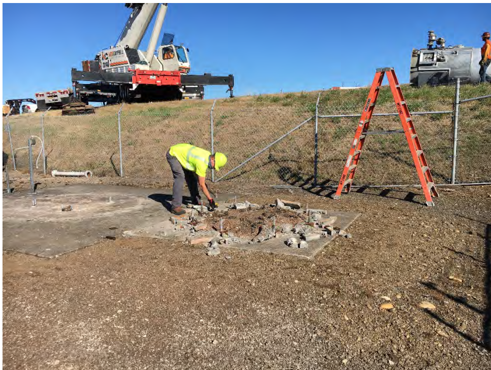
September 28, 2020 – cleanup of old flare pad (right) prior to placement of new flare on new flare pad (left)
