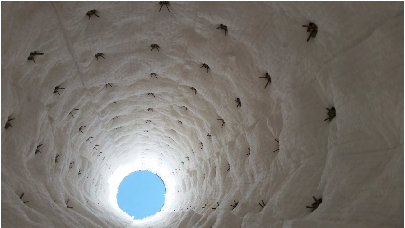
August 25, 2020 – Looking up flare stack with flare insulation at Perennial manufacturing facility
