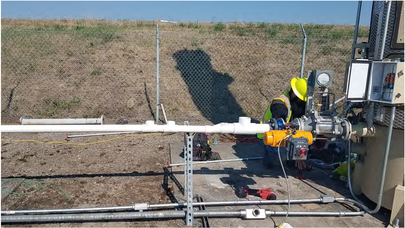
September 30, 2020 - GCCS piping to flare inlet
