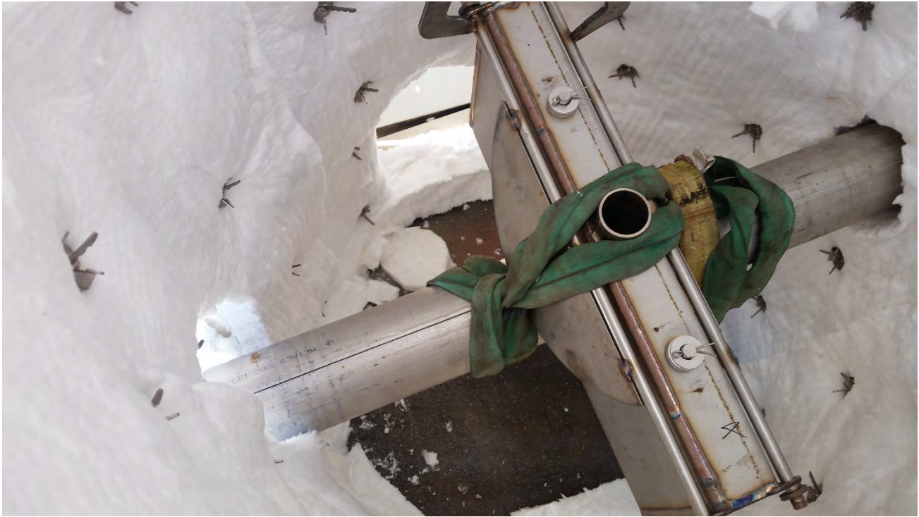
August 25, 2020 – Flare burner manifold at Perennial manufacturing facility
