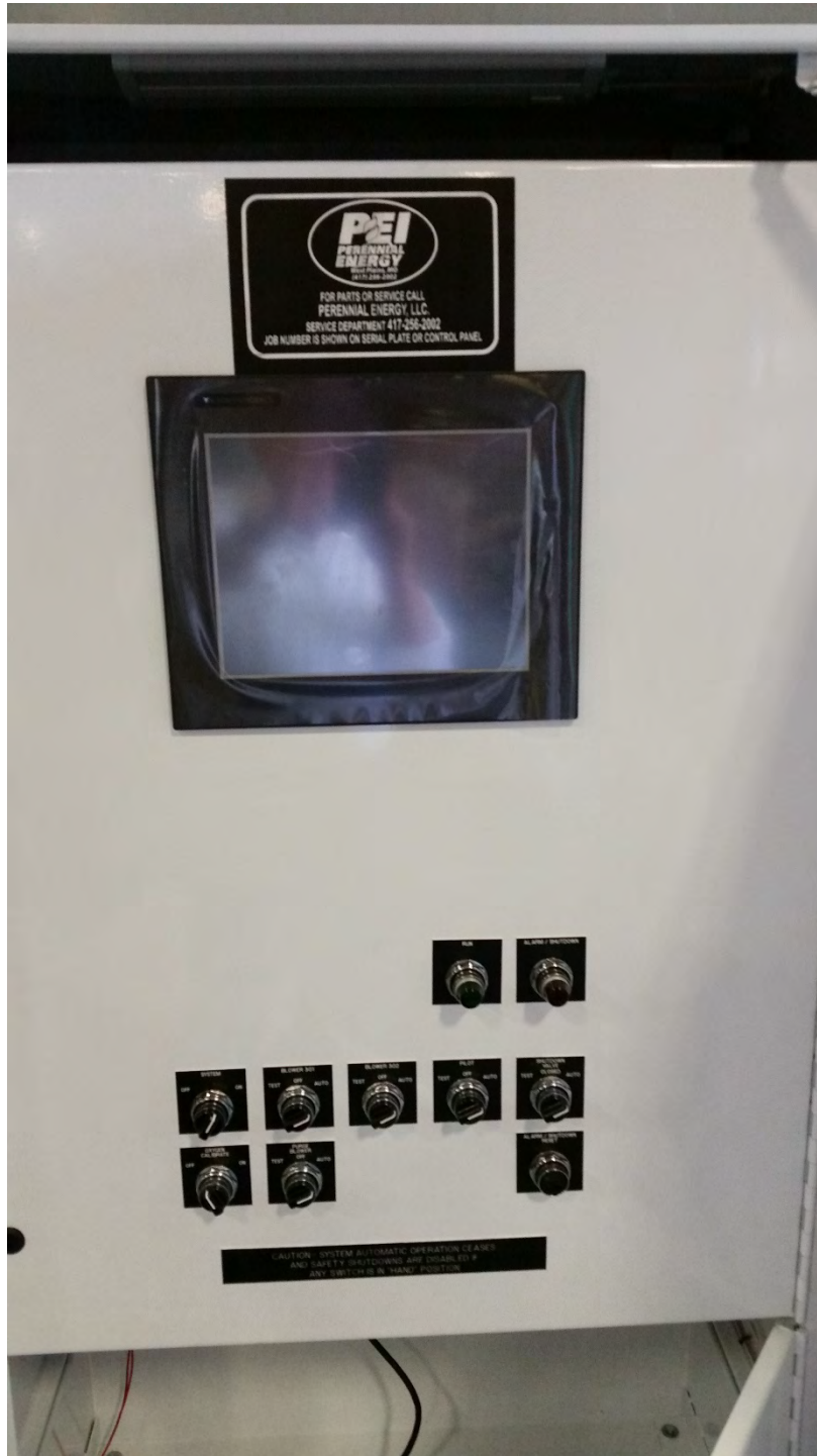
September 24, 2020 - Flare control panel prior to shipment at Perennial manufacturing facility
