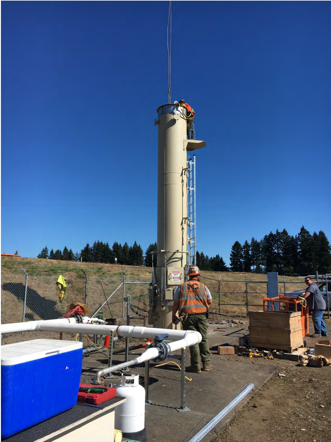
September 28, 2020 – removal of lifting cables after flare alignment on flare pad and preparation for burner pot placement
