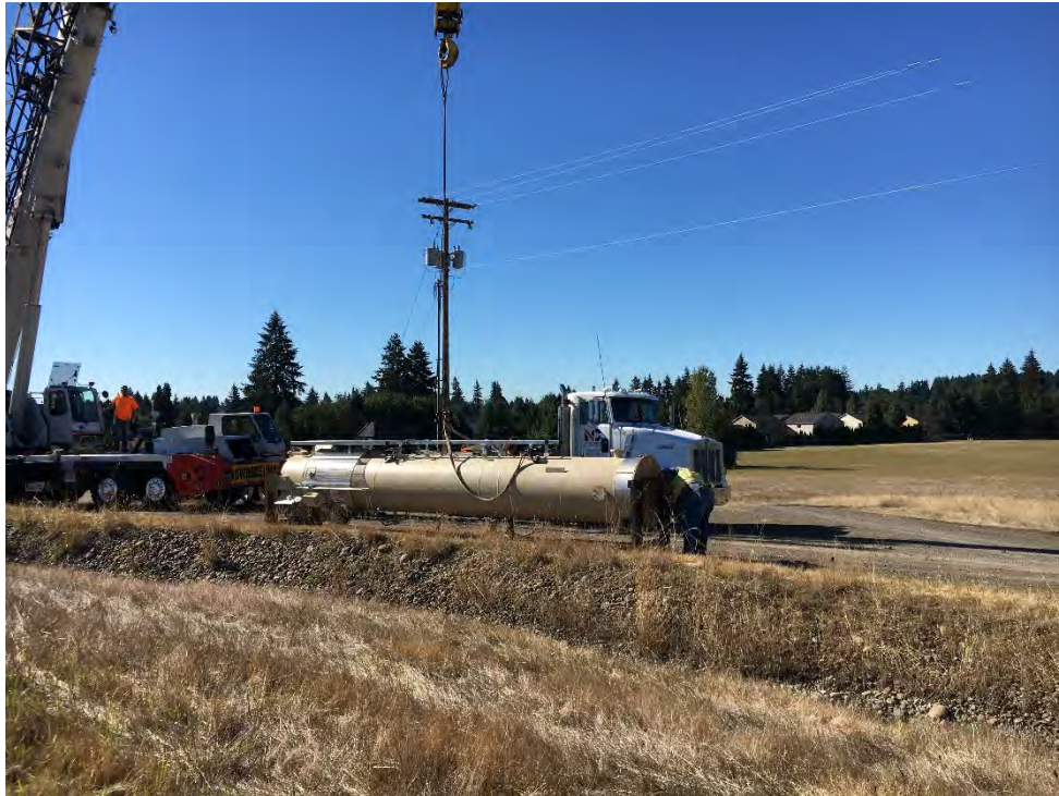
September 28, 2020 – flare on ground to remove shipping stand and connect flare at lifting lugs for placement on flare pad
