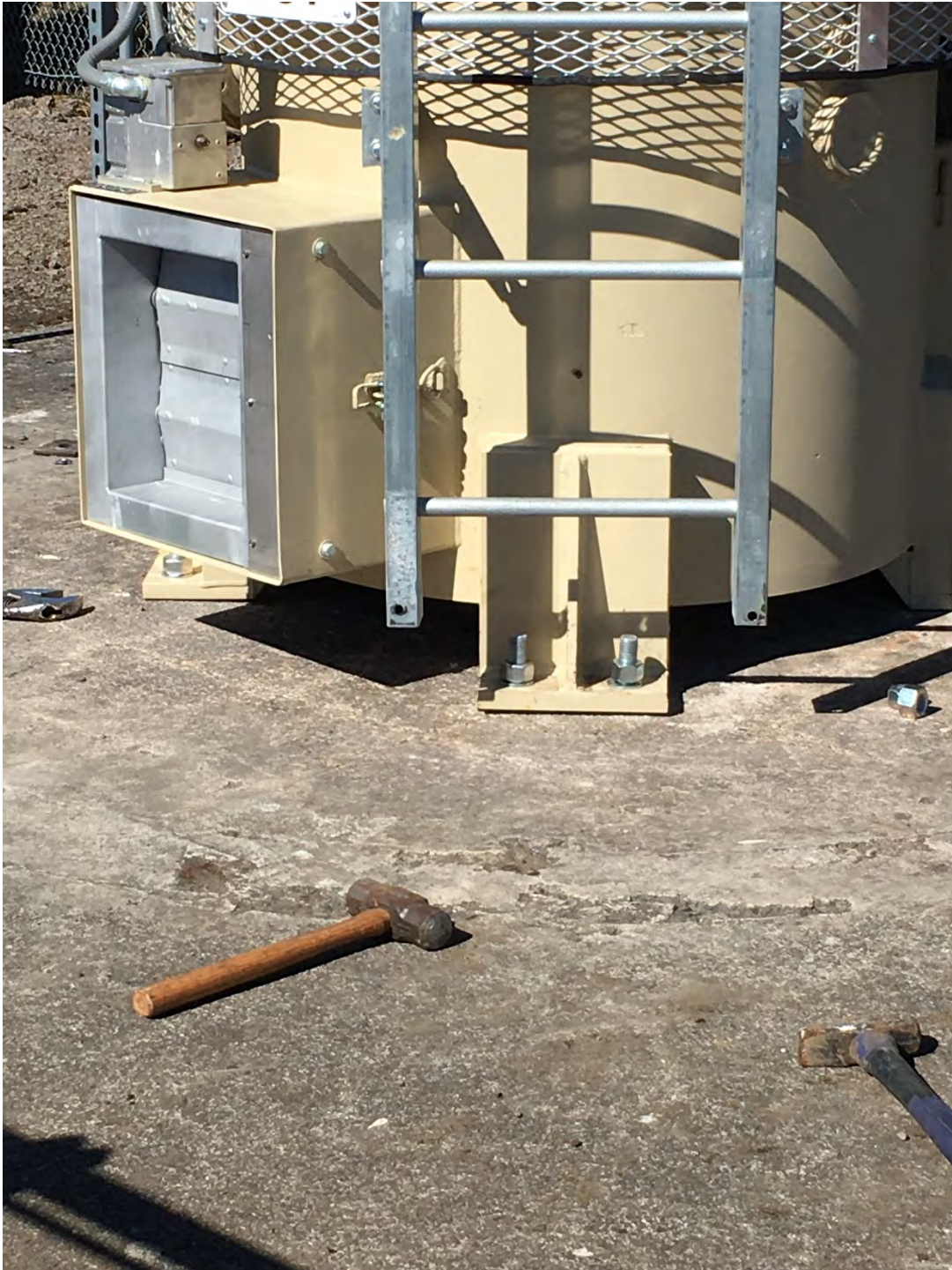
September 28, 2020 – alignment of flare feet on flare pad after enlargement of bolt holes
