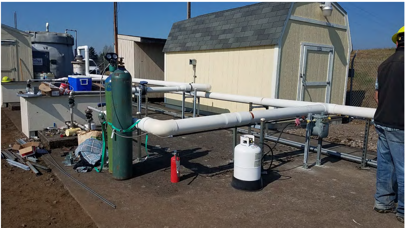
October 2, 2020 – GCCS piping and nitrogen tanks
