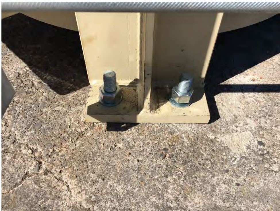
September 28, 2020 – flare foot where bolt holes were enlarged for alignment purposes
