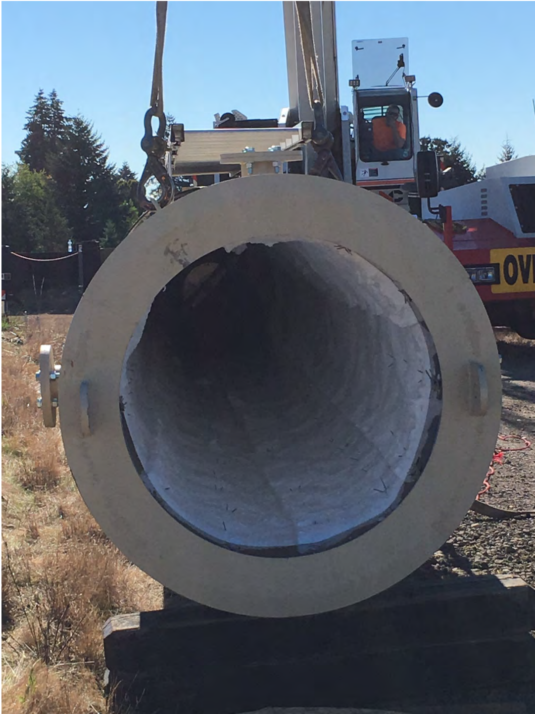
September 28, 2020 – looking inside flare from top
