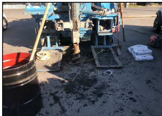
View looking southwest across site, a drill rig can be seen installing the new MW-06 monitoring well in the background.
