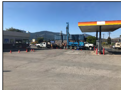
View looking southwest across site, a drill rig can be seen installing the new MW-04 well in the background.
