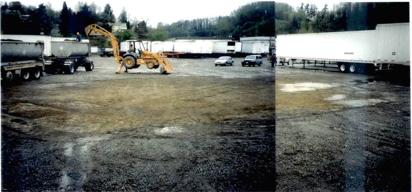
Diese Spill Area Following Removal Action View to North (4/6/96)
