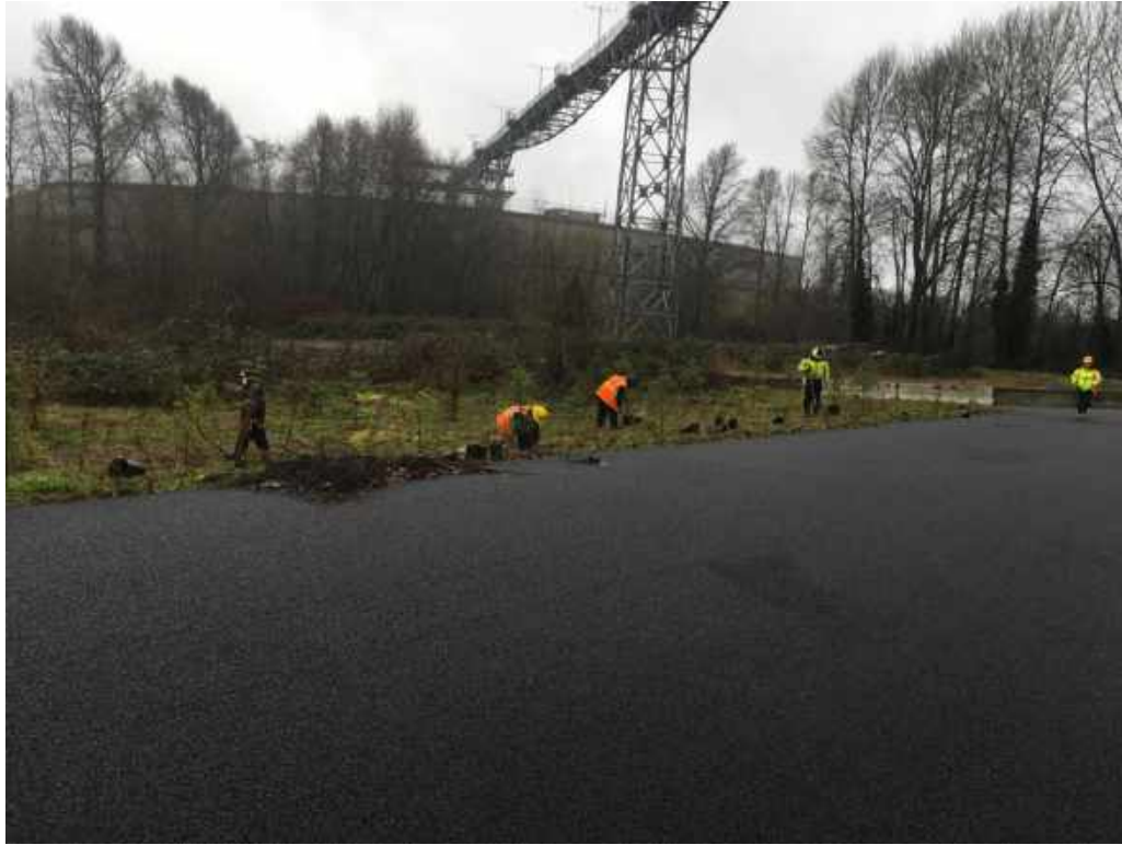
Photograph 1. Port crew performing maintenance of the planted filter strip just south of the 1982 Dredged Material Containment Area (DMCA).
