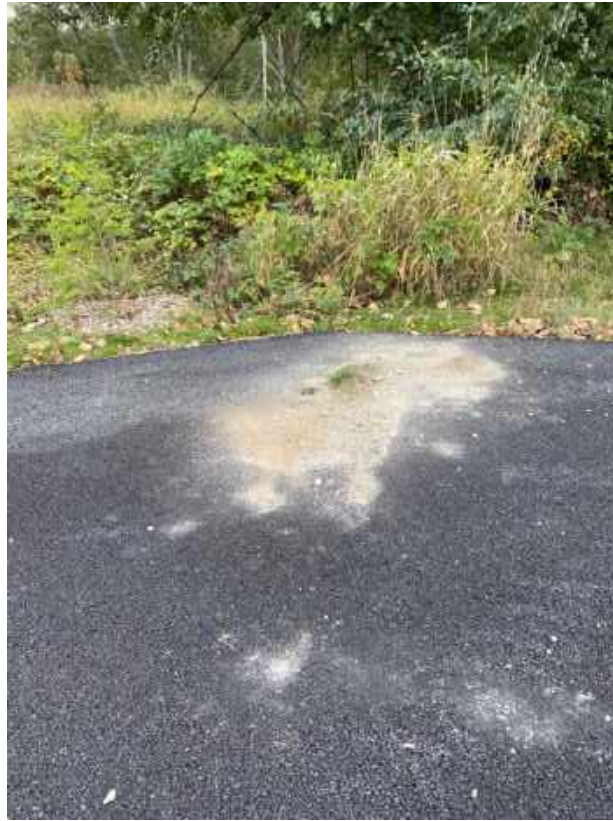
Photograph 5. This photograph was taken at the northeast corner near monitoring station DMCA 04, facing northeast. Debris piled on pavement was observed at this location.
