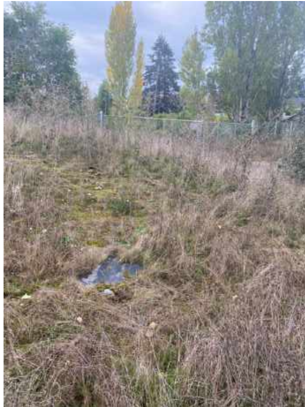
Photograph 9. This photograph was taken near the property entrance near monitoring station LLA 11, facing south. Exposed erosion lining was observed at this location.
