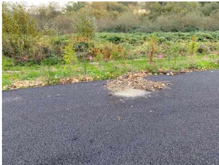
Photograph 6. This photograph was taken at the east property line near monitoring station DMCA 05, facing east. Debris piled on pavement was observed at this location.
