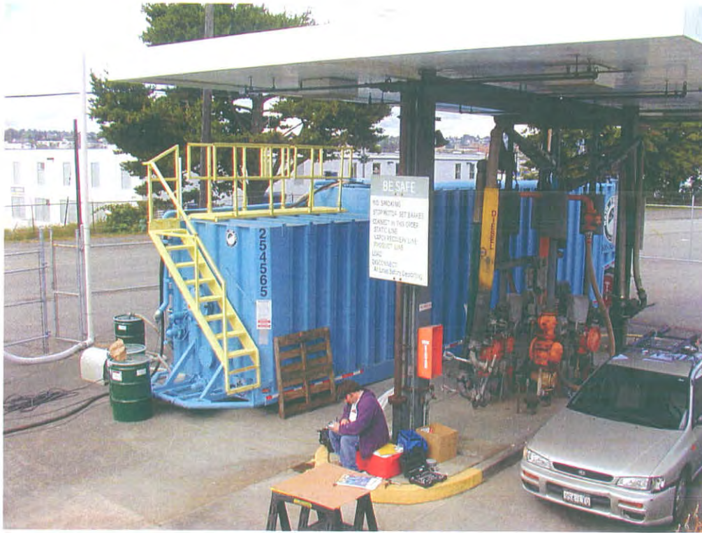
Photograph C.4 Holding Tank for Effluent Water Stream from Oil/Water Separator
