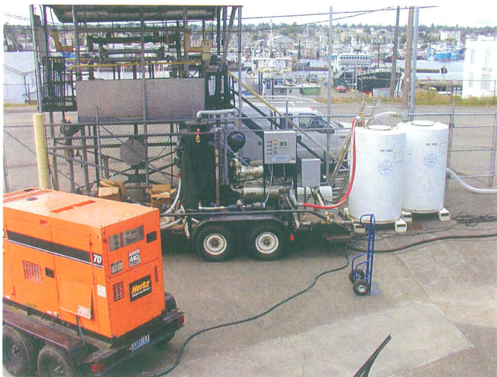
Photograph C.3 DPE Effluent Stream Treatment System – Oil/Water Separator and Activated Carbon Units
