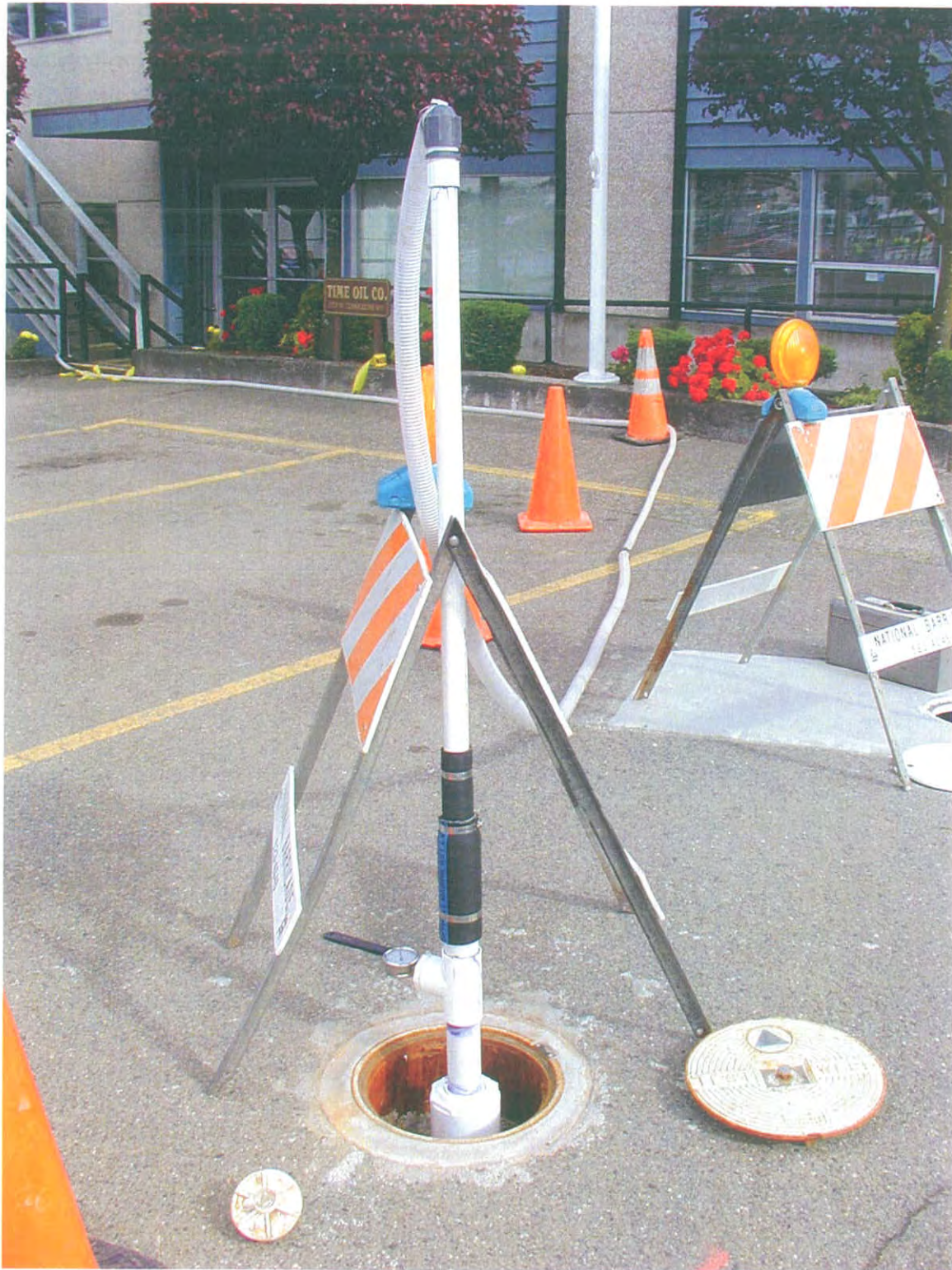
Photograph C.1 DPE Well 01MW-18 with Stinger Extraction Point Set at 20 feet below Top of Casing
