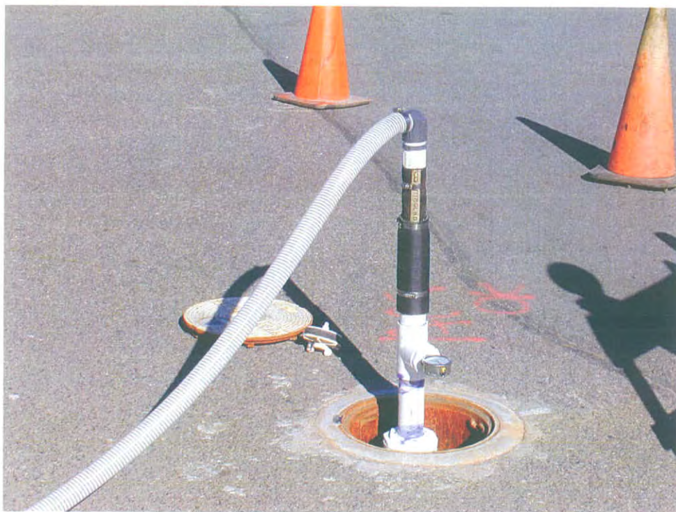
Photograph C.2 DPE Well 01MW-18 with Stinger Extraction Point Set at 23 feet below Top of Casing
