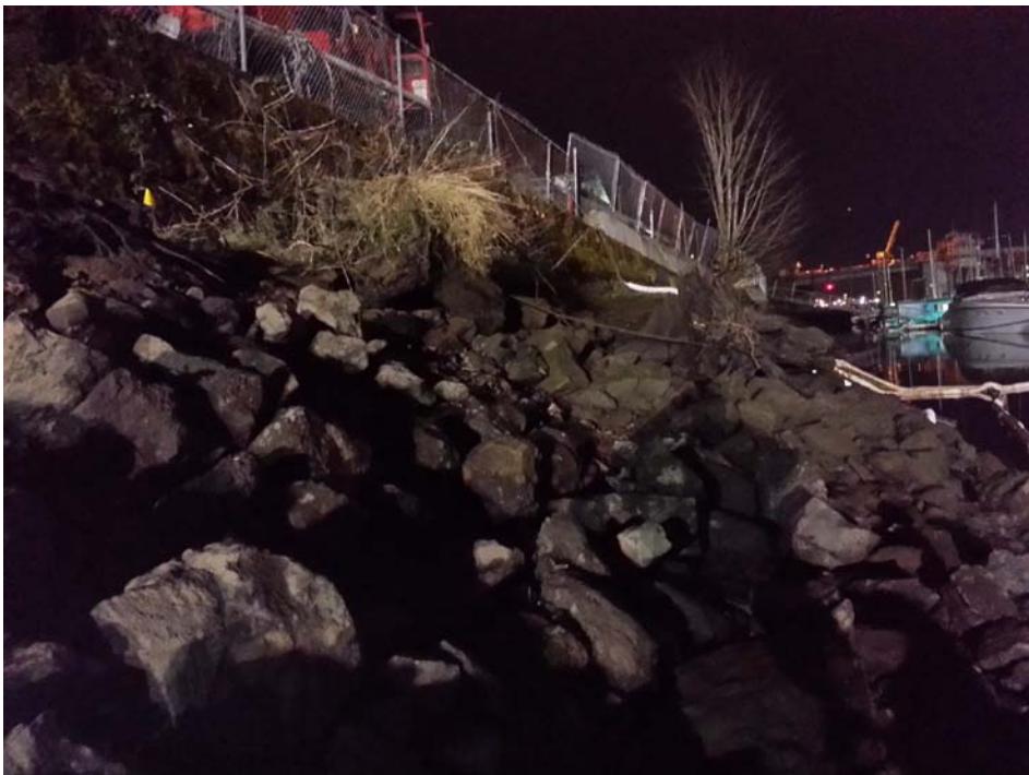
Photograph 4: Conditions of South Park Marina Bank observed during low tide. Yellow flag indicates Station 99-G (photograph taken on 2/13/14).
