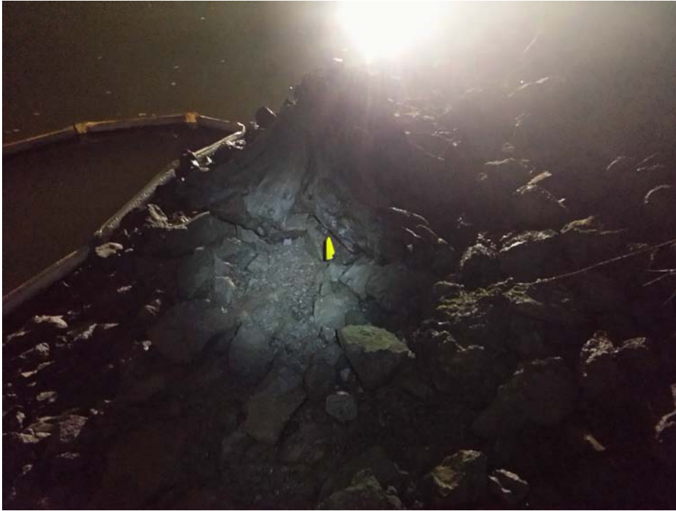
Photograph 1: Yellow flag shows Station 99-G staked by the Port surveyor (photograph taken on 2/13/14).
