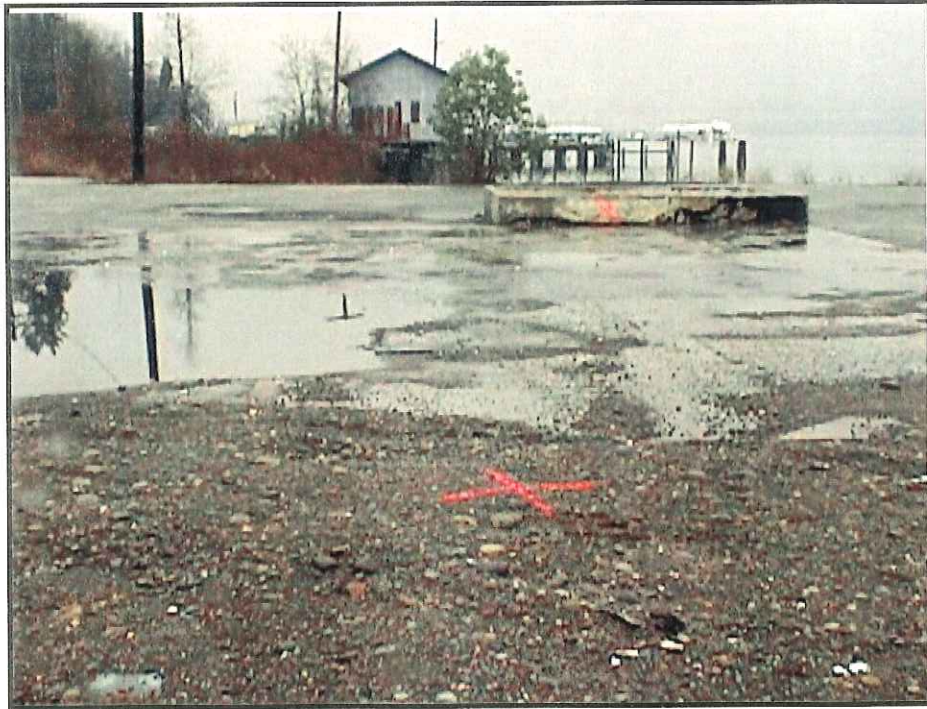
Glue speaker wastewater tank foundation and storage shed lying across northern property boundary..
