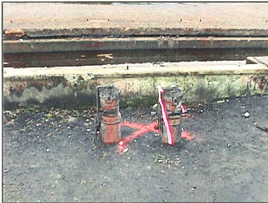
Close-up of 2 pipes, part of dryer fire deluge system (point 125) .
