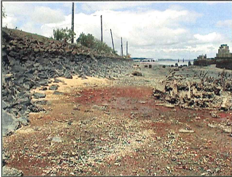
View of iron-stained sediments and former dock facing north from southern property boundary.
