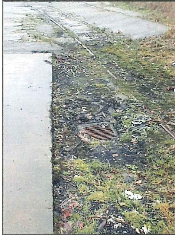
Close-up of storm sewer grate by railroad tracks, southwest corner of site.
