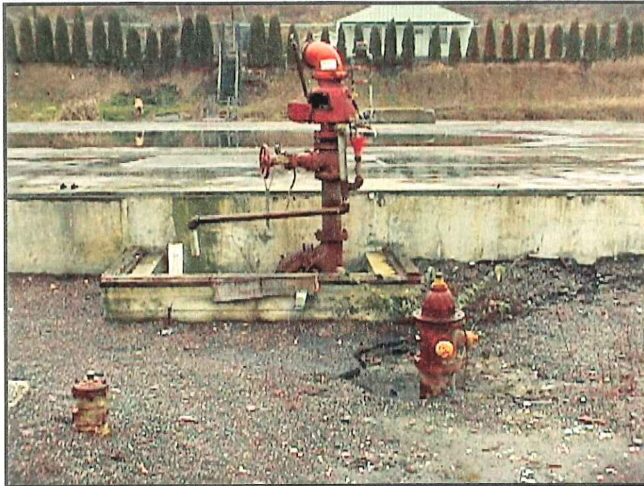
Fire system with concrete building foundation and former office in background facing west.
