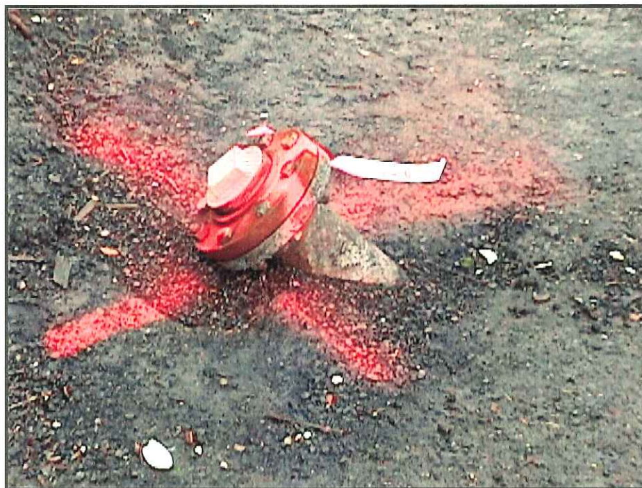
Close-up of pipe angled into ground, probable part of sanitary sewer or fire prevention system (point 126).
