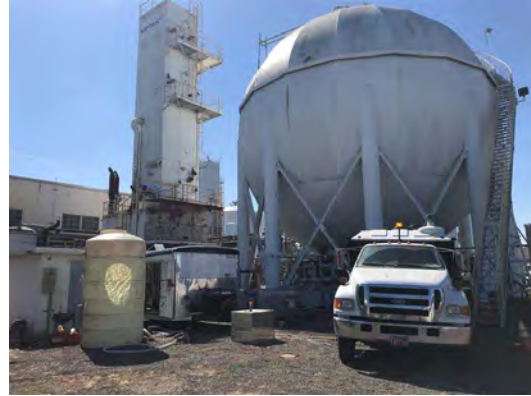
Photo 8: Injection trailer location inside Messer plant.
