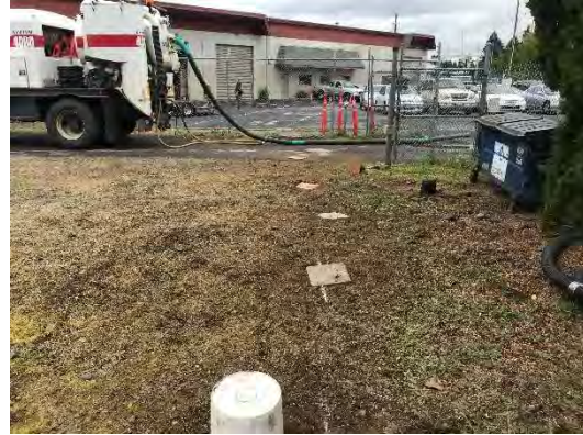
Photo 2: Row 9/Row 10 air-knife clearing.
