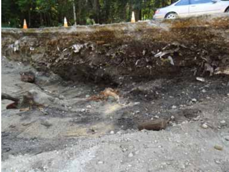
9. Fiberglass debris under Halo Kuntux lane.
