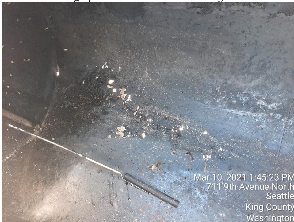
Photograph 8: Holes in the bottom of UST-A.
