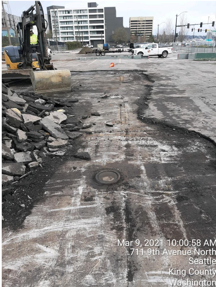
Photograph 14: Above right. Hoist-S2, Hoist-4, Hoist-S1, and Hoist-3 from the south before concrete demolition.
