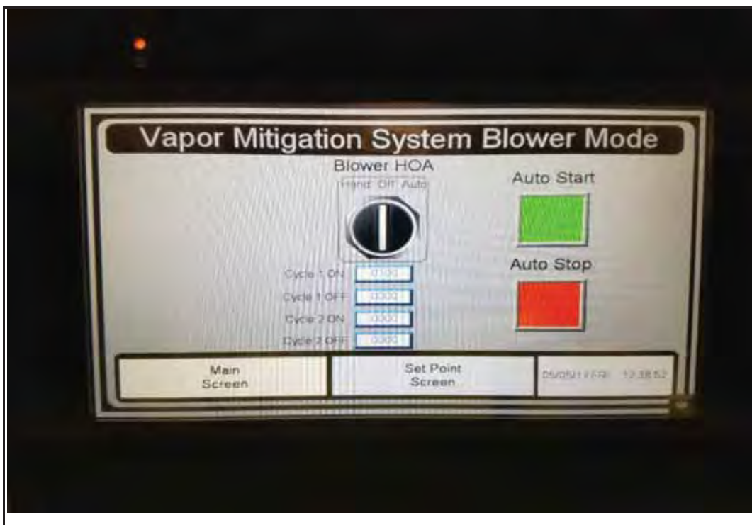
Photo 16: View of the VMS Control Panel - Blower HOA (Mode) Screen. Note the virtual HOA switch (center) and ON/OFF cycle buttons (below switch) and Auto Stop/Start buttons.
