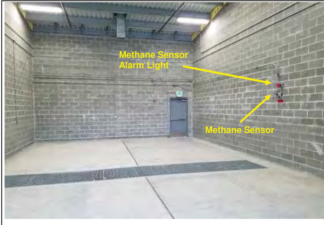
Photo 7: View of room "C" (from plans) looking to the west. Note the methane sensor and associated alarm light on the north wall (right side).
