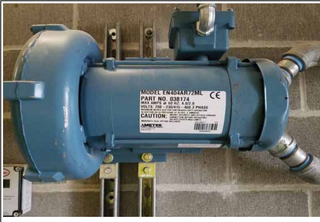
Photo 13: View of the Ametek Rotron EN404AR72ML regenerative blower that induces the vacuum and air flow from the sub-slab recover pipes.
