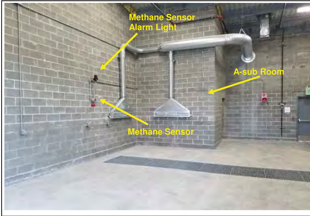
Photo 9: View of room "A" (from plans) looking to the west. Note the methane sensor and associated alarm light on the south wall (left side). Note A-sub room in corner.
