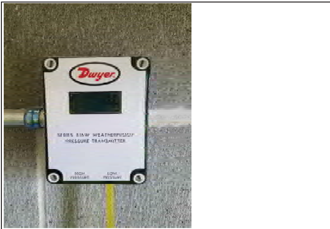
Photo 12: View of Dwyer differential pressure transmitter and screen. Transmitter reads in inches water column vacuum.
