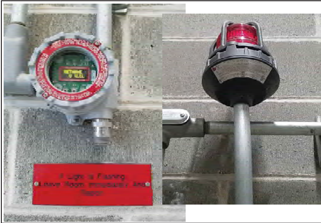
Photo 11: View of a methane sensor (left side) reading in percent (%) lower explosive limit (LEL). View of methane sensor alarm light (right side).
