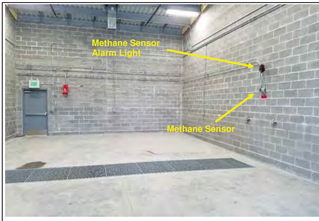
Photo 6: View of room "D" (from plans) looking to the west. Note the methane sensor and associated alarm light on the north wall (right side).
