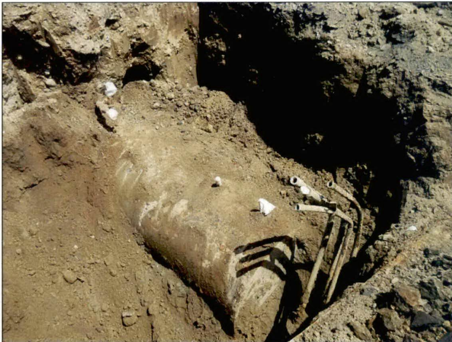
Photograph 4: One of the uncovered USTs.
