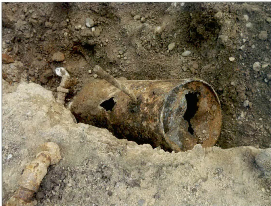
Photograph 6: The pressure vessel associated with UST2 with large holes.
