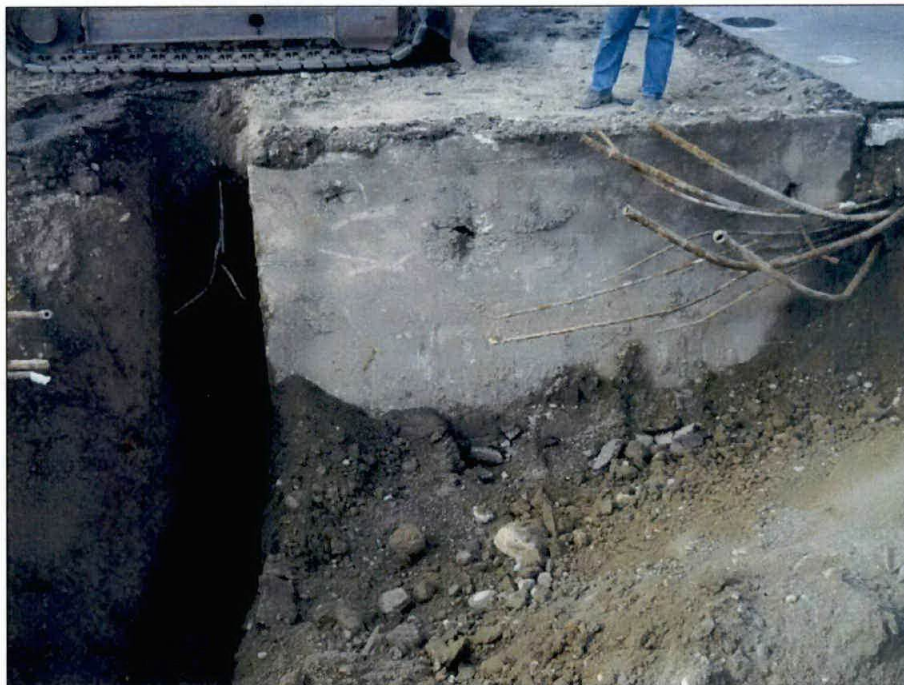
Photograph 10: Excavation around the corner of the discovered concrete vault. Piping visible includes product piping from UST to former pump islands.
