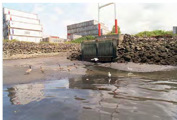
Diagonal Storm Drain Outfall at Low Tide; Grate Is Now Gone.
