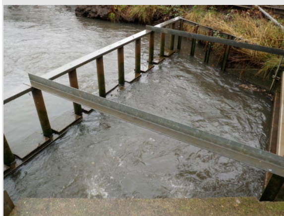
Michigan Regulator CSO Overflowing 10/26/09
