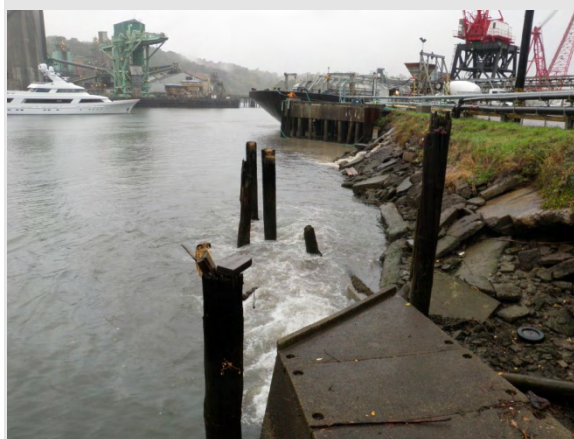
Brandon Regulator CSO Overflowing 10/17/09
