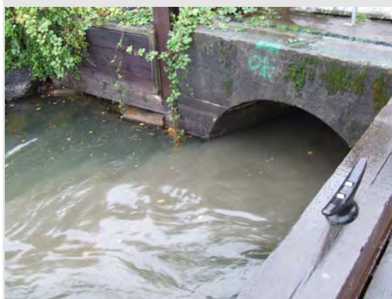
University Regulator Overflowing 10/26/09
