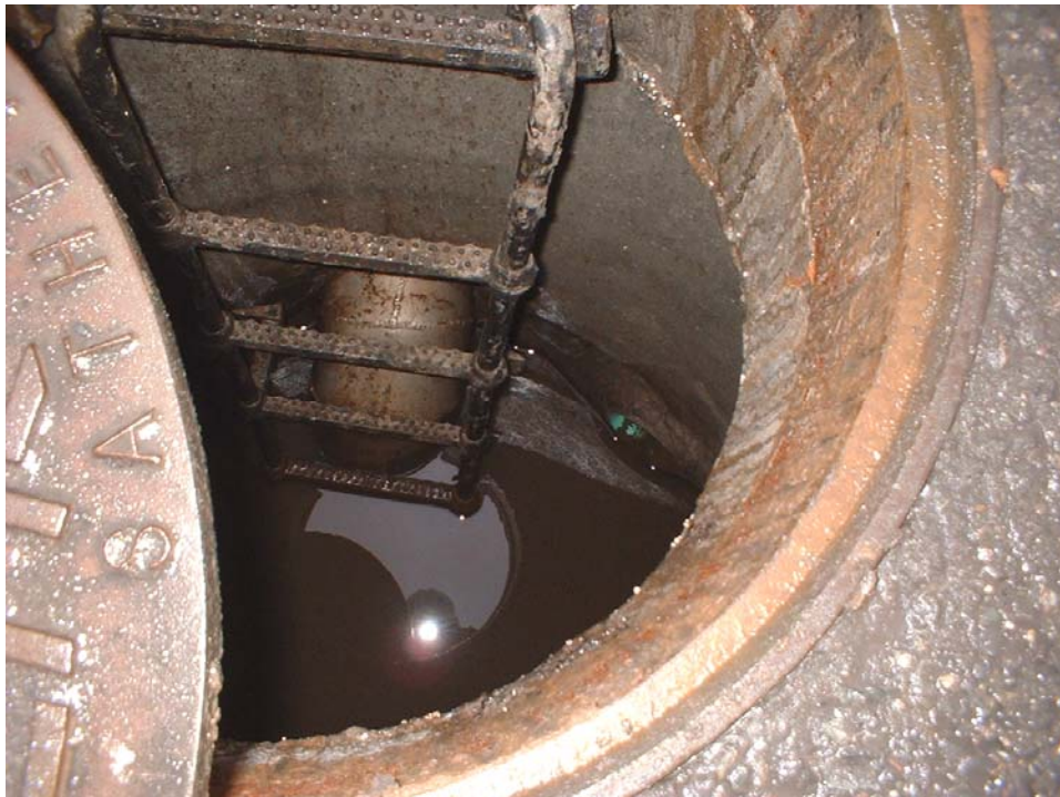
Photo 100-0031 – Looking into MH 513A showing sediment trap on south wall and pipe possibly coming in from MH 513B (to the right of sediment trap).
