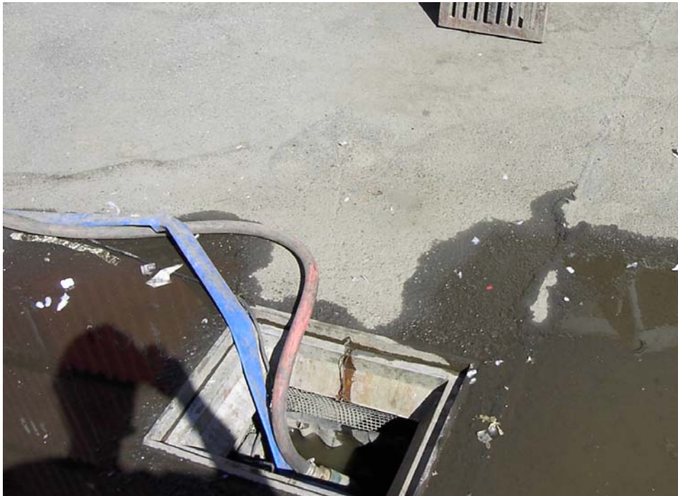
Photo 100-0838 - Shows the sump pump and filter box insert in the CB #434.
