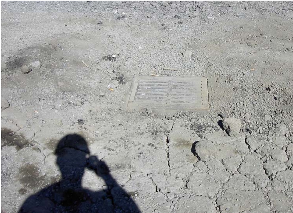
Photo 100-0840 – Looking east at CB #530. This picture also shows the condition of portions of the surfaces in the NW Container Services tenant area on the western section of the site.
