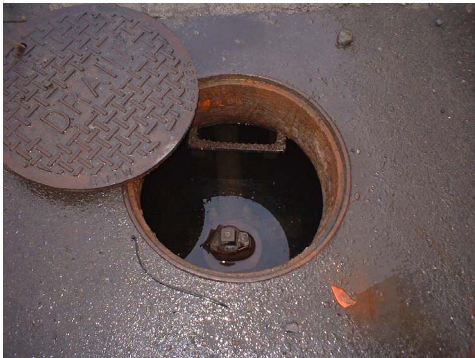
Photo 100-0033 – Looking into MH 384 showing an enclosed line with shut off valve.
