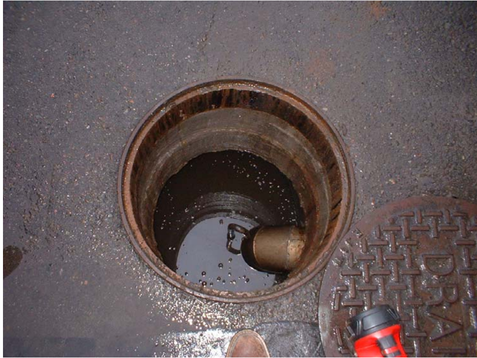
Photo 100-0034 – Looking into MH 363D, showing the sediment trap on south wall.
