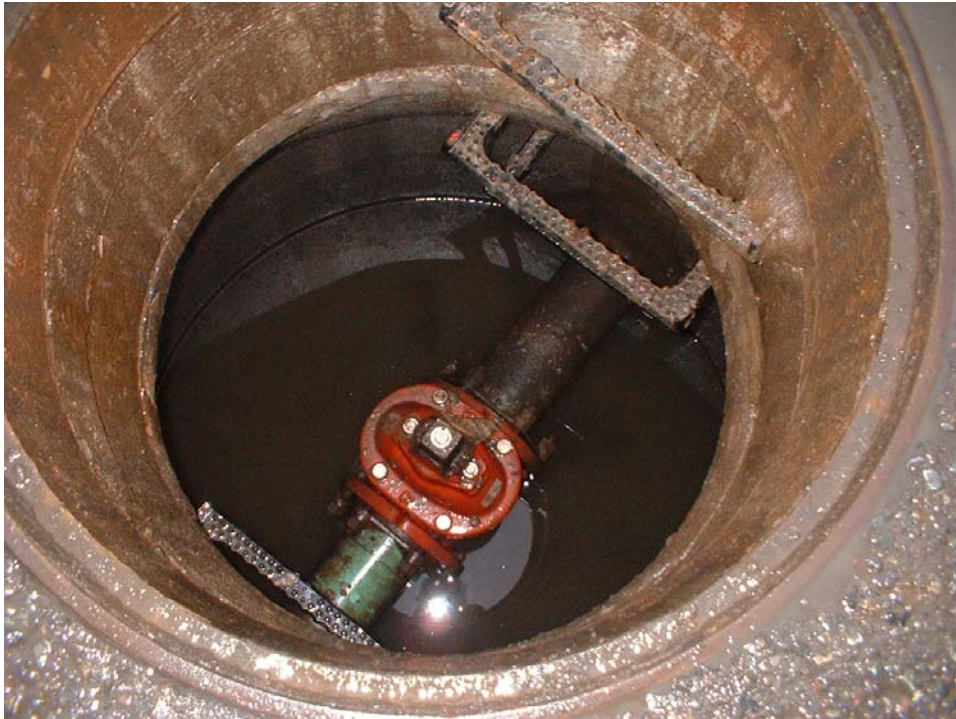
Photo 100-0027 – Looking into MH 513B showing an enclosed pipe and shut off valve.
