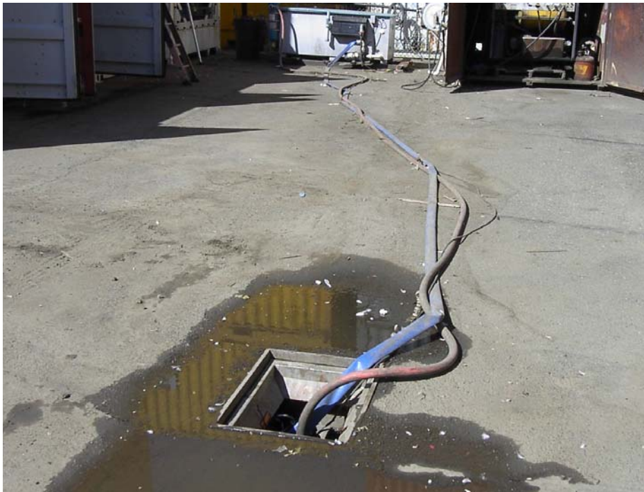
Photo 100-0839 – Looking at CB #434. Showing the sump pump and filter box insert in the CB. The pump diverts stormwater to a treatment system, shown in the background of the photo, and then back to the CB.
