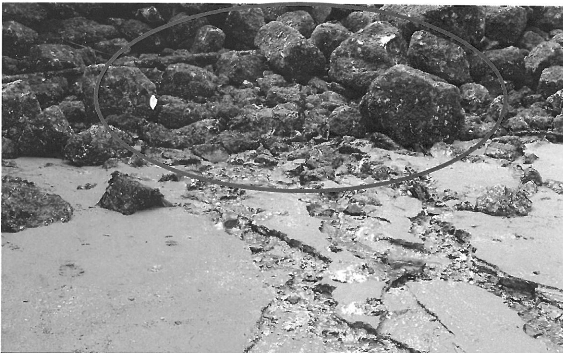
June 14, 2007 - Photo DCS-0025 Looking south at the general area of outfall # Harbor Island_Outfall_09. This outfall was evident by the water flowing from the bank and the associated structures on the surface. The size of this outfall could not be determined.
