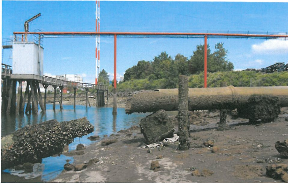
June 14, 2007 - Photo DSC-0060 Looking northeast at outfall # T108_Outfall_01.
