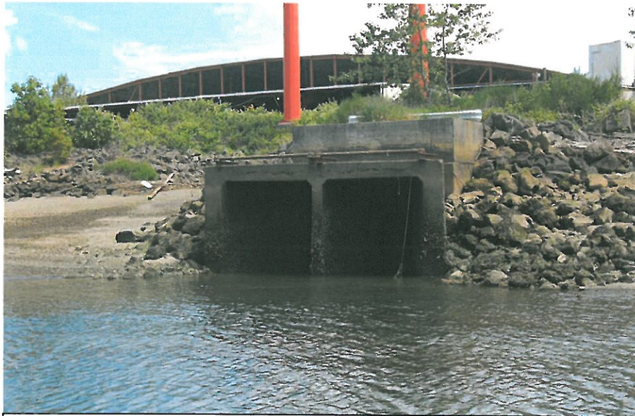
June 14, 2007 - Photo DSC-0063 Looking east at outfall # T108_Outfall_03.
