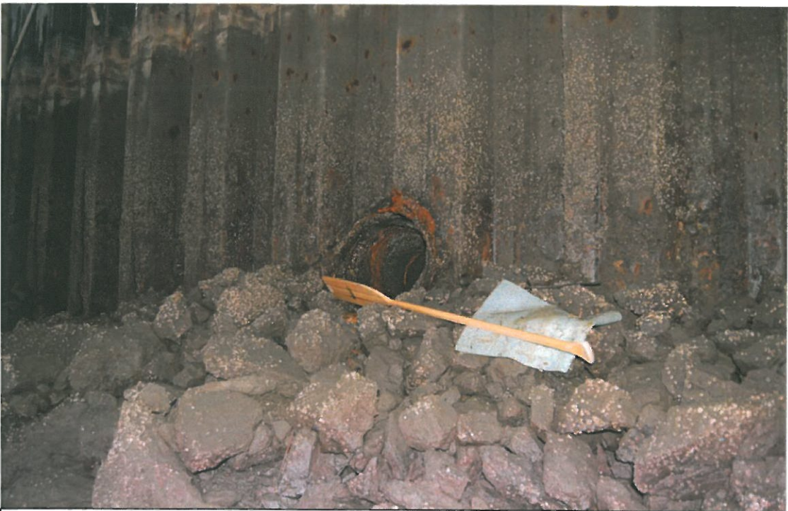
June 13, 2007 - Photo DSC-0026 Looking northeast at outfall # T30_Outfall_06.
