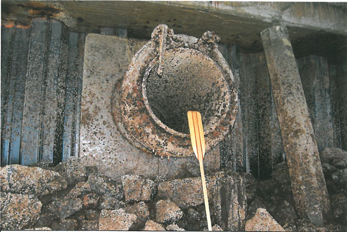
June 13, 2007 - Photo DSC-0049 Looking east at outfall # T46_Outfall_02.
