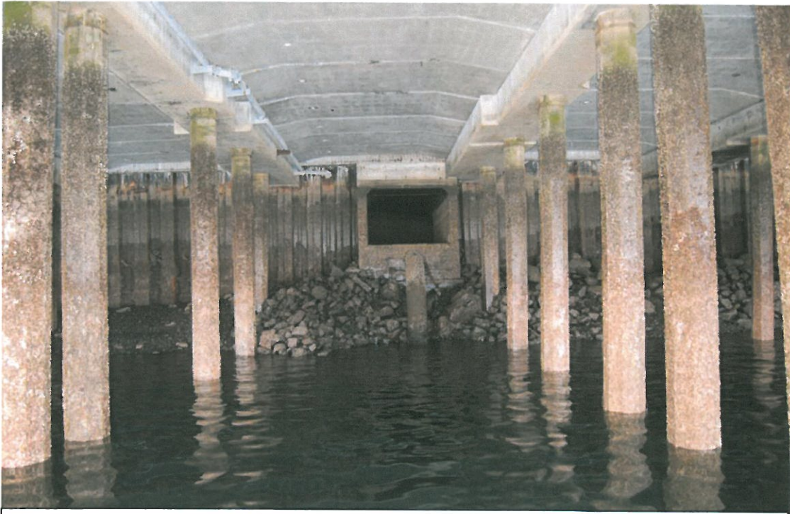
June 13, 2007 - Photo DSC-0028 Looking east at outfall # T30_Outfall_05.
