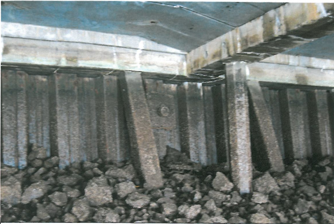
June 13, 2007 - Photo DSC-0081 Looking west at outfall # T18_Outfall_06, 3 rd of 4 sealed outfalls.
