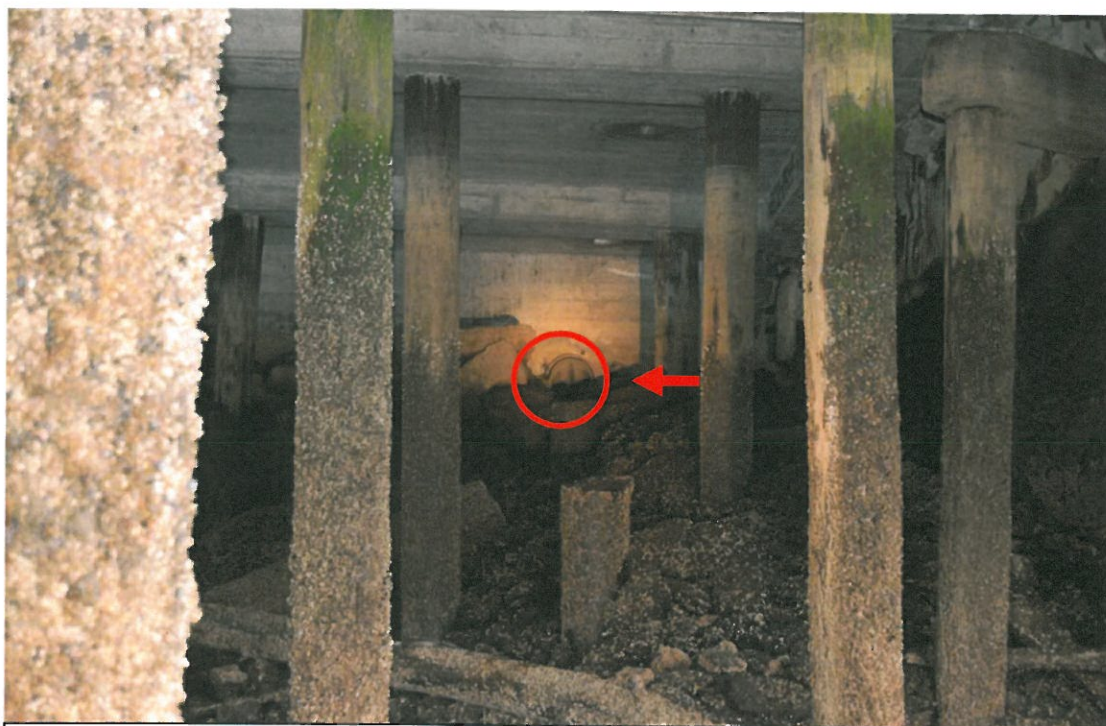
June 14, 2007 - Photo DSC-0007 Looking West at Harbor Island Outfall_02 located SE of Terminal 18.
