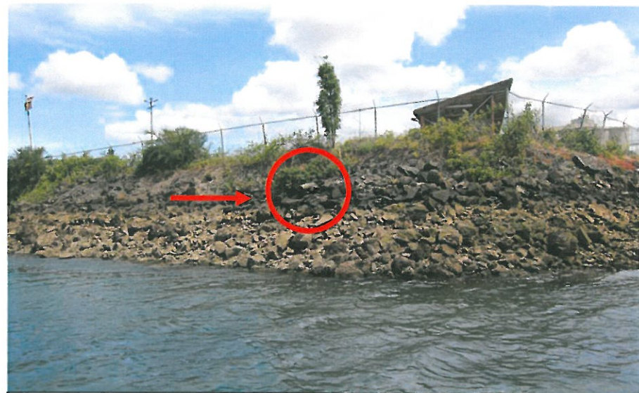
June 13, 2007 - Photo DSC-0105 Looking east at outfall # T104_Outfall_02.
