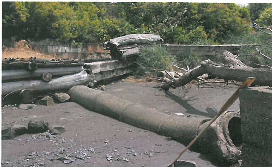
June 14, 2007 - Photo DSC-0058 Looking east at outfall # T108_Outfall_02.
