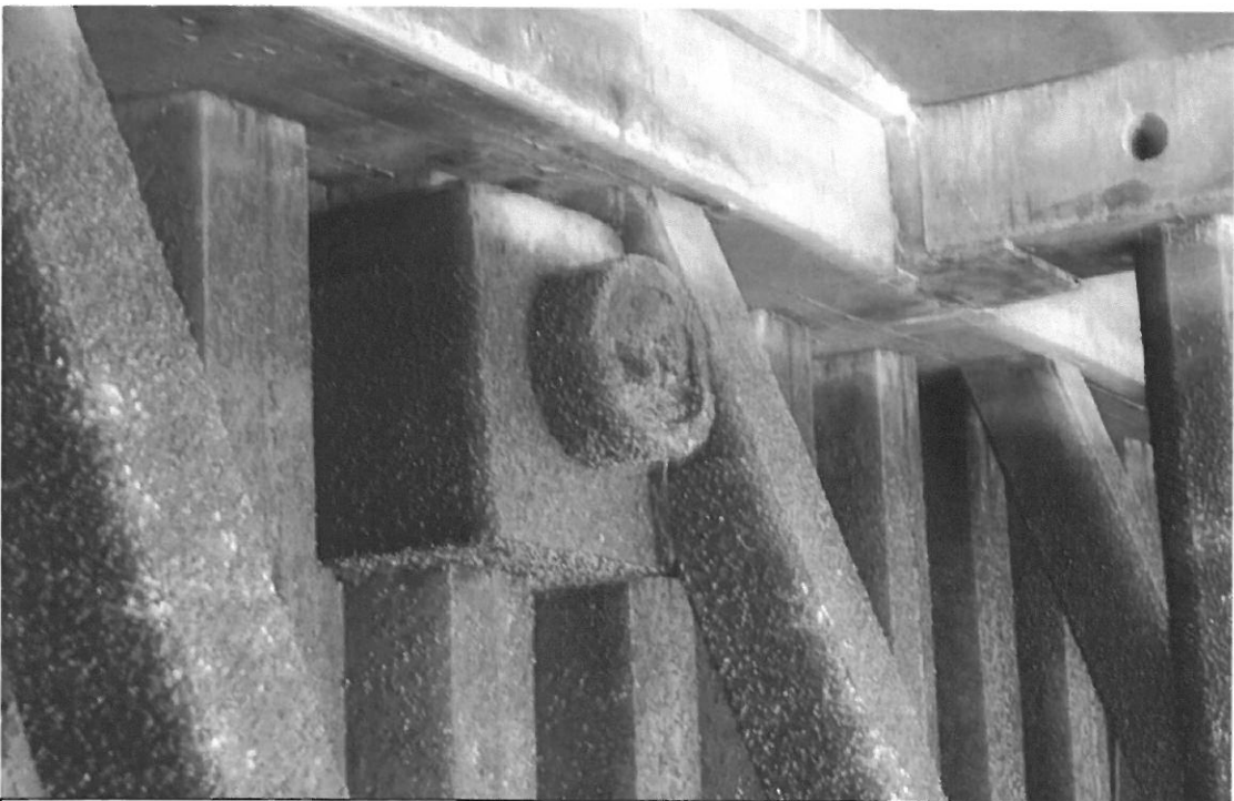
June 13, 2007 - Photo DSC-0076 Looking northwest at outfall # T18_Outfall_03, 1st of 4 sealed outfalls.
