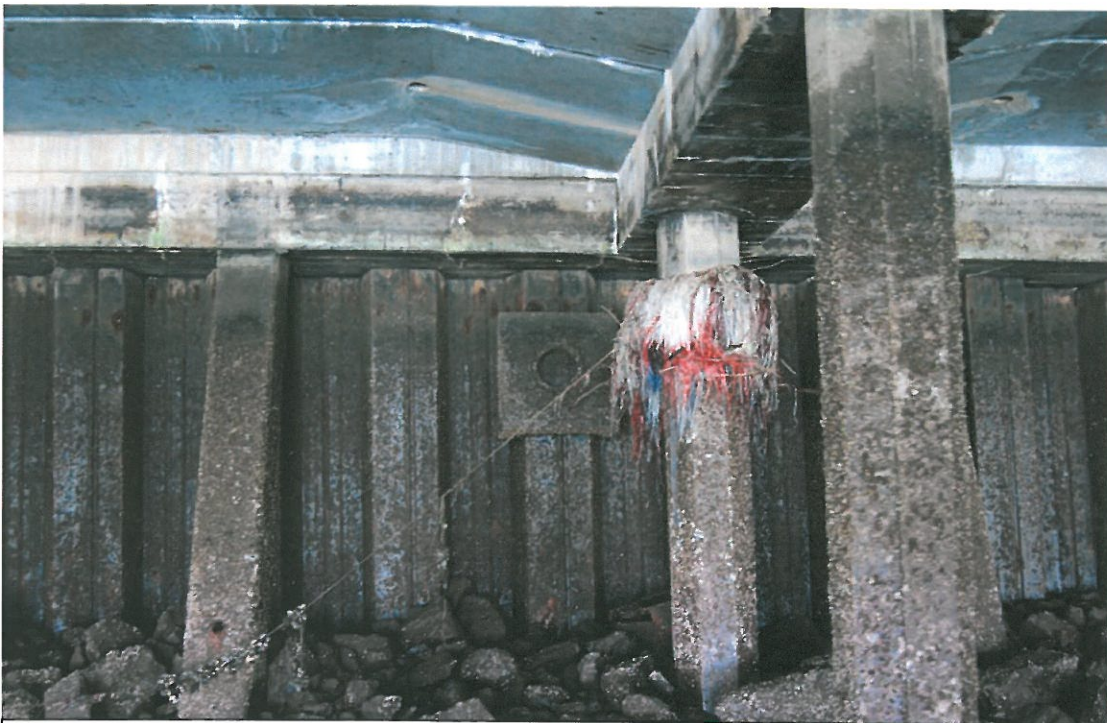
June 13, 2007 - Photo DSC-0082 Looking west at outfall # T18_Outfall_07, 4 th of 4 sealed outfalls.
