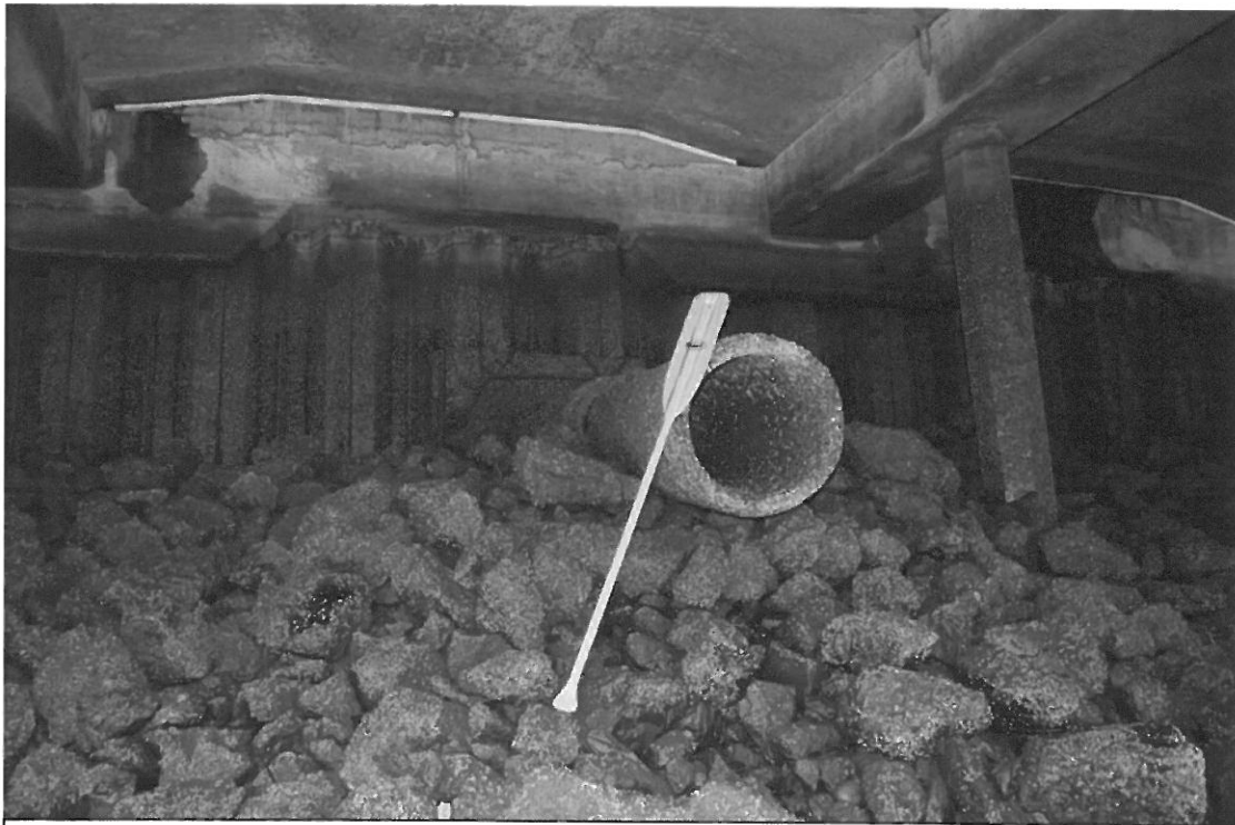
June 13, 2007 - Photo DSC-0032 Looking east at outfall # T30_Outfall_04.
