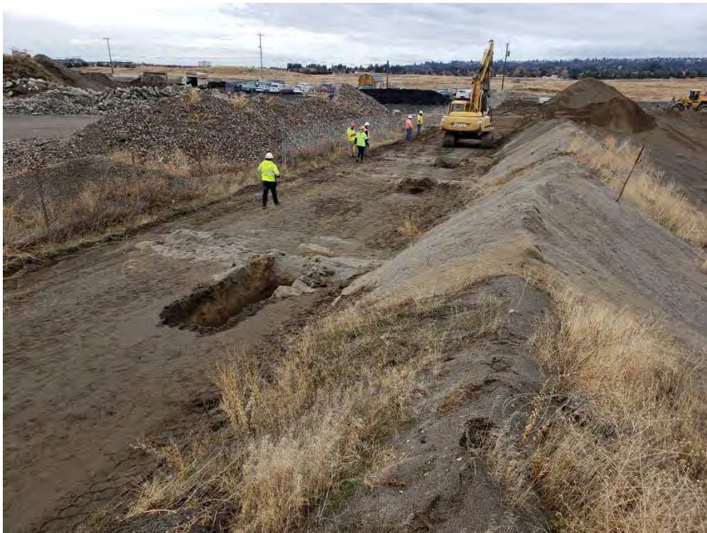
Photo shows test pits dug along the pipeline along the southern property boundary. Photo was taken looking in a southwesterly direction.
