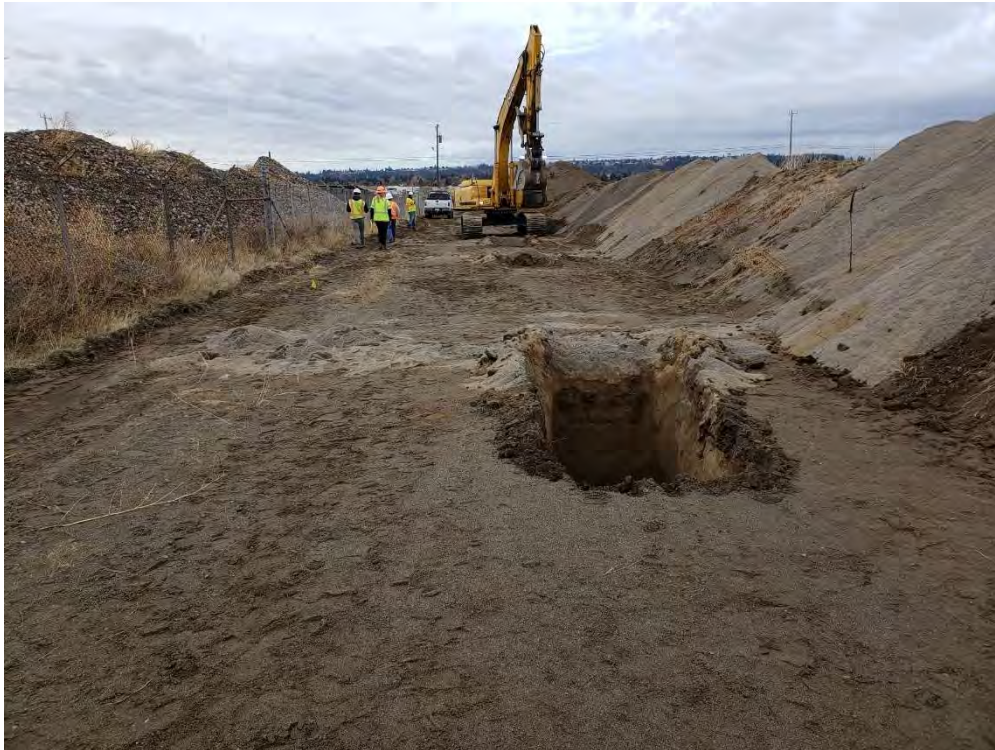
Photo shows test pits being dug along the pipeline along the southern property boundary. Yellow flags mark the pipeline. Photo was taken looking in a westerly direction.
