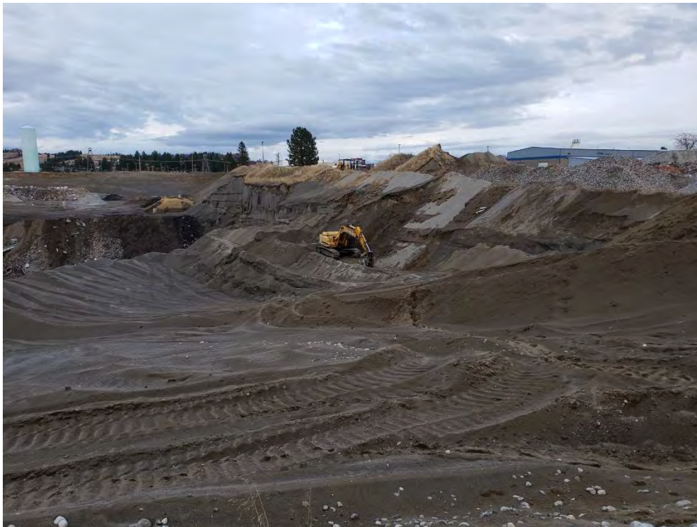
Photo shows location of bench where contamination was discovered (where excavator is located). Photo was taken looking in a southeasterly direction.
