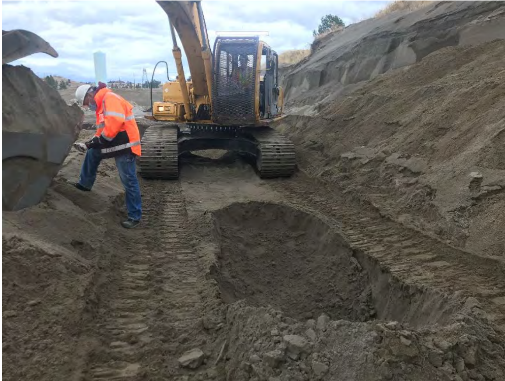
Photo shows ACT personnel investigating soils from a test pit dug into the bench where contamination was discovered. Photo was taken looking in an easterly direction.
