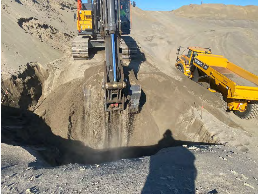
Photo shows contaminated soil being removed. Photo was taken looking in a westerly direction.
