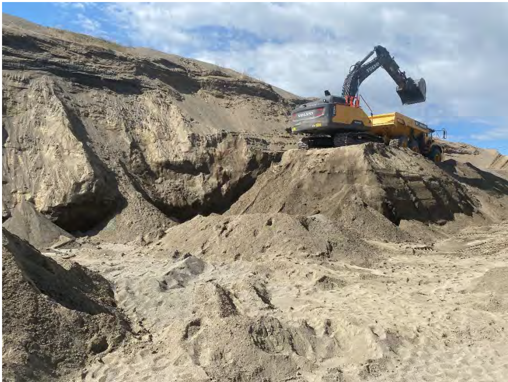
Photo shows contaminated soil from the bench being removed. Photo was taken looking in a southwesterly direction.
