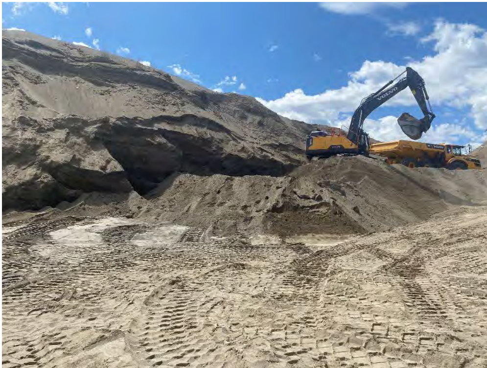
Photo shows contaminated soil being removed. Contamination here did not go as deep thus excavation was benched up higher. Photo was taken looking in a southwesterly direction.
