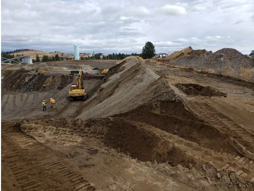
Photo shows pipeline associated test pits in relation to bench where contamination was discovered (where excavator is located). Photo was taken looking in an easterly direction.
