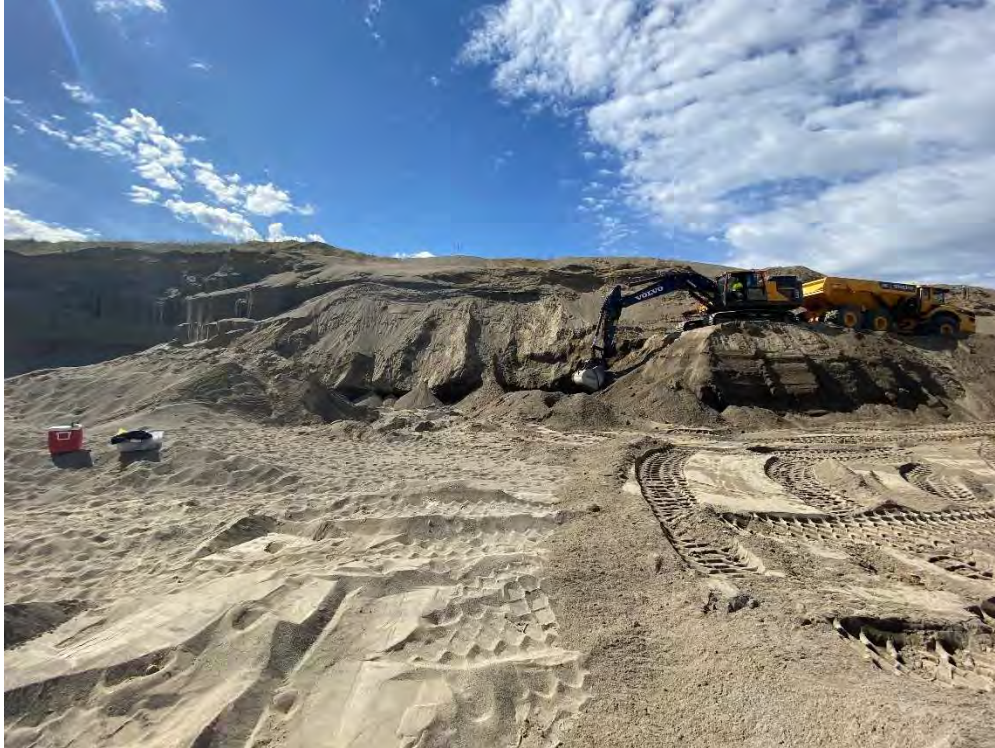
Photo shows contaminated soil being removed. Most of the bench was being removed up to this point. Photo was taken looking in a southerly direction.
