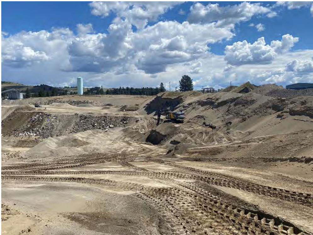
Photo shows contaminated soil being removed. Photo was taken looking in a southeasterly direction.
