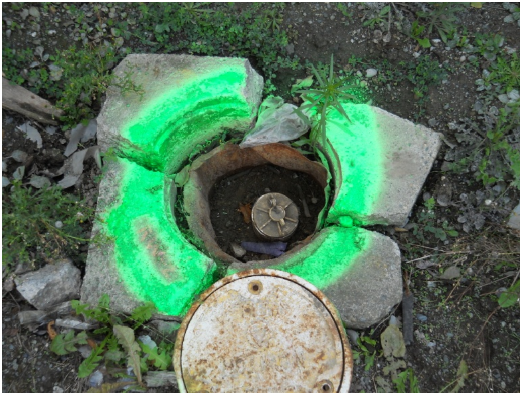
Photograph 1. Condition of well RW-2 prior to repair.
