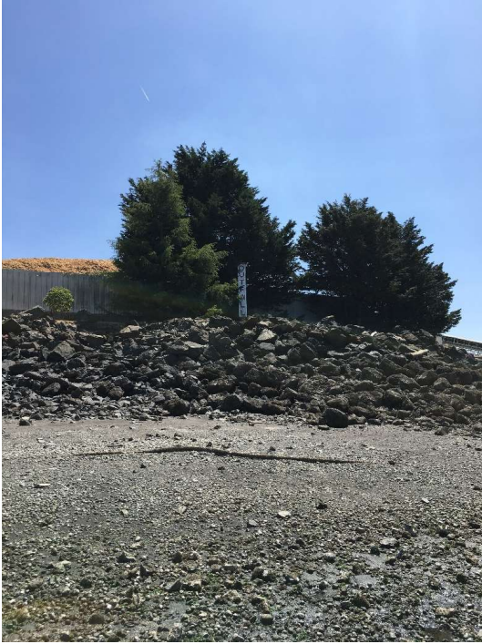
Photo 15: Looking South, bank location of buried NPDES outfall pipe is marked with vertical white sign.
