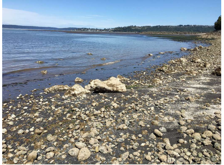
Photo 10: Western end of cap looking East toward far Jetty, peninsula, and Puyallup River. Scattered larger rocks noted, and more frequent patchy areas of finer-grained material observed in foreground.
