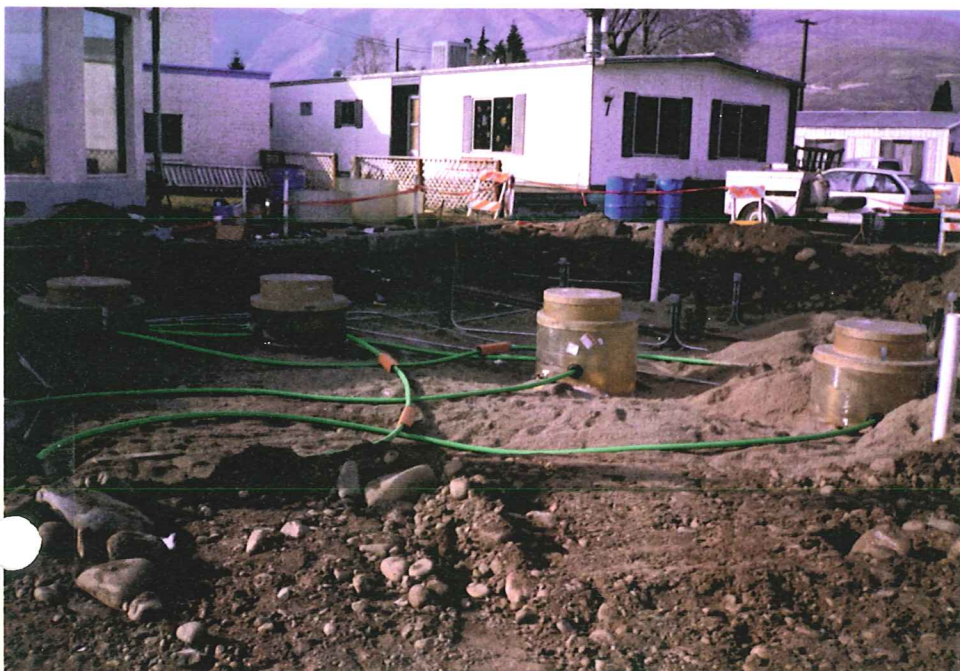
Site Photograph 6 - Construction phase of new station showing product sumps, FLEX II HDPE product line and collector sump.
