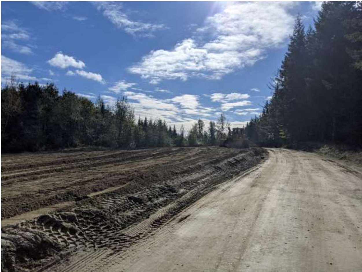
Photograph 3 – View of general fill soil placed over geomembrane and geocomposite at Areas 7/8.
