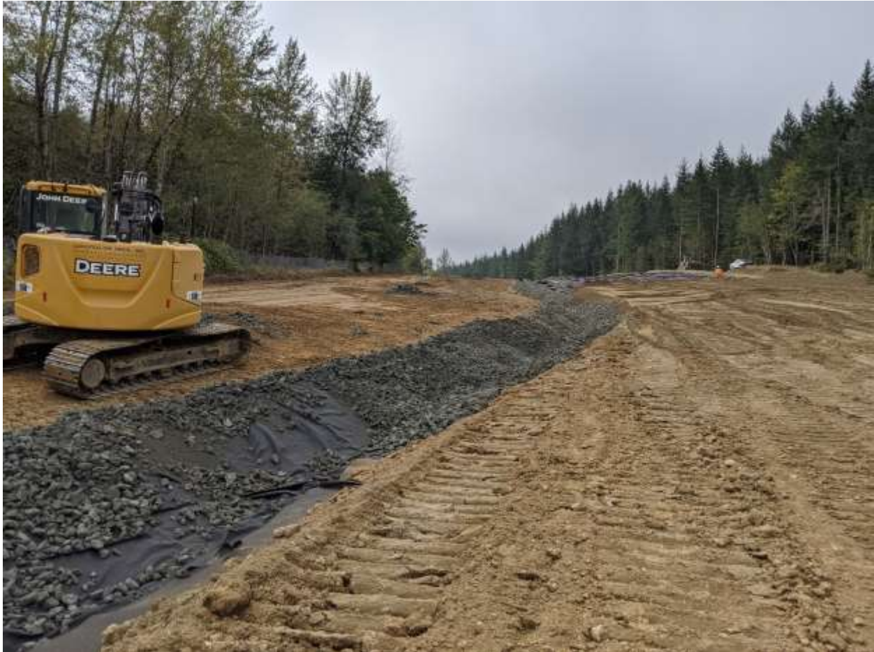
Photograph 4 – View of rock-lined ditch being installed at east side of Area 7/8. This ditch ties into the rock-lined ditch west of Area 9.
