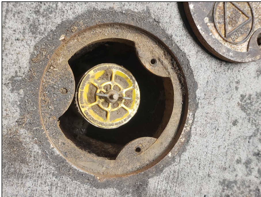
Photograph 6: View of RW1 well casing.
