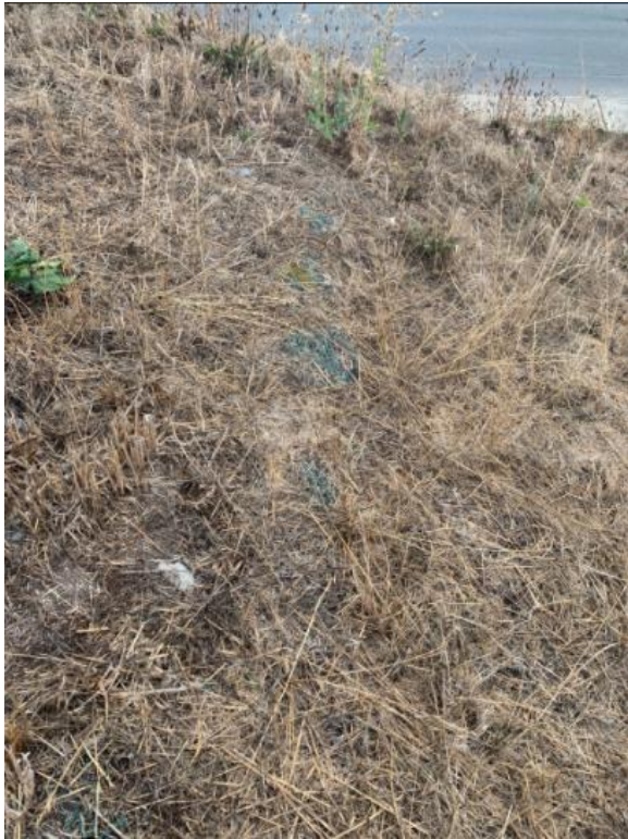
Location 35. Exposed Geotextile
