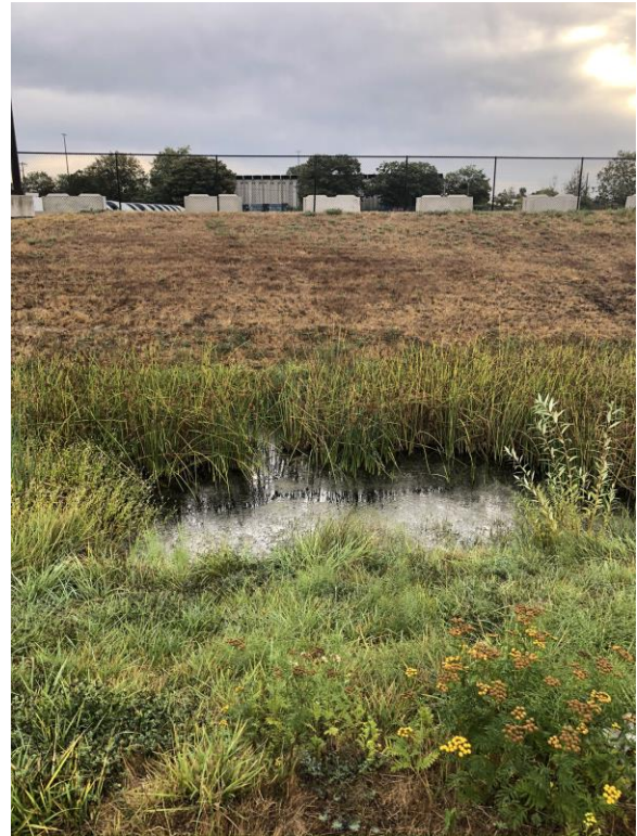
Location 1. Standing Water in West Bioswale
