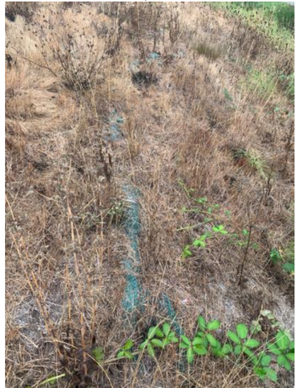
Location 38. Exposed Geotextile
