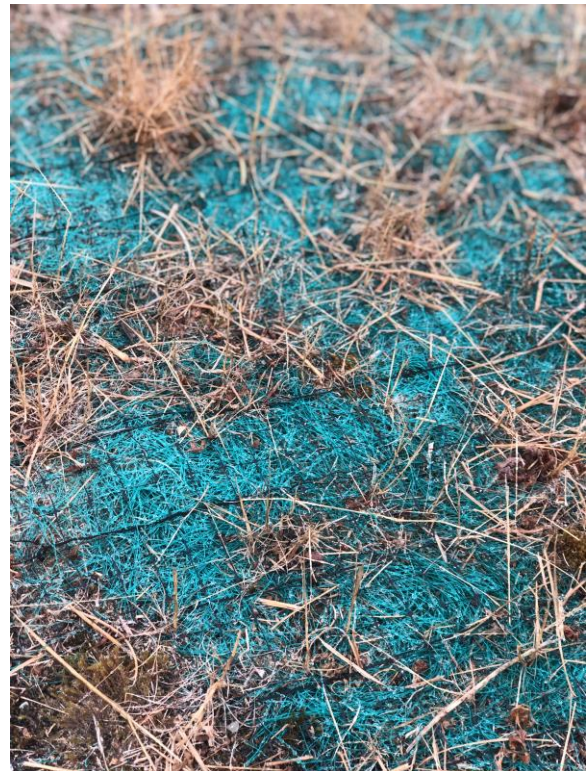
Location 2. Exposed Geotextile
