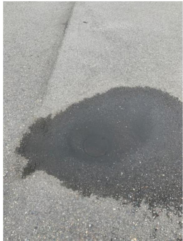
Location 22. Ponding above Sanitary Cleanout
