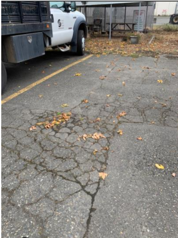
Location 27. Minor Pavement Cracking
