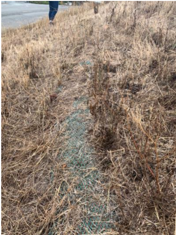
Location 37. Exposed Geotextile
