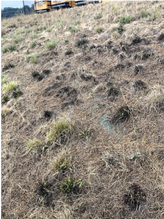
Location 12. Exposed Geotextile
