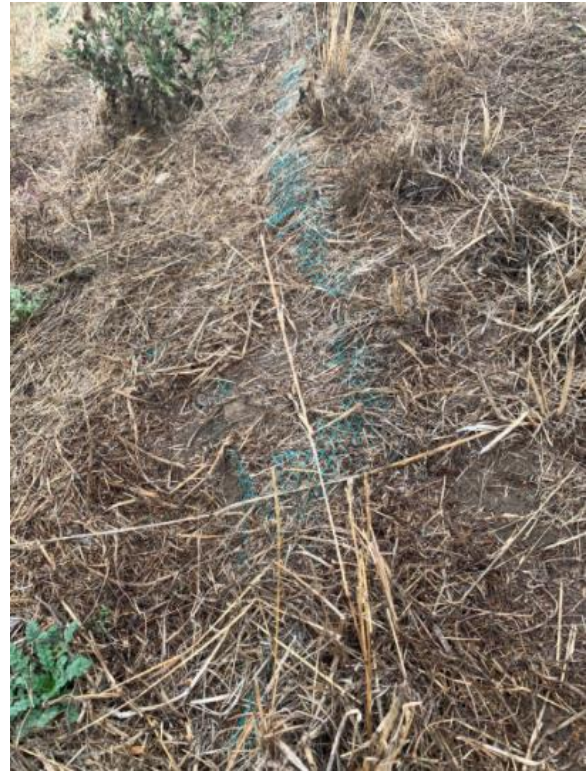
Location 36. Exposed Geotextile
