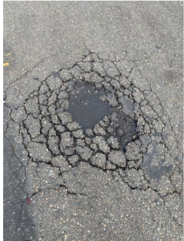
Location 32. Minor Pavement Cracking
