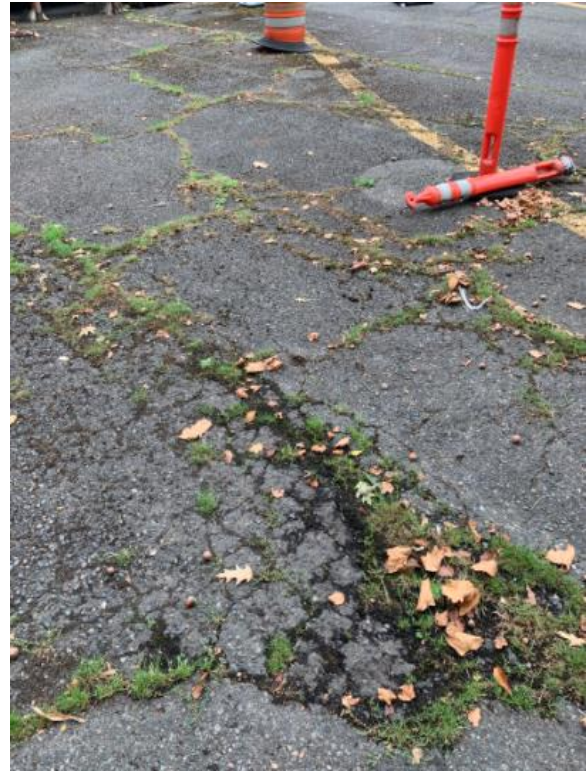
Location 28. Minor Pavement Cracking
