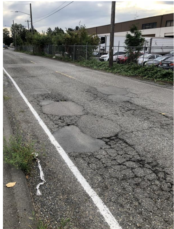
Location 8. Potholes/Pavement Cracking
