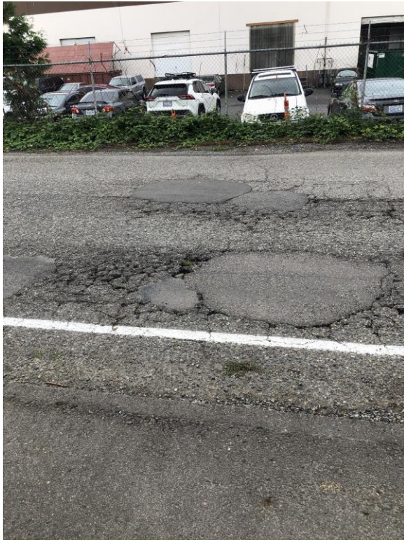
Location 8. Potholes/Pavement Cracking
