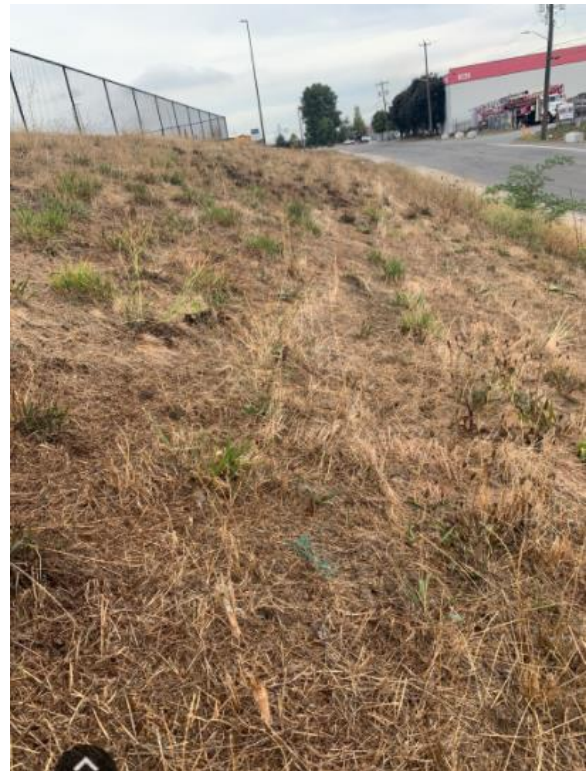
Location 34. Exposed Geotextile
