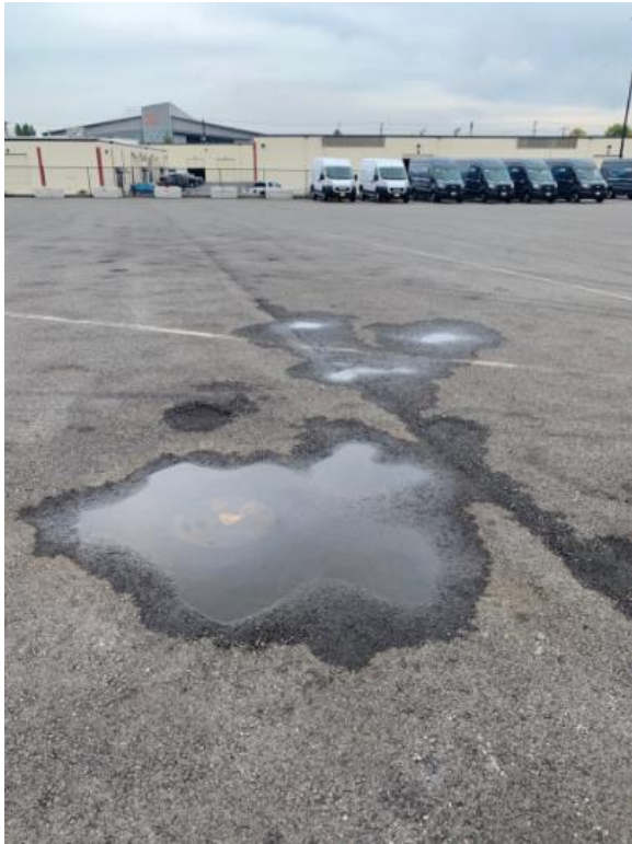
Location 16. Ponding above LFG Collector Control Box V4
