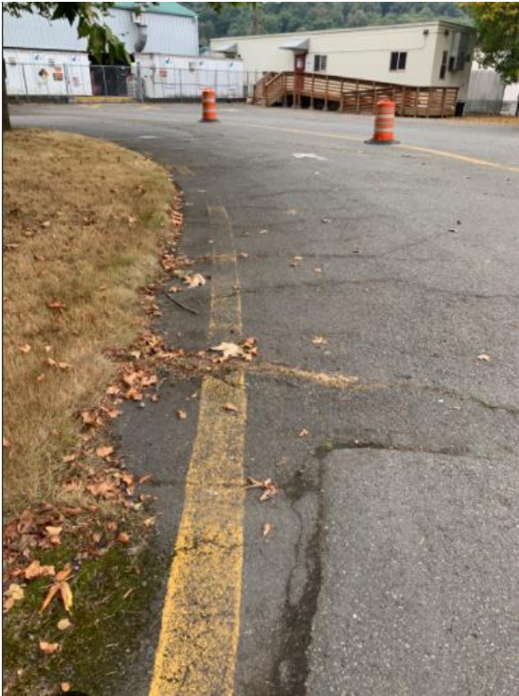
Location 39. Minor Pavement Cracking
