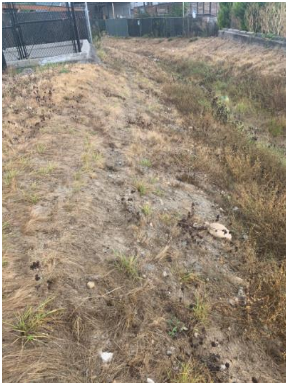
Location 33. Exposed Geotextile
