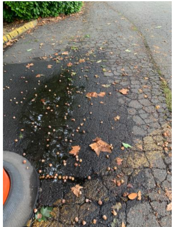
Location 26. Minor Pavement Cracking/Ponding
