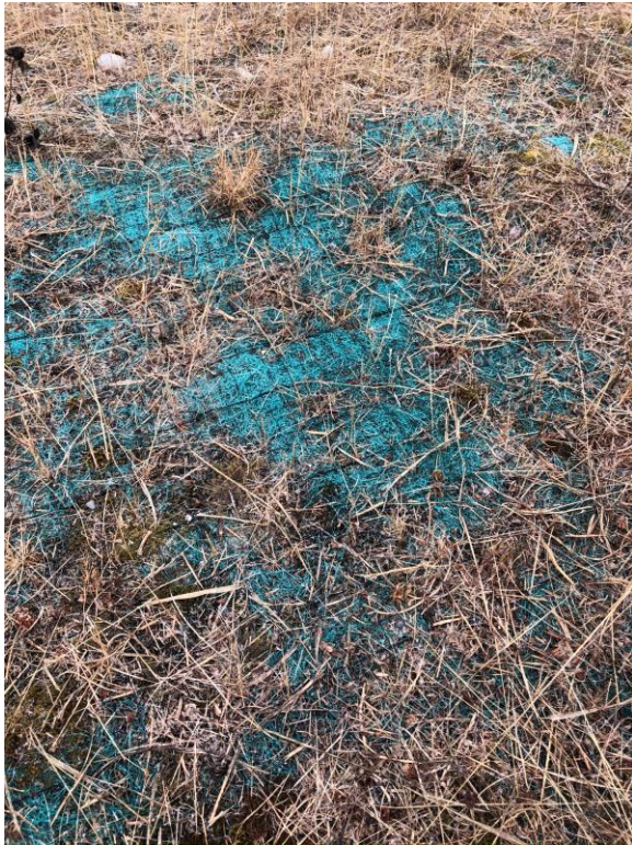
Location 2. Exposed Geotextile
