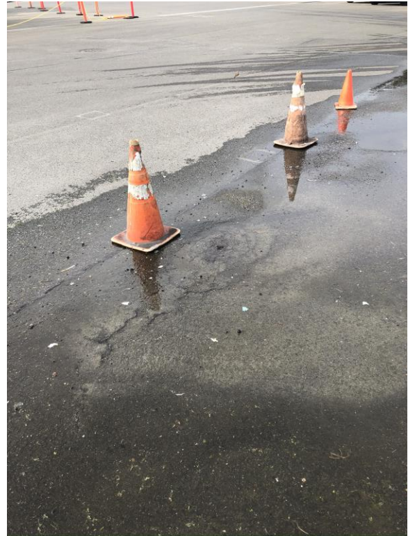
Location 20. Water Flowing from Asphalt
