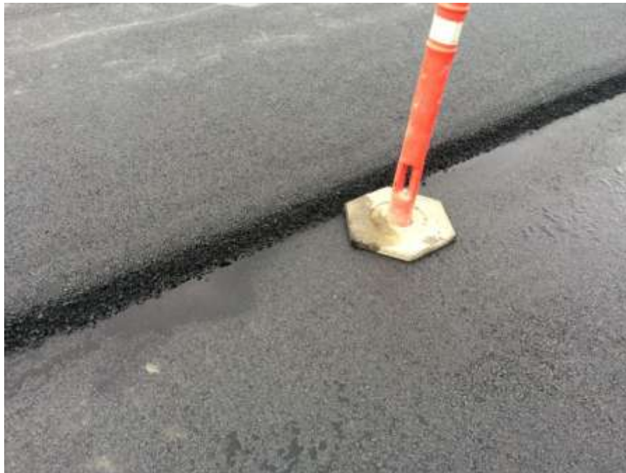
Photo 18: Asphaltic concrete pavement cover cap first 2-inch lift and second 2-inch lift
