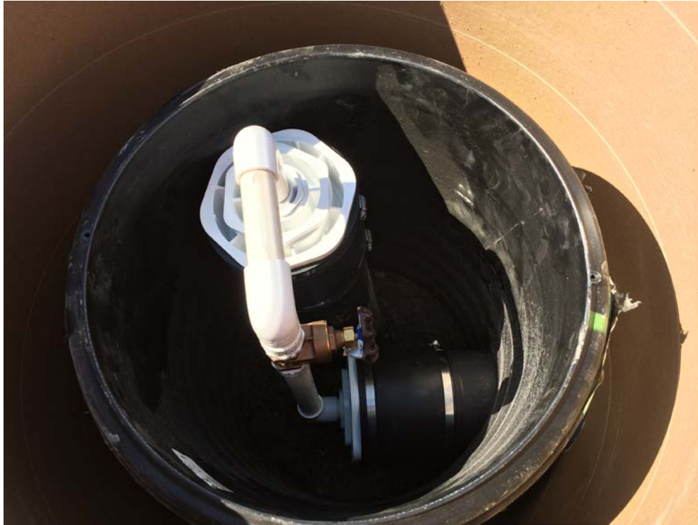
Photograph 33: Gas collection well head assembly.
