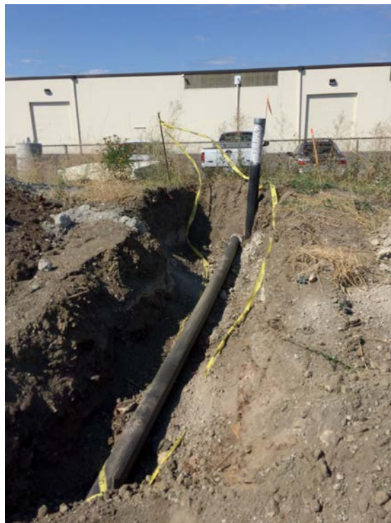
Photograph 28: Landfill gas collection well and connector piping prior to backfill placement, looking north.
