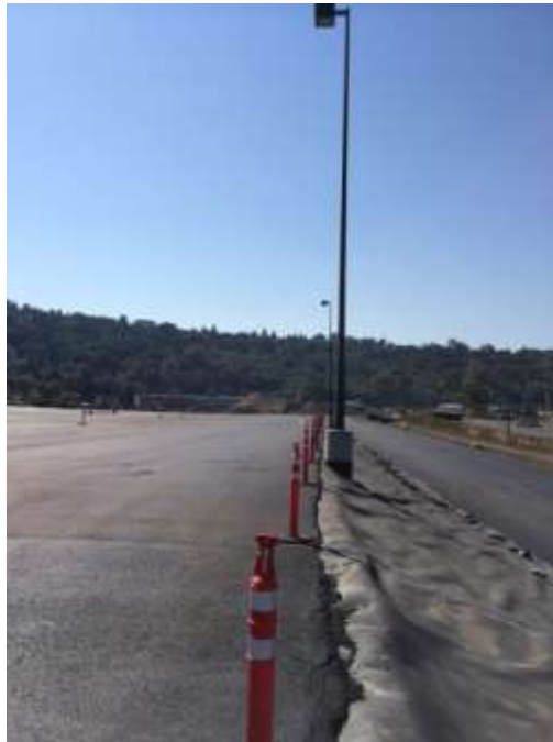
Photo 17: Asphaltic concrete pavement cover cap and low-permeability liner on north slope above north access road
