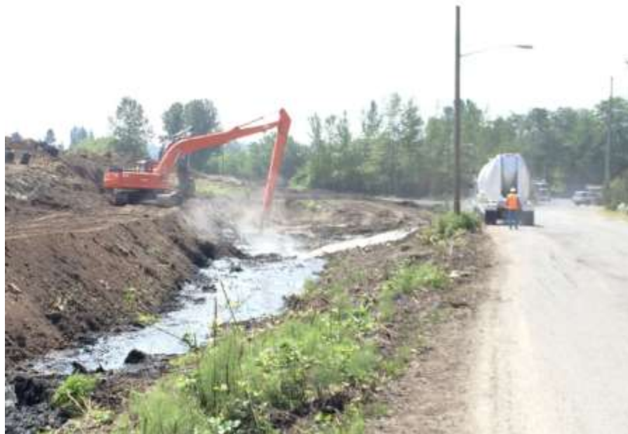
Photo 2: West Ditch soil solidification at south end
