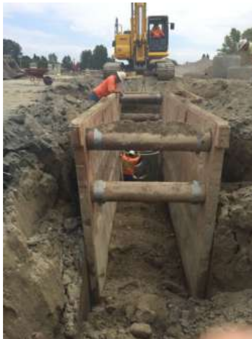
Photo 4: Storm water pipe trench through approximately 8 feet of new backfill atop landfill
