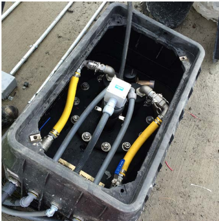
Photograph 4: North sump surface structure and discharge piping.
