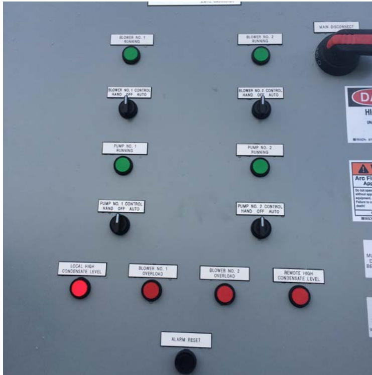
Photograph 5: North treatment compound control panel.
