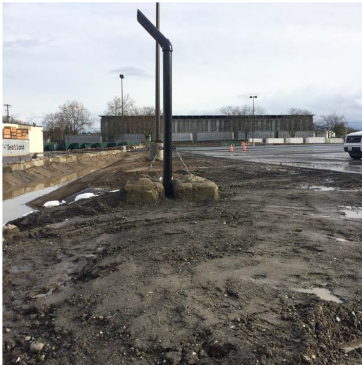
Photograph 2: Landfill gas vent stack at north treatment compound.
