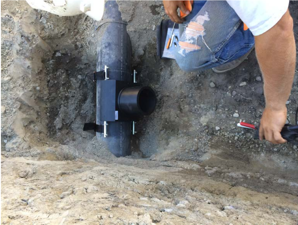
Photograph 29: Gas connector tee for lateral connection.
