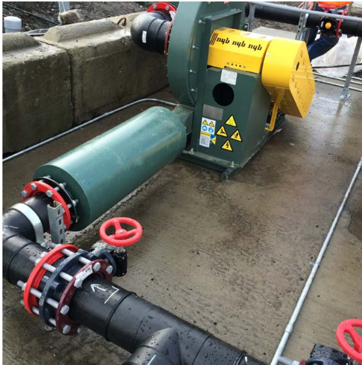
Photograph 3: Landfill gas blower, silencer, and discharge piping.
