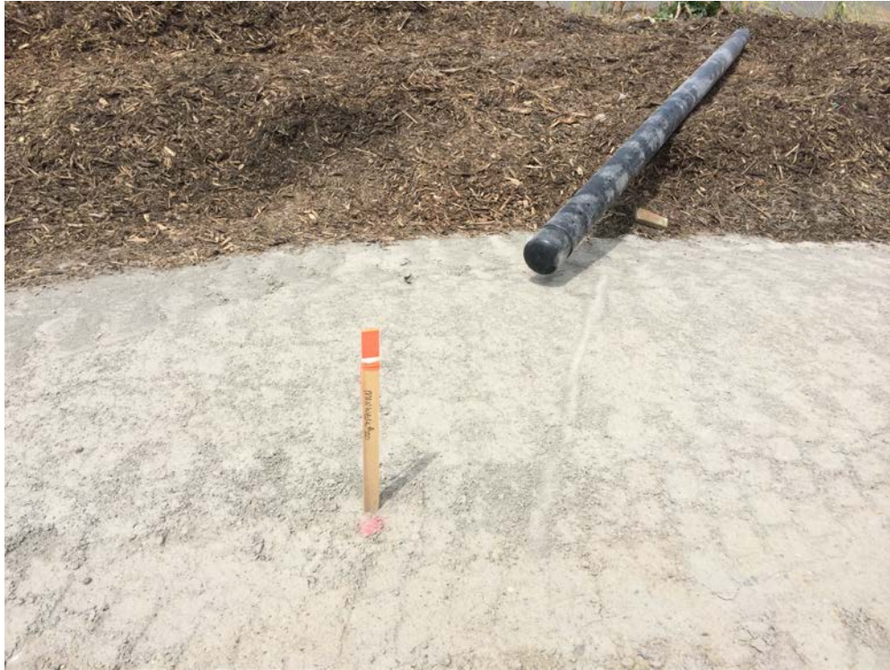
Photograph 9: Gas collection well No. 20 location and associated well materials, looking north.
