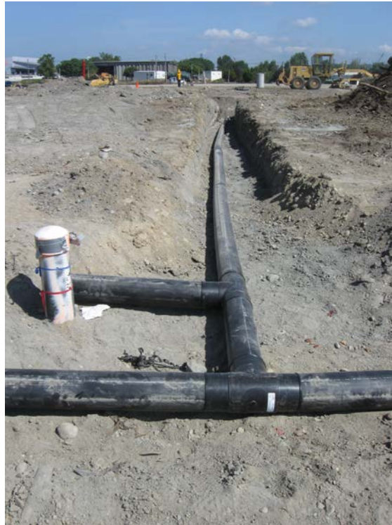
Photograph 27: Landfill gas collection well and connector piping prior to backfill placement, looking north.
