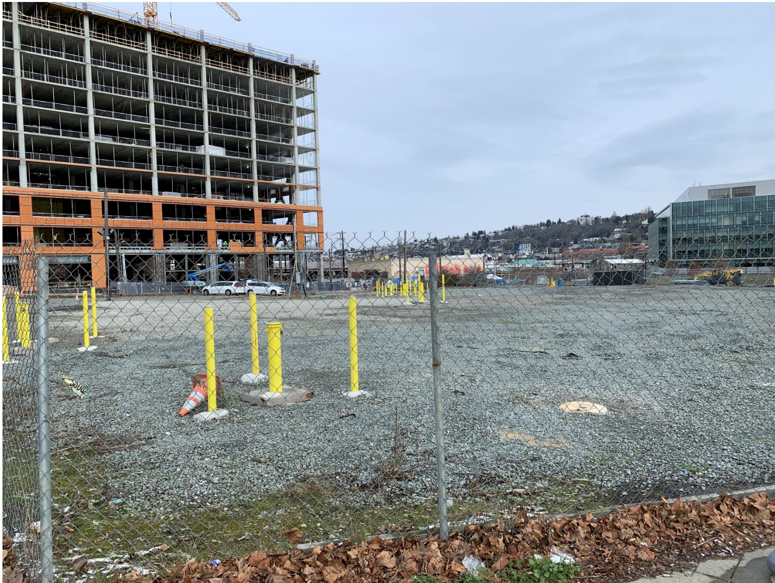
Figure 3. Seattle DOT Mercer Parcels looking northeast, February 2021. The redevelopment at the American Linen site is on the left.
