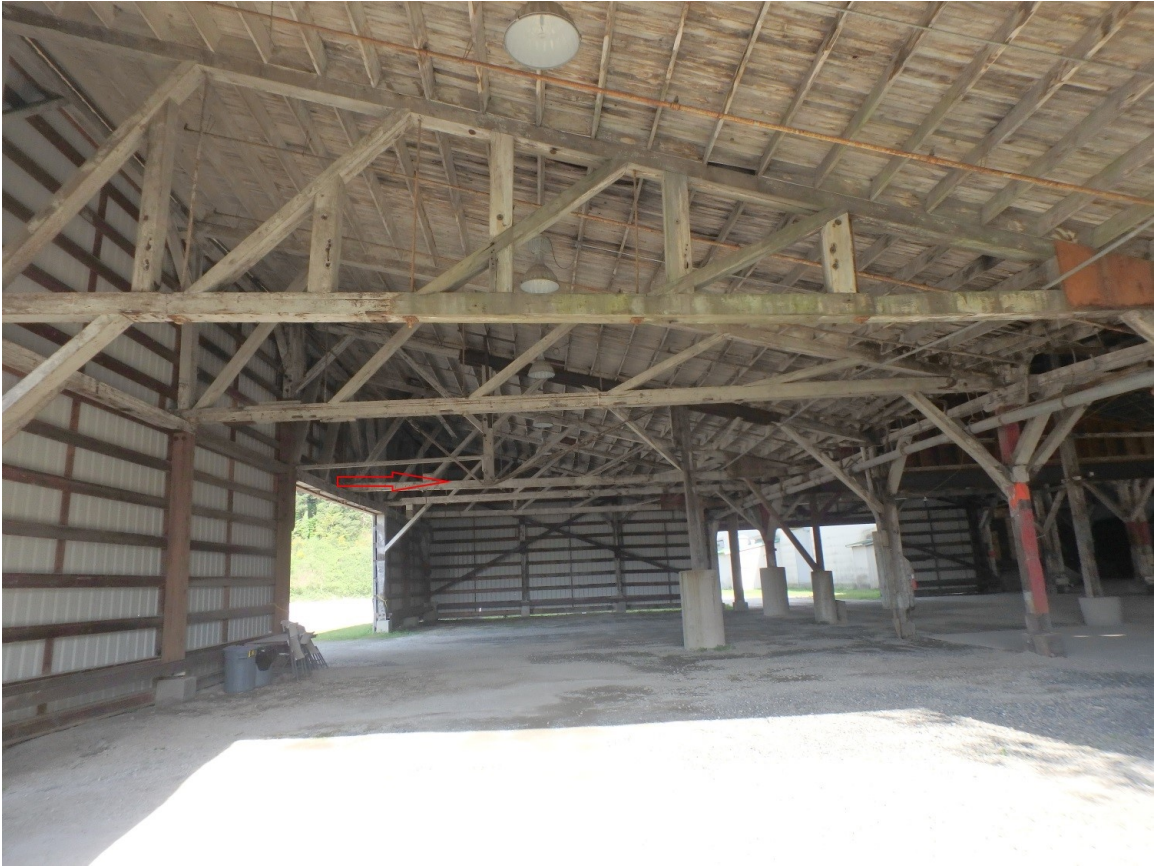
Figure 35. Interior of the Planing Mill's northernmost section. Facing east. Red arrow points to cut-off post supported by metal trusses.
