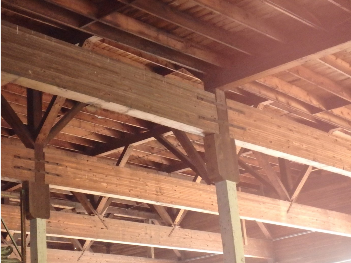
Figure 39. Detail of the structural system in the main section of the Finished Lumber Shed.
