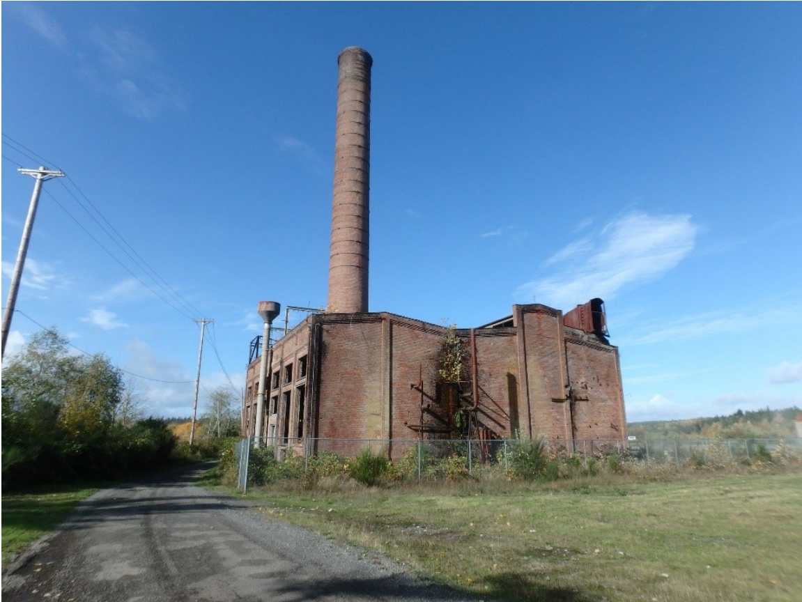
Figure 20. Power Plant south and east elevations. Taken October 2017. Note: The power poles run wire from a modern transformer station 150 ft. southeast of the power plant.
