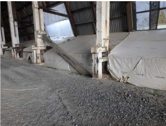
Interior - detail where east wall failed
