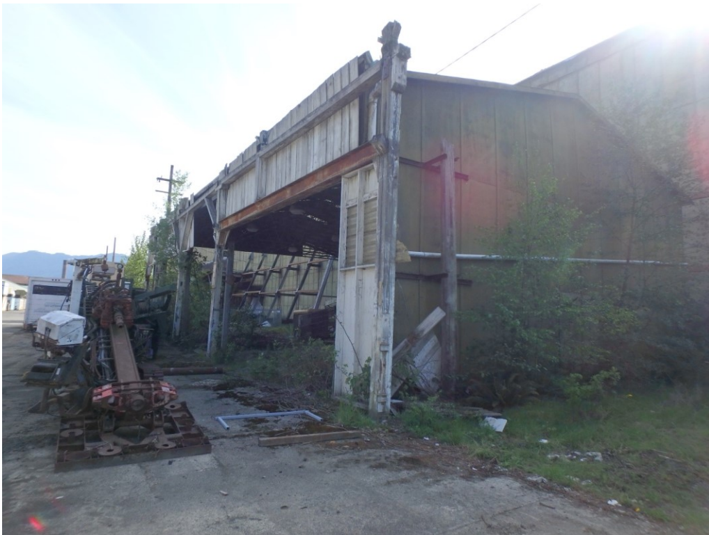
Figure 44. Modern (ca. 1980) shed between the Package Lumber and Finished Lumber sheds. The date of construction is based on aerial images and historic maps. Except for the metal roof system, the building appeared to be made of scrap material.
