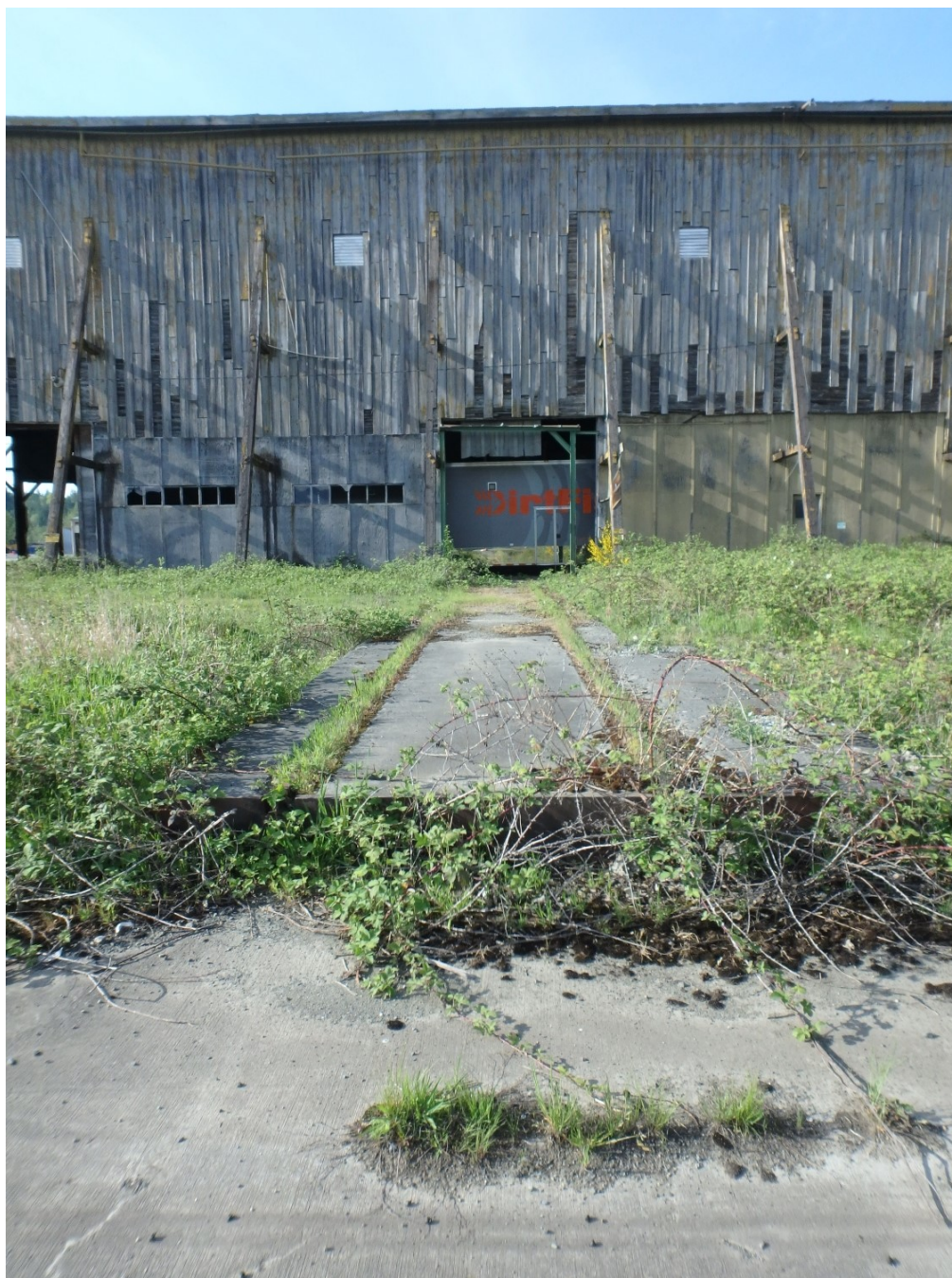
Figure 28. Rails approximately 225 ft. west of the east end of Crane Shed No. 3, facing north.
