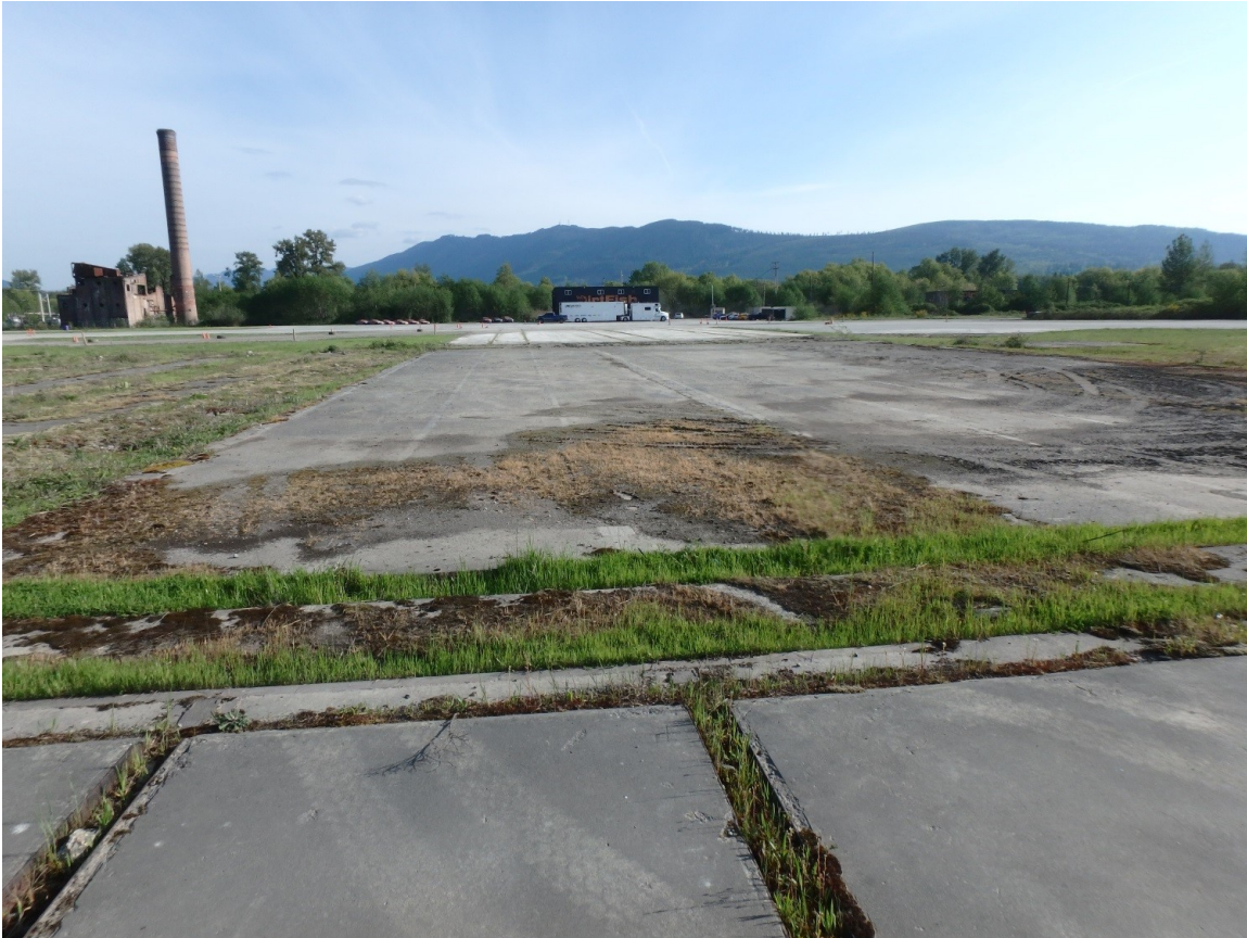
Figure 30. Loading Tracks taken from the northernmost section looking south across the other two sections. Also shown are the Power Plant (left) and modern DirtFish Rally building (middle background).
