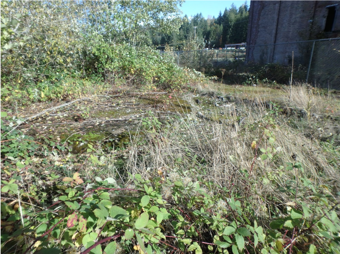
Figure 22. Concrete exposed at the location of the Fuel Vault, facing northeast. Northwest corner of the Power Plant (upper right).
