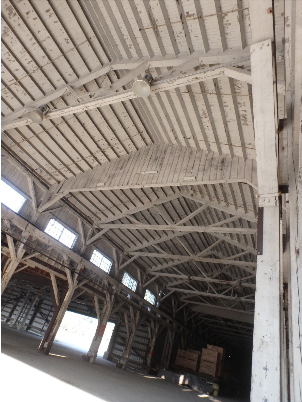
Figure 34. Interior of the Planing Mill-Crane Shed. Facing northeast. A portion of the first shed roof section is visible.
