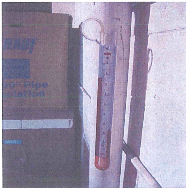
8-6-07 VIMS-4 Hudson Bay Warehouse (Facing Northwest) – Manometer installed
