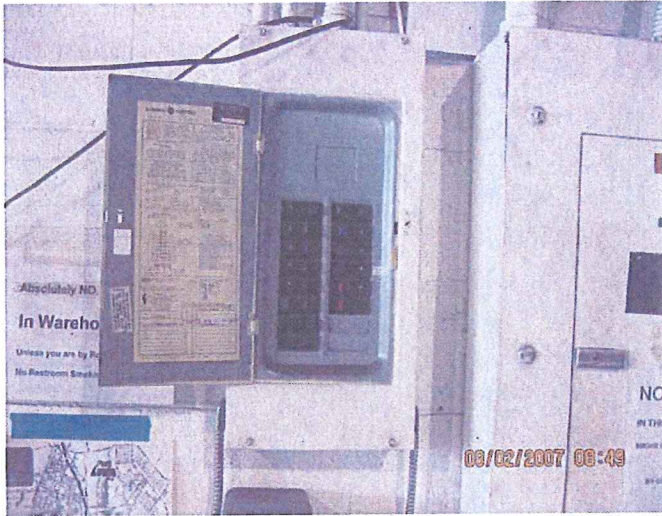
8-2-07 Hudson Bay Warehouse (Facing South) -Electrical box for exhaust fan
