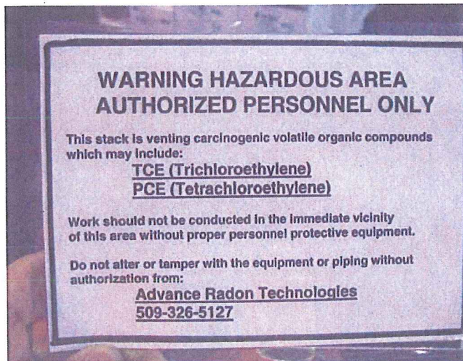
8-6-07 Exhaust Fan– Sign placed on PVC exhaust pipe
