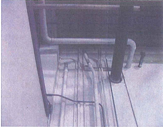
8-3-07 VIMS-5A Puget Sound Pipe (Facing South and Up) – Piping coming through Hudson Bay internal wall to Puget Sound Pipe.
