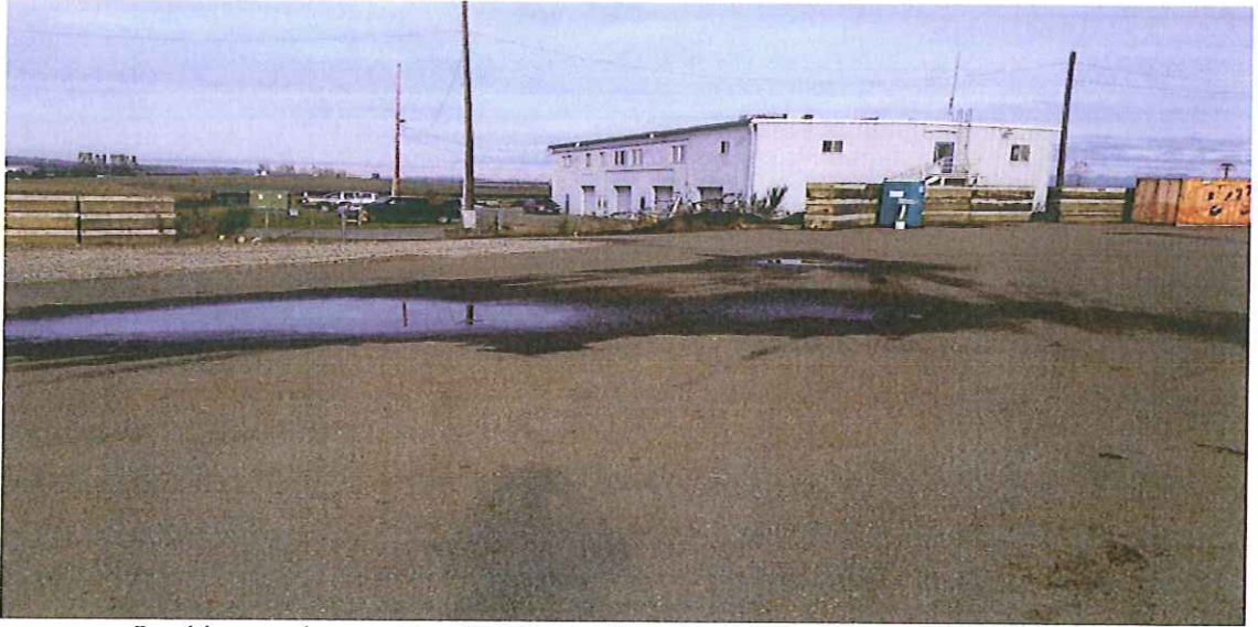
Looking northwest towards entry road. Areas of ponded water on pavement.
