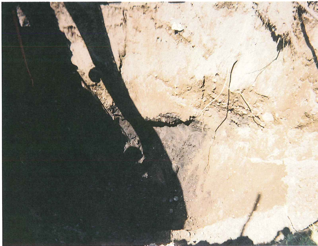
PHOTO 6: CONTAMINATED SOIL IN BASE OF EXCAVATION BEFORE PROJECT COMPLETION
