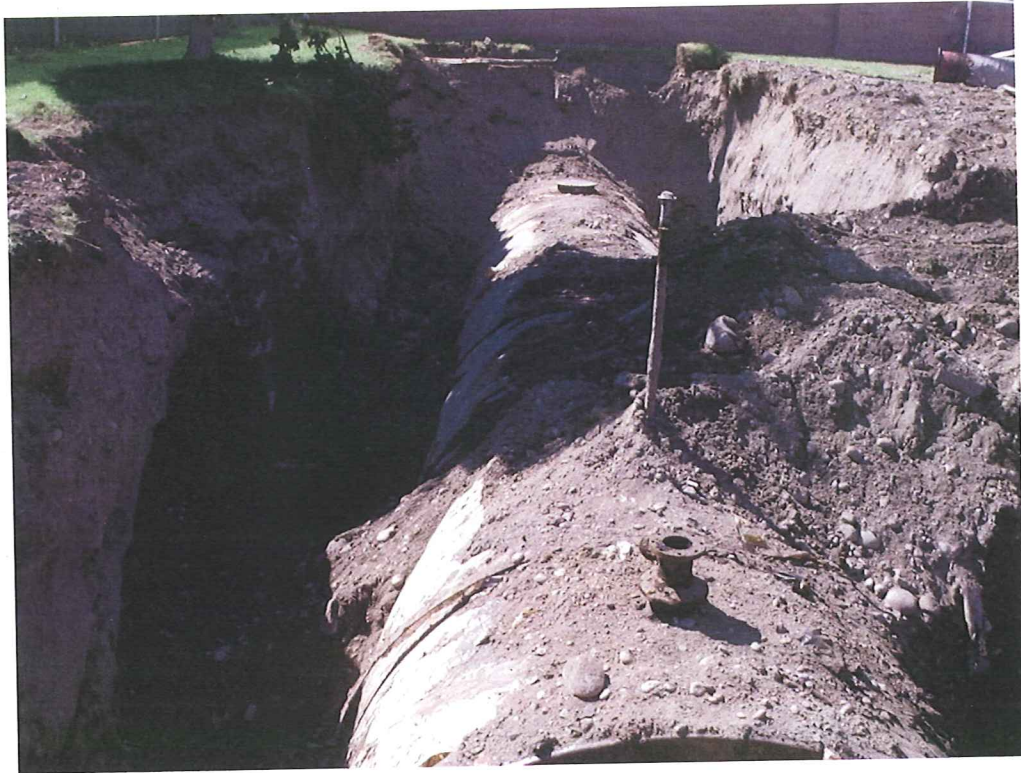
PHOTO 3: TOP OF TANK SHOWING UPPER CONNECTIONS
