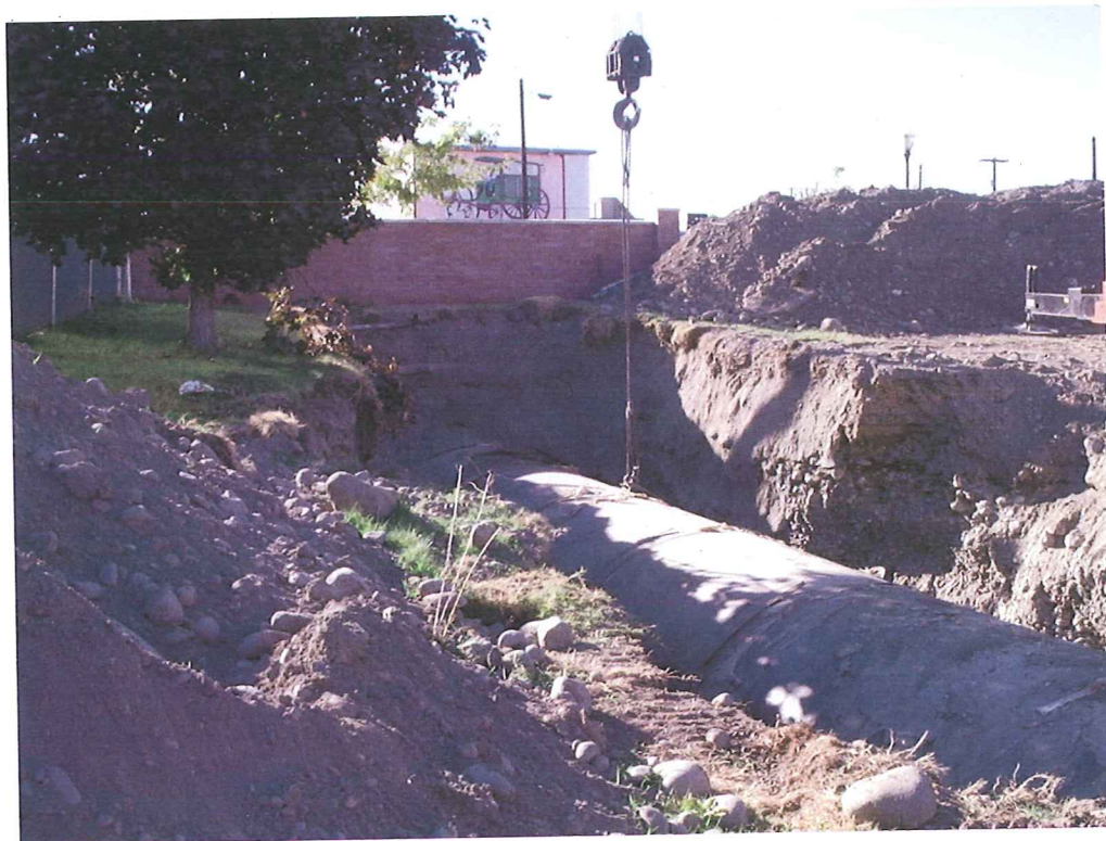
PHOTO 2: LOOKING NORTH WEST AT TANK IN TANK BASIN
