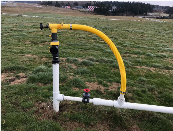
Installed Well Heads at E-37
