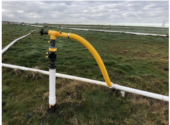
Installed Well Heads at E-41
