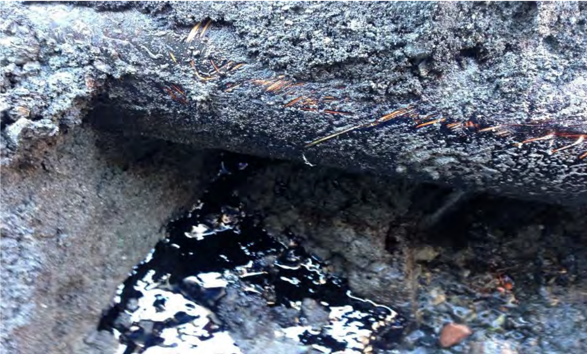
Bunker C ASTs excavation: bunker oil product
