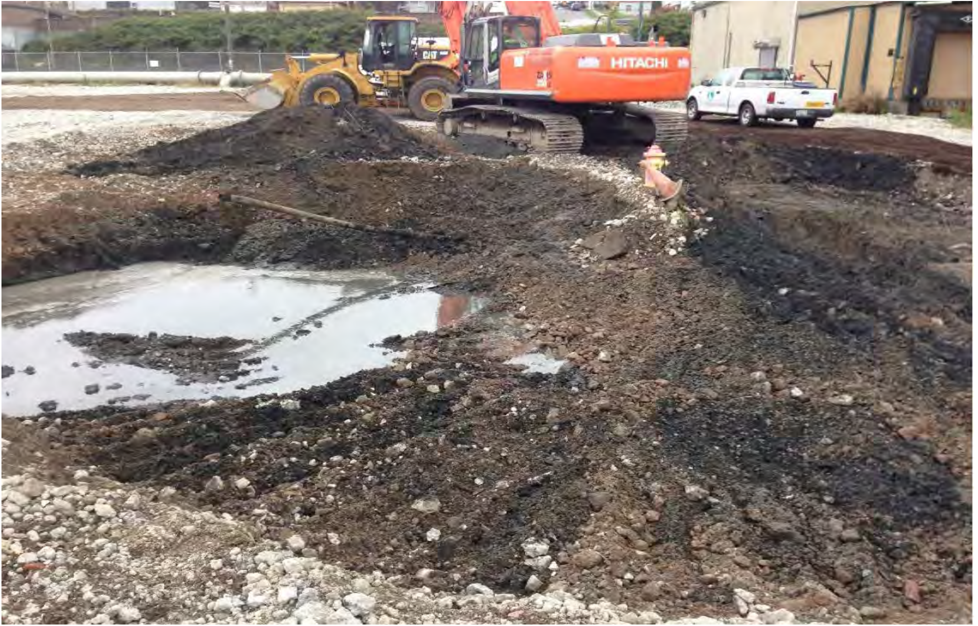
REC2-MW-5 excavation: looking east with black petroleum contaminated stained soil
