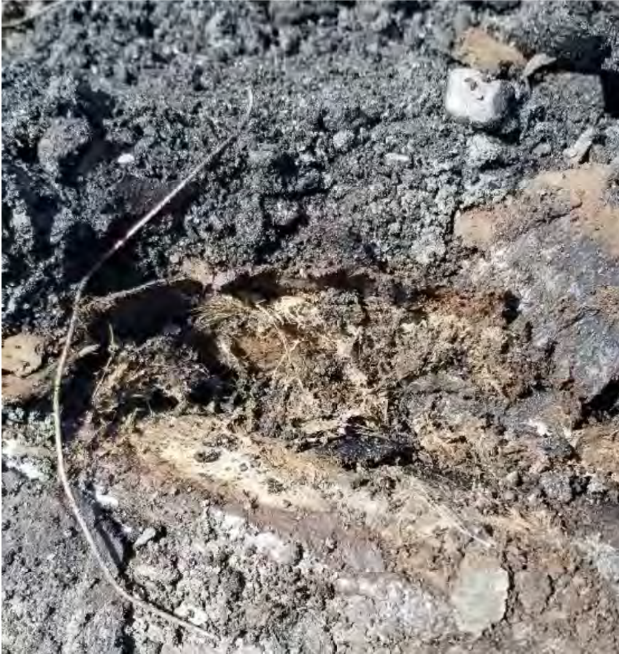
Asbestos-containing material insulation on pipes
