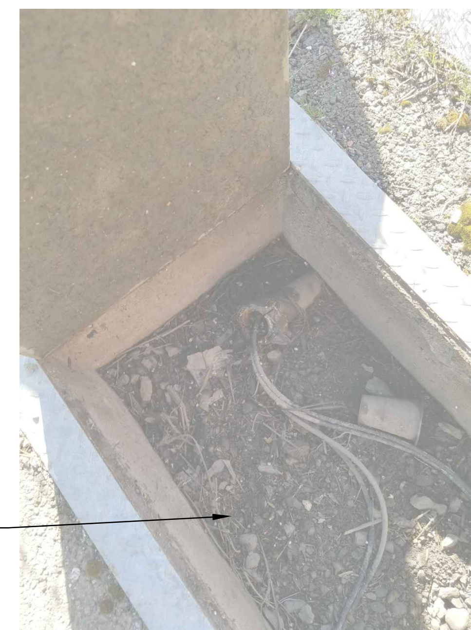
EXISTING HANDHOLE PHOTO 2 -
