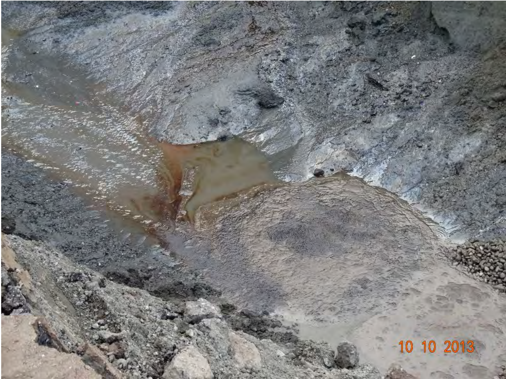
Bunker C ASTs excavation: bunker oil product
