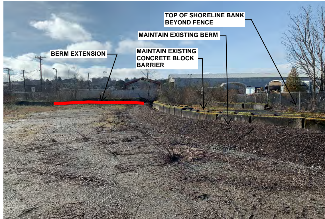
P2 - END OF BERM AT SOUTH END LOOKING SOUTH. BERM WILL BE EXTENDED 85-FEET TO FORM A CONTINUOUS BARRIER WITH NO GAPS. BERM WILL TIE TO AN EXISTING CONCRETE BLOCK BARRIER.
