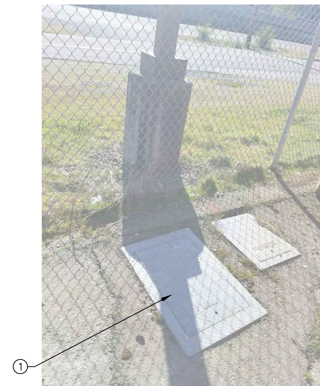
EXISTING HANDHOLE PHOTO 1 -
