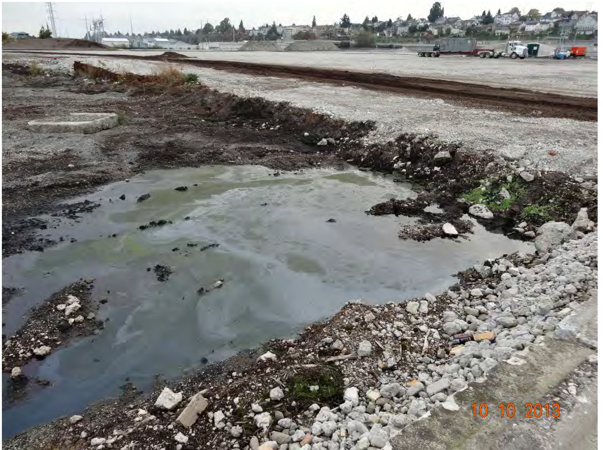
Excavation with oily sheen on the water
