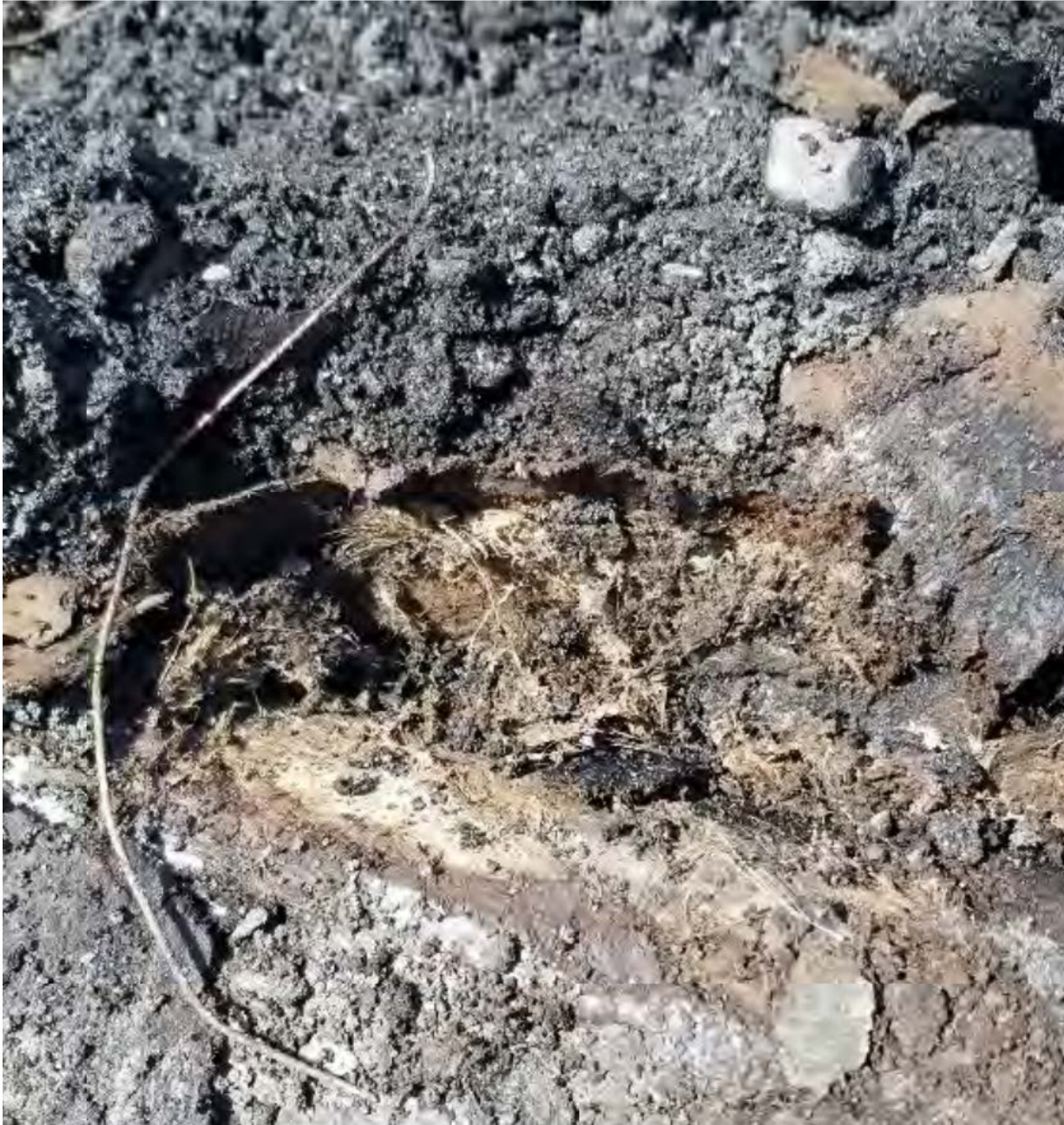
Asbestos-containing material insulation on pipes
