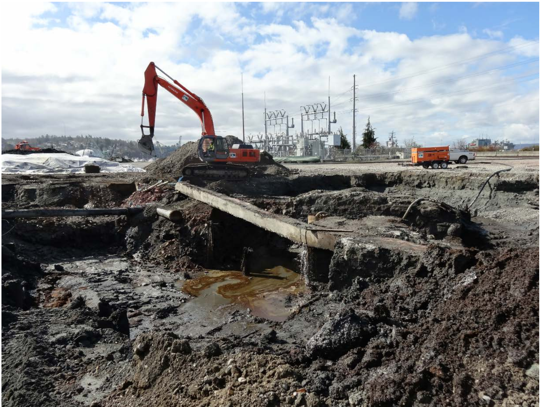
Clark-Nickerson Area Excavation: oily sheen on the water; petroleum contaminated sawdust
