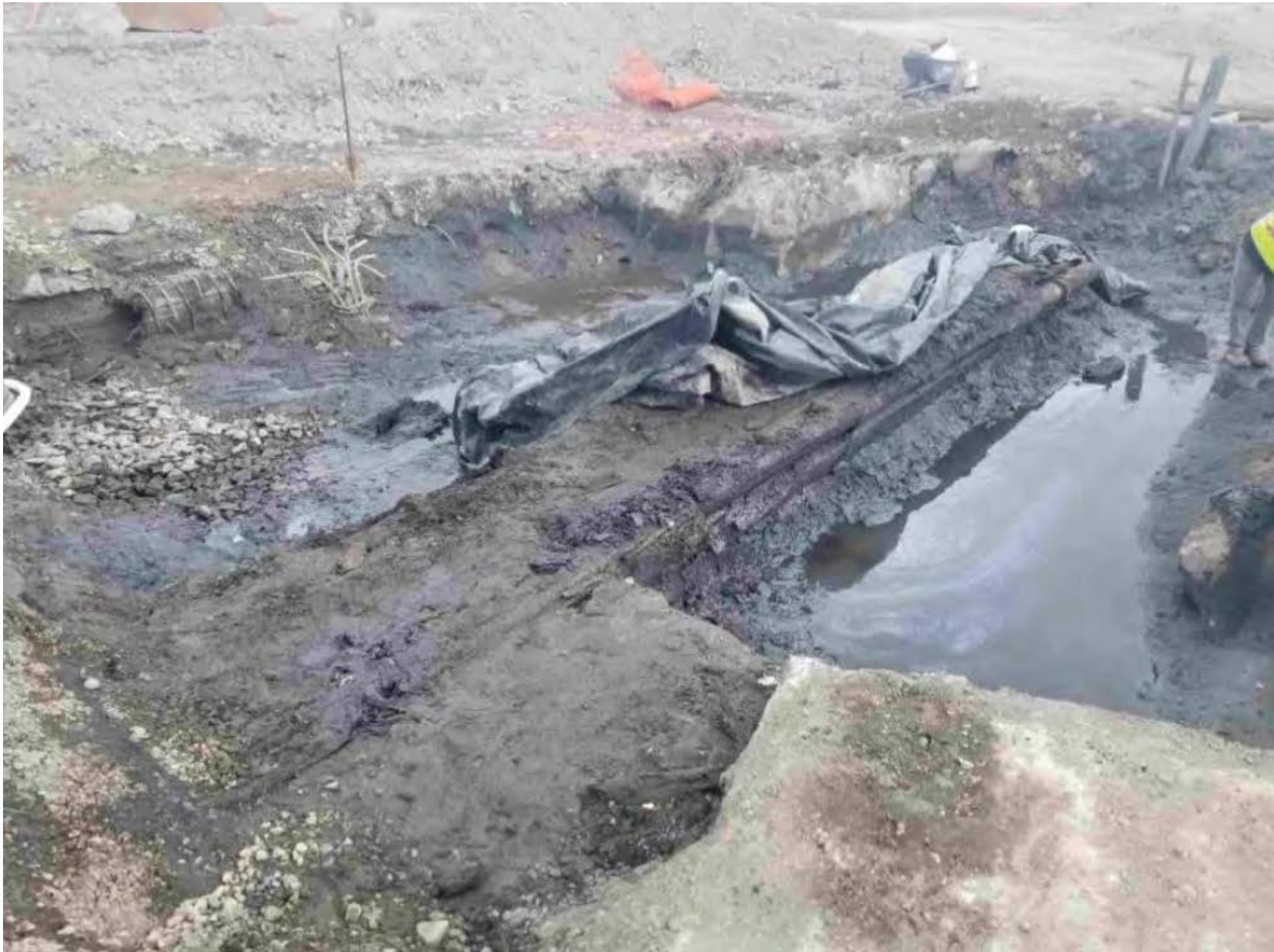
One Bunker C fuel pipe encountered within wooden conduit, stained soil with sheen on water, looking north
