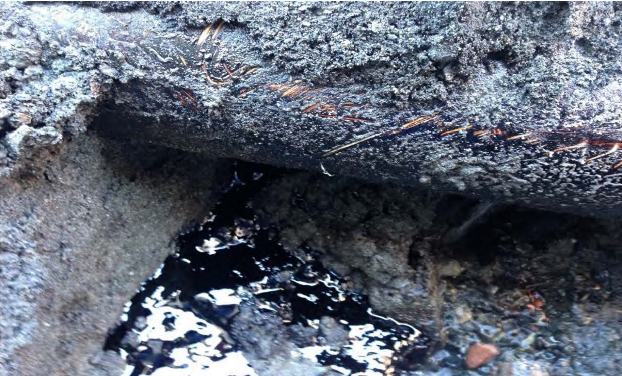
Bunker C ASTs excavation: bunker oil product
