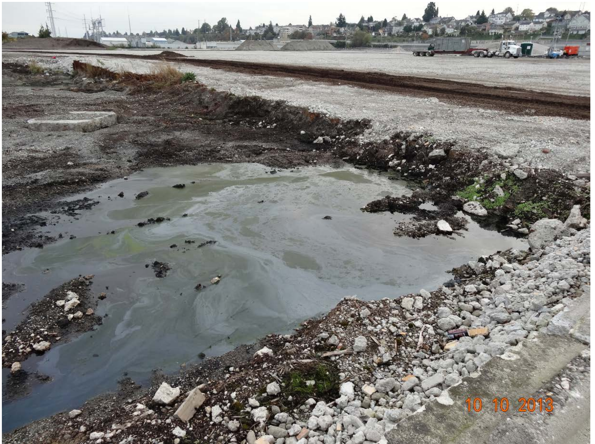
Excavation with oily sheen on the water
