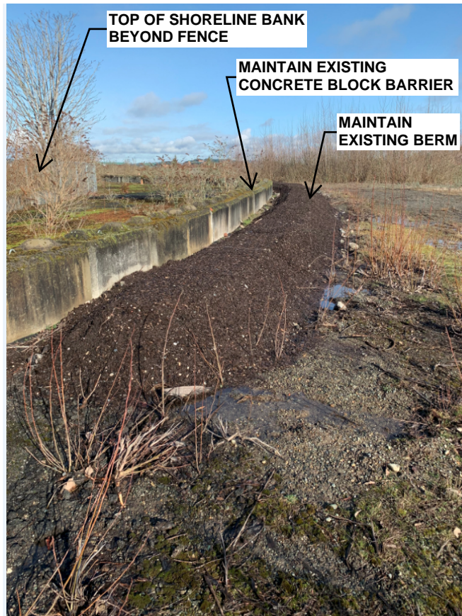
P1 - END OF BERM AT SOUTH END LOOKING NORTH. BERM WILL BE EXTENDED 85-FEET TO FORM A CONTINUOUS BARRIER WITH NO GAPS. BERM WILL TIE TO AN EXISTING CONCRETE BLOCK BARRIER.
