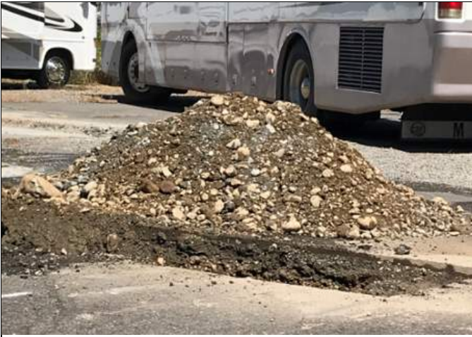
Picture Date: Wednesday 07/29/2020 Picture Taken By: Haley Provinsal Picture Location: Milton, Washington Project Name: USG Highway 99 Site Description: 99-TP-1 Top 3 ft of material
