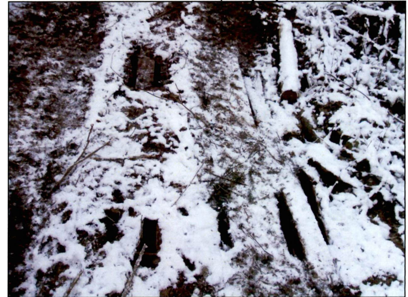
Middle View of Grid V-18 (dilapidated bridge)
