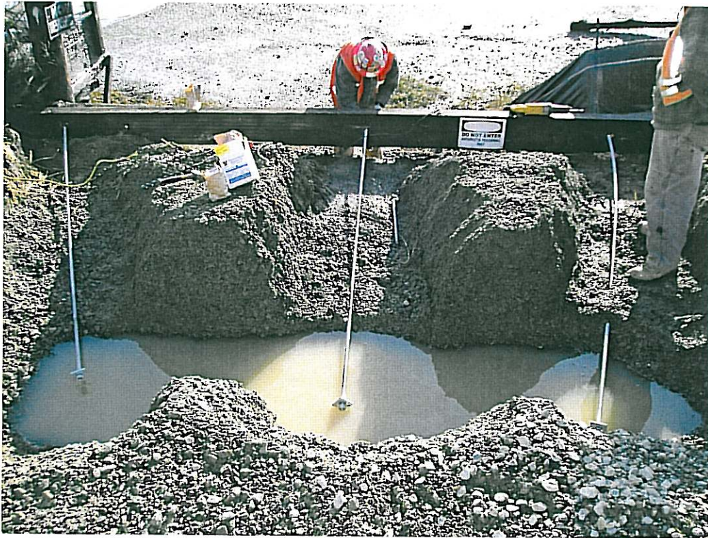
Photograph 18: Replacement of tension rods and preparation for emplacement of concrete earth anchors.
