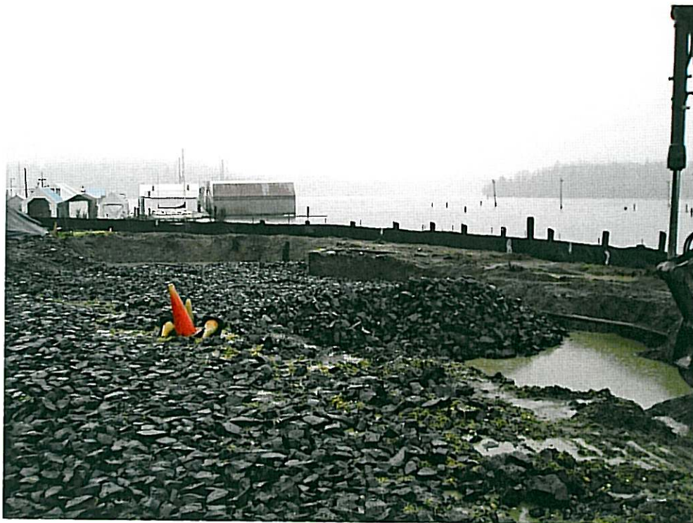
Photograph 9: Excavation on southern portion of the Site. (Note: Oil-water separator in center of photo)
