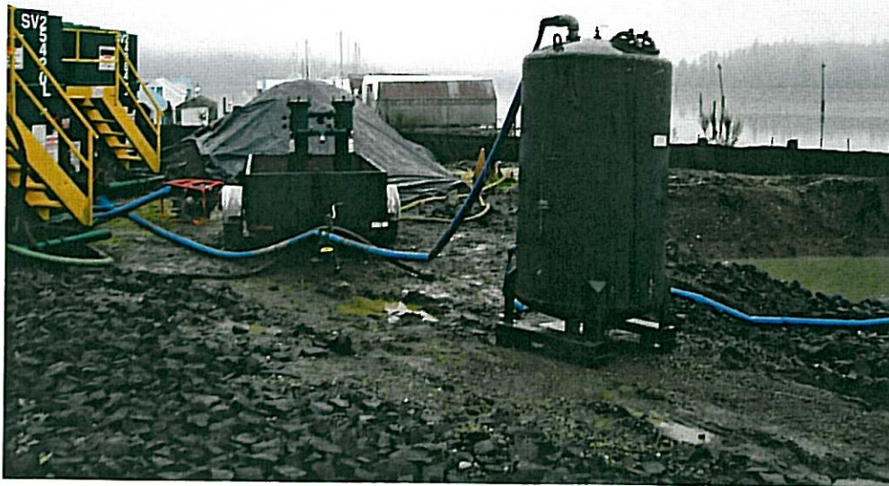
Photograph 5: Wastewater treatment and discharge.
