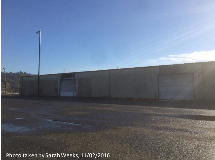
Figure 3. Northern exterior of the building, looking southeast. Missing panels above northwest garage door.
