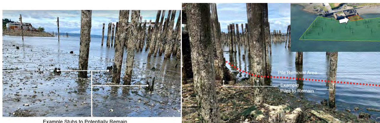
Figure 4 - Pile Stubs to potentially remain (left) and Nearshore Piles to Remain (right)
