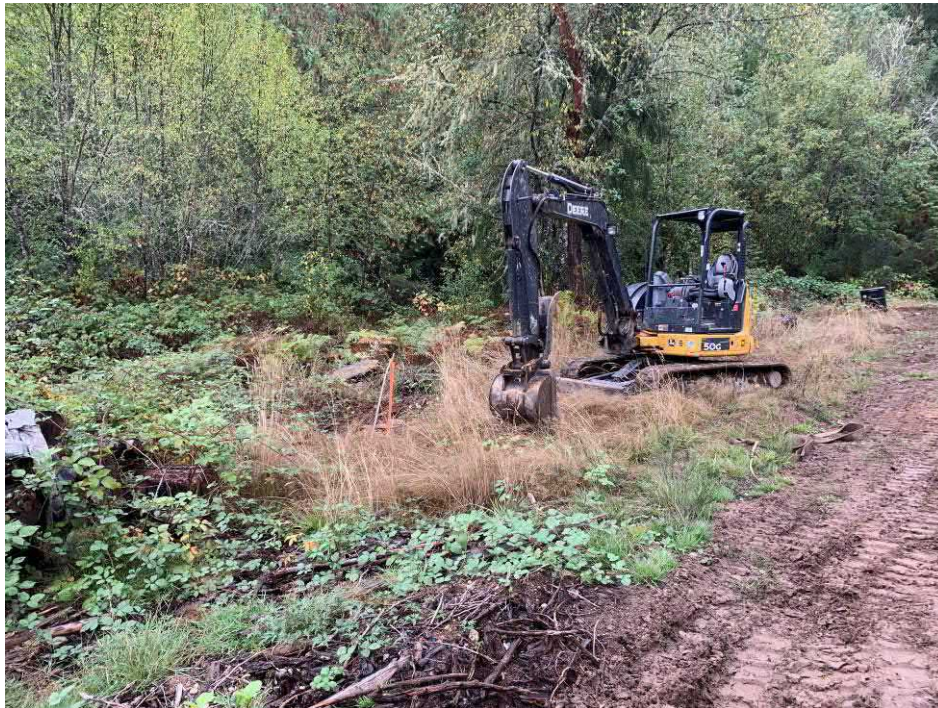
Photo 12: 9-27-21 Remedial Action Soil Removal – Showing soil removal in the former house and drum area.
