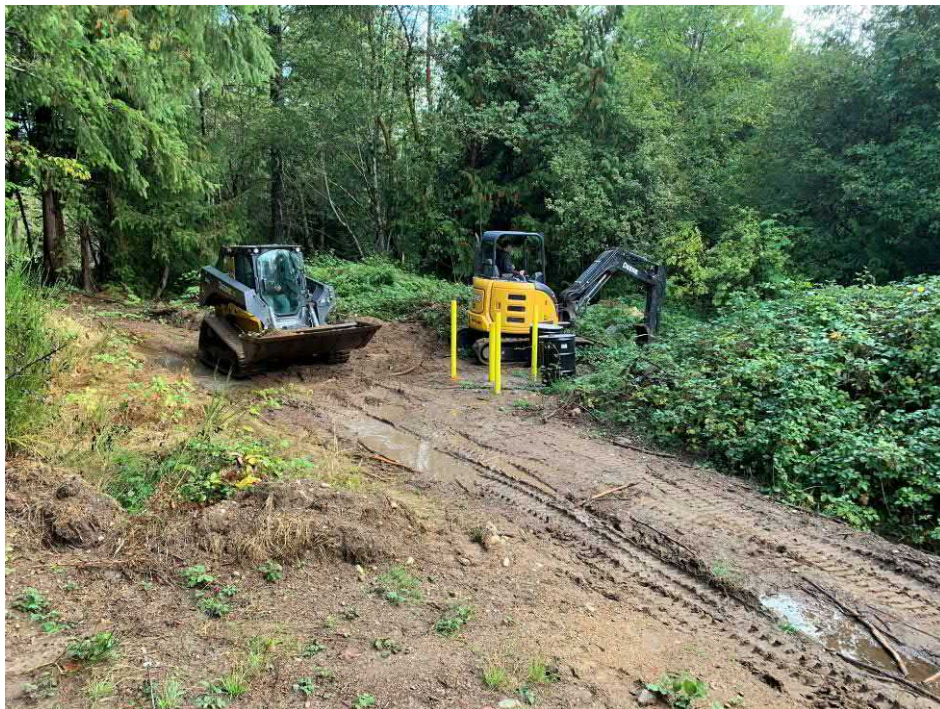
Photo 10: 9-27-21 Remedial Action Soil Removal – Showing soil removal in the area of former debris pile 1.
