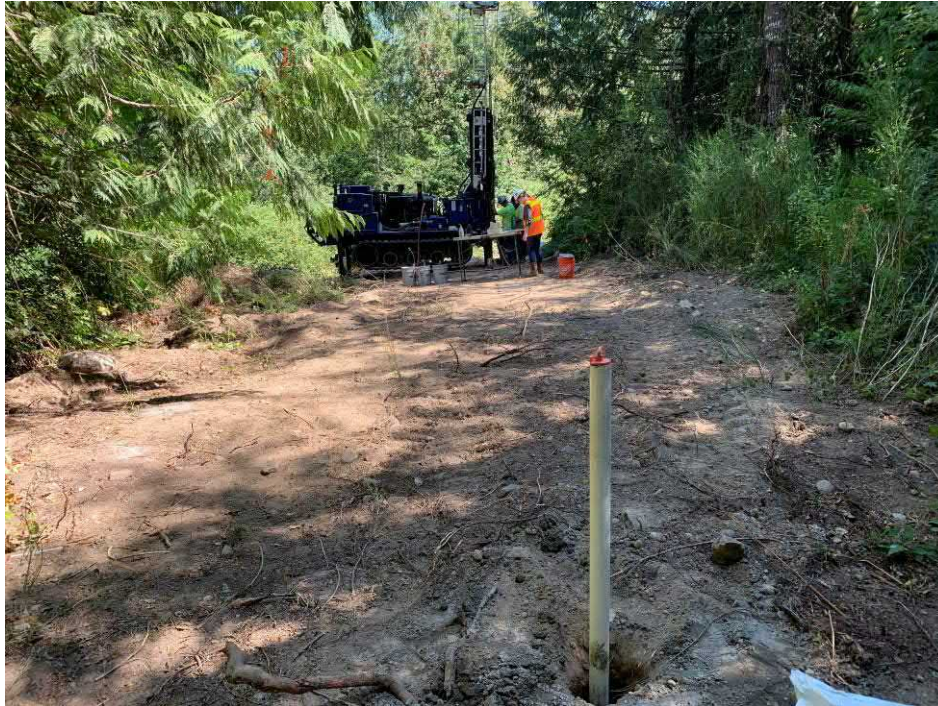
Photo 5: 7-12-21 Monitoring Well Installation – Showing installation of Monitoring Well MW-3 in the former drum storage area with completed MW-1 in foreground.
