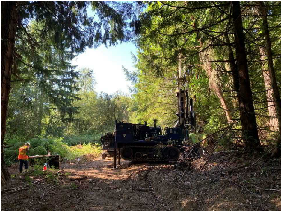
Photo 6: 7-12-21 Monitoring Well Installation – Showing installation of Monitoring Well MW-2 adjacent to the former drum storage area.
