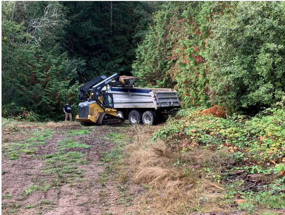
Photo 14: 9-27-21 Remedial Action Soil Removal – Showing some of the removed soil being placed in the truck for transport to offsite disposal site.
