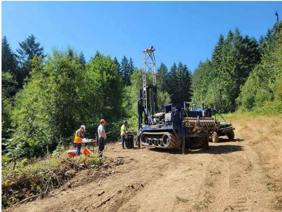
Photo 8: 7-13-21 Monitoring Well Installation – Showing installation of Monitoring Well MW-5 in the area of former debris pile 2.
