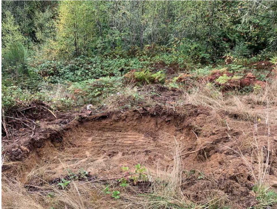
Photo 13: 9-27-21 Remedial Action Soil Removal – Showing limits of the soil removal excavation in the former house and drum area.
