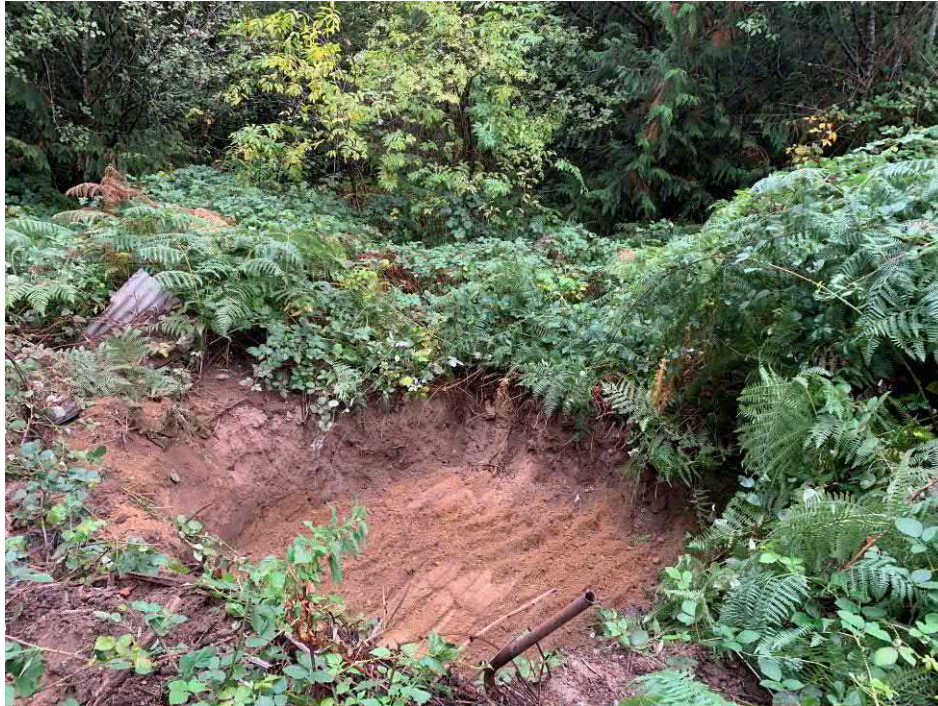
Photo 11: 9-27-21 Remedial Action Soil Removal – Showing the limits of the soil removal excavation in the area of former debris pile 1.
