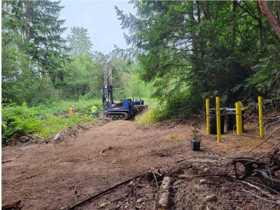
Photo 7: 7-13-21 Monitoring Well Installation – Showing installation of Monitoring Well MW-4 in the area of former debris pile 1.
