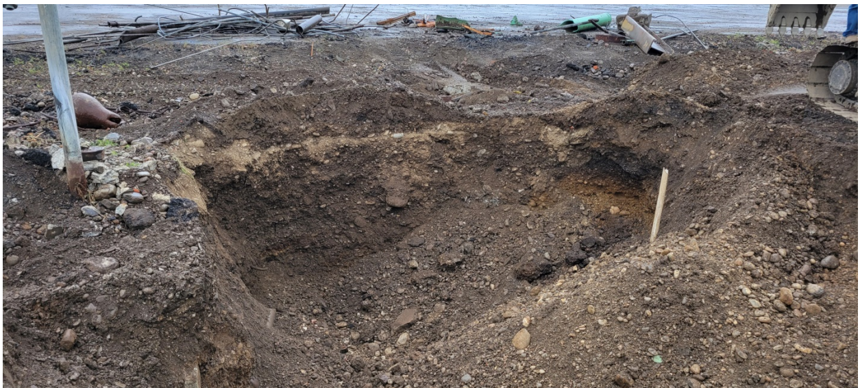
Questionnable soils below wash bay drain (excavated until clean) May 2021
