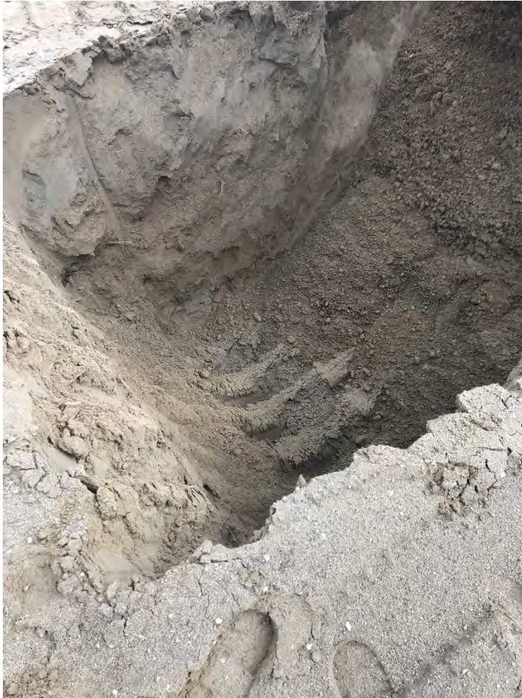
Photograph 3. Typical pot hole observation - no landfill material observed.
