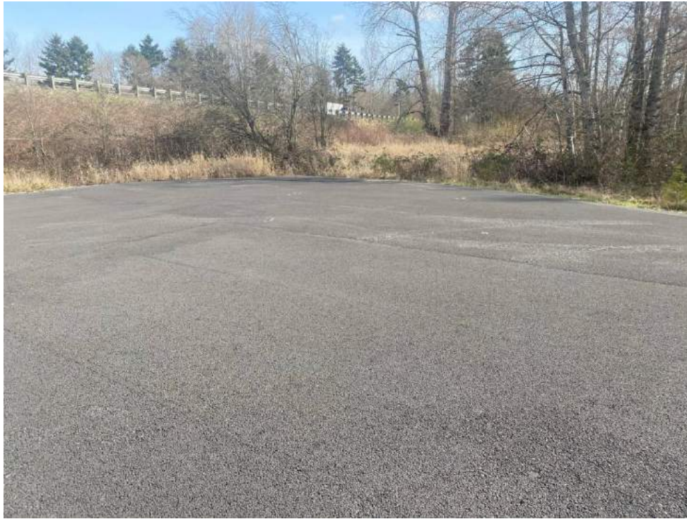
Photograph 5. Good cap conditions at the northeast corner of the DMCA at station DMCA 04 where previously noted debris was addressed by the Port.
