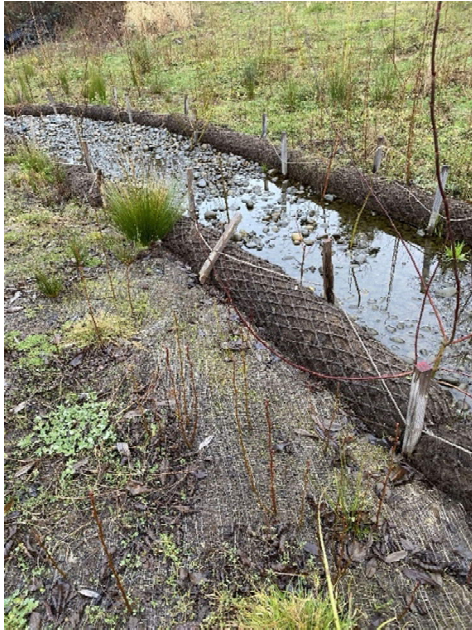
Photo 16: loose wattle stake
