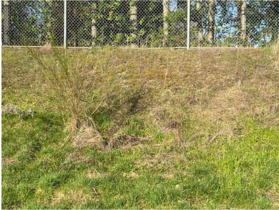
Photograph 11. Fair cap conditions on the slope of the east boundary between stations LLA 12 and LLA 13.
