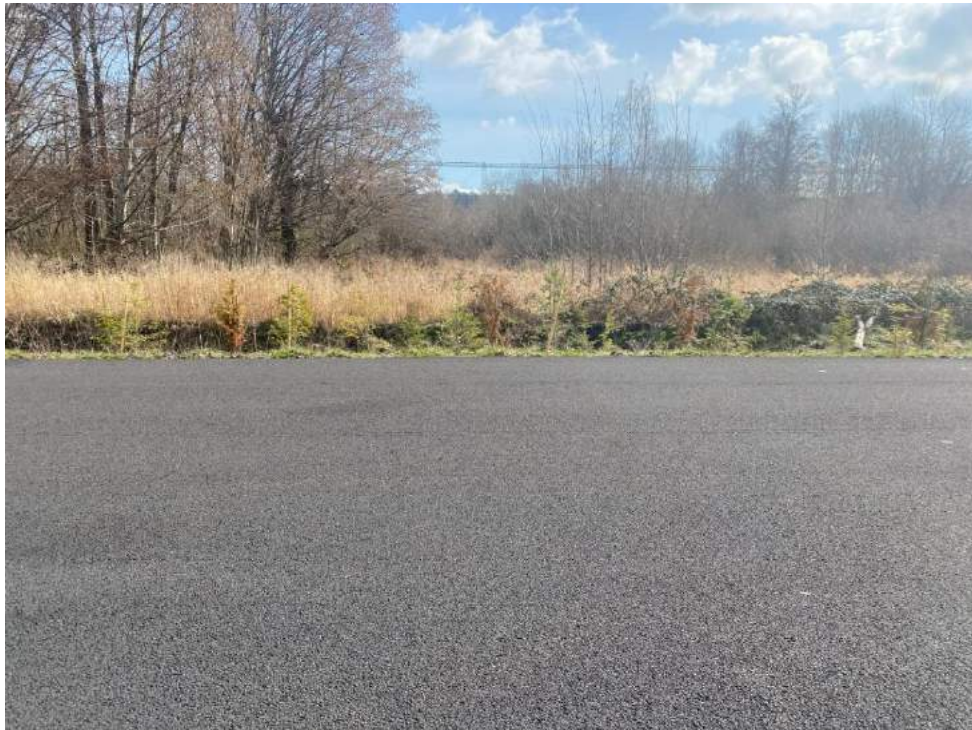
Photograph 6. Good cap conditions along the east boundary of the DMCA near stations DMCA 05 and DMCA 06 where previously noted debris was addressed by the Port.
