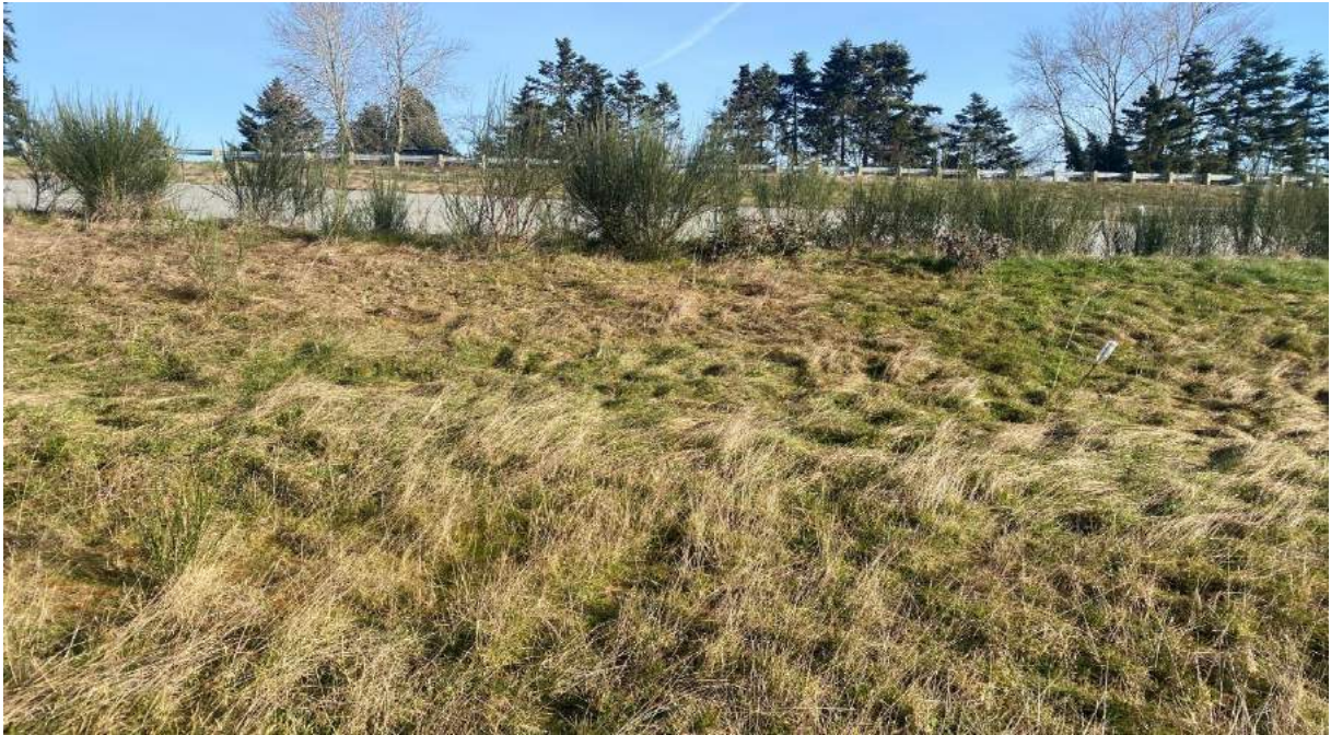
Photograph 3. Minimal plant overgrowth at the north border, including stations LLA 03 and LLA 04.
