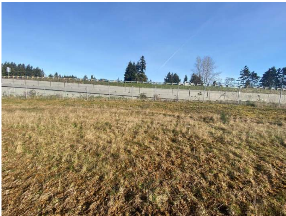
Photograph 6. Large 18' by 30' area of loss of barrier material at stations LLA 05, LLA 06, and LLA 25.
