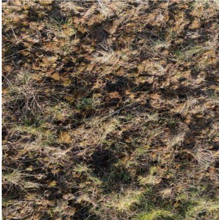
Photograph 5. Ground conditions requiring repair to address loss of barrier material at stations LLA 05, LLA 06, and LLA 25.
