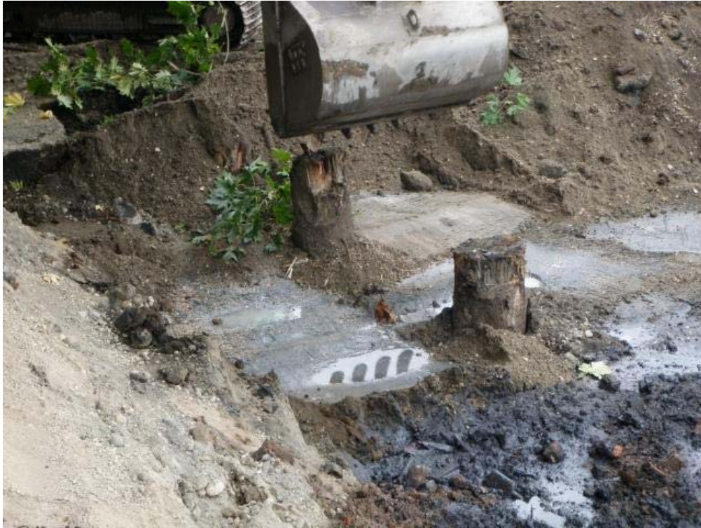
Photograph 7: Unpreserved wood piles (southeast corner of property)
