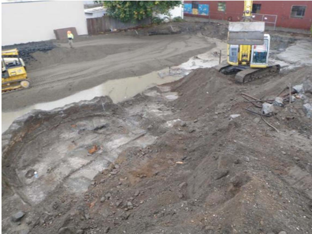
Photograph 5: Apparent concrete footing for the former gas holder (left side of photo) located towards the north-northwest portion of the site
