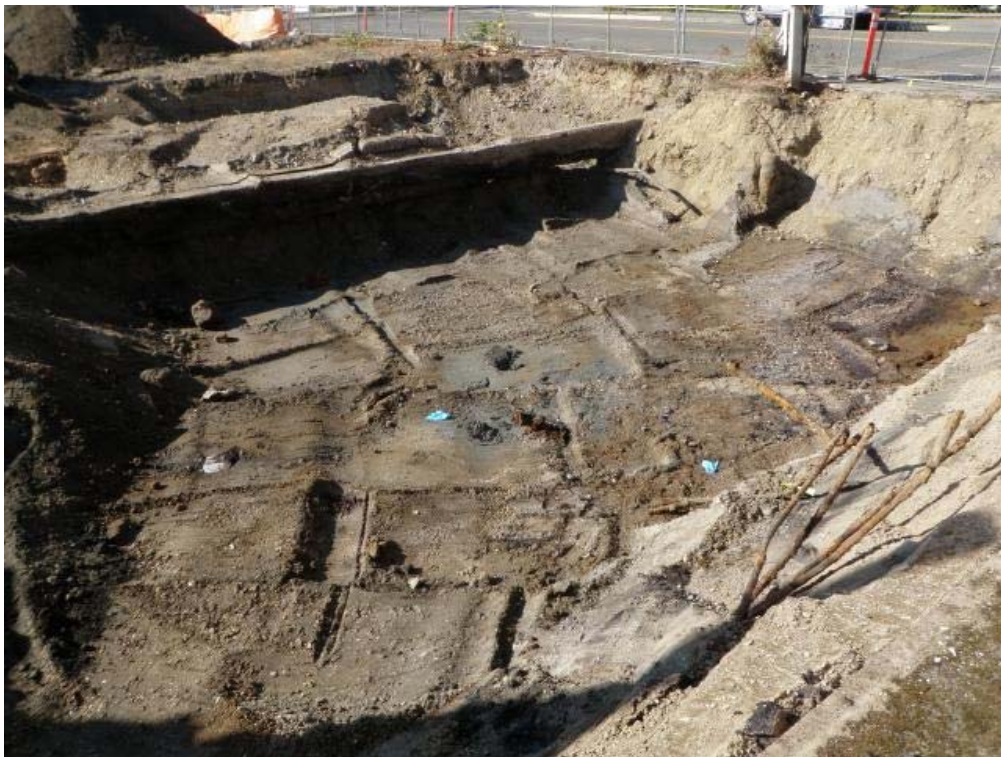
Photograph 4: Remnant underground piping (northeast corner of property)
