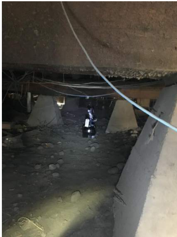
Photograph 5. Crawl space SUMMA canister located in the center of the crawl space. View to the west.
