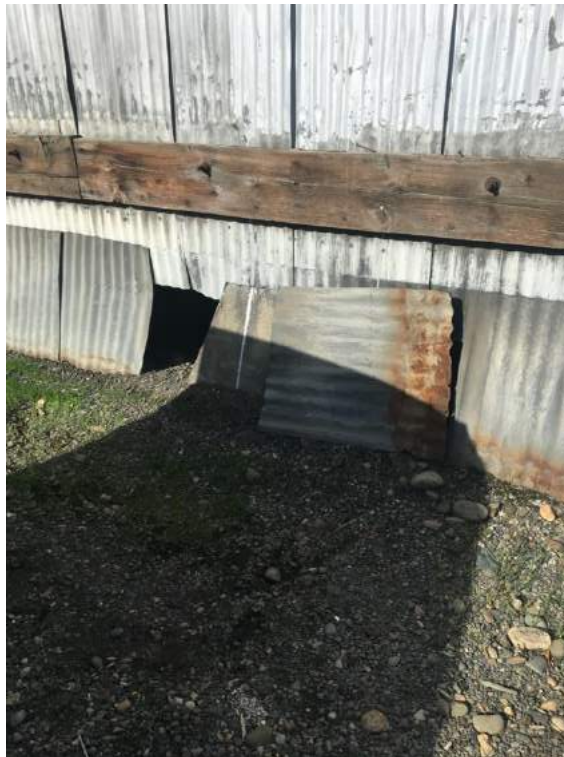
Photograph 4. Crawl space entrance located on the east side of the office space. View to the west.
