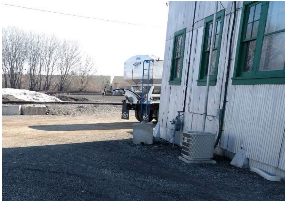
Photograph 3. Heat pump and AC unit on north side of office building, looking southeast.
