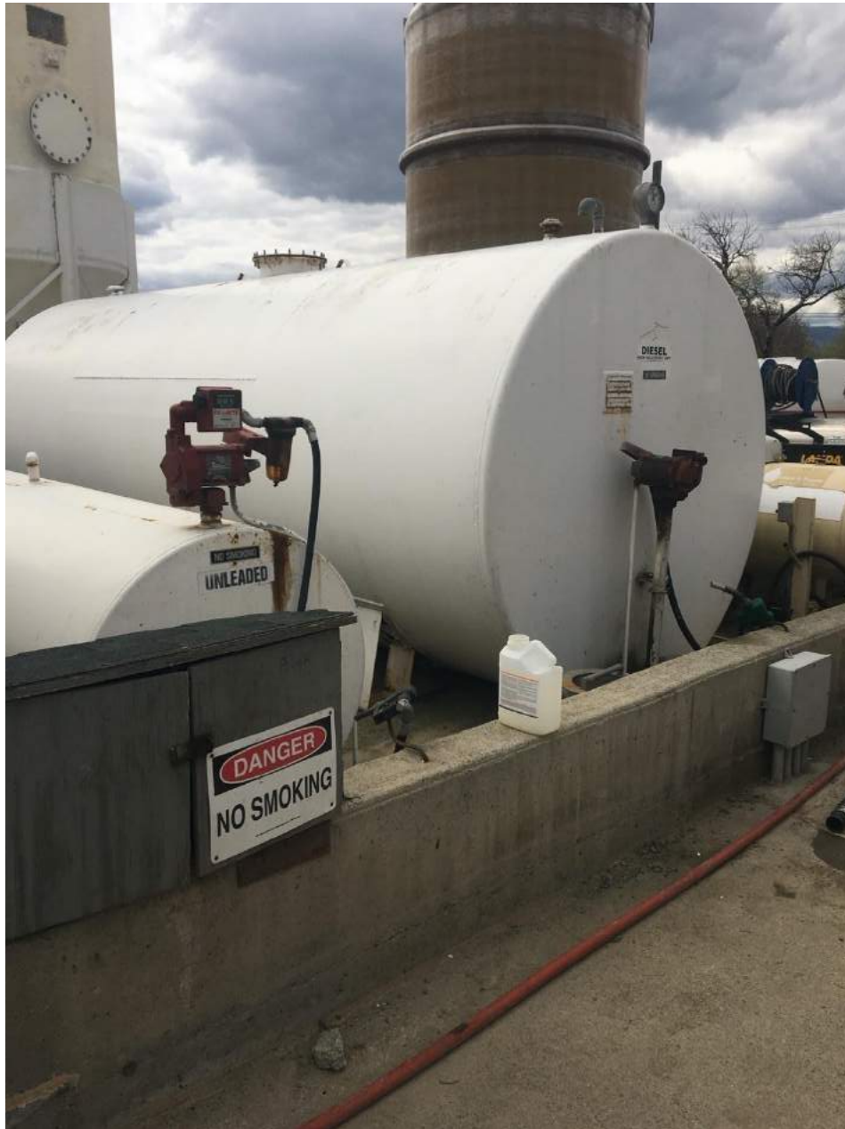
Photograph 9. Fuel aboveground storage tanks (ASTs) located south of the office building in AST containment area. View to the southwest.
