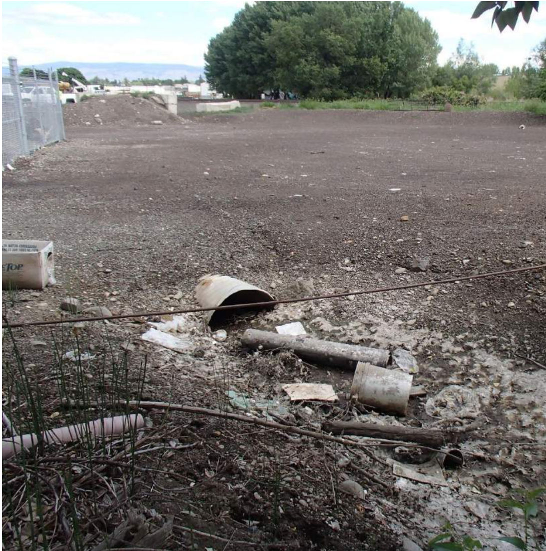
Photograph 23. Culvert daylighting in low area/ditch on Wales Property south of Smith-Kem Property (looking north). June 2017.
