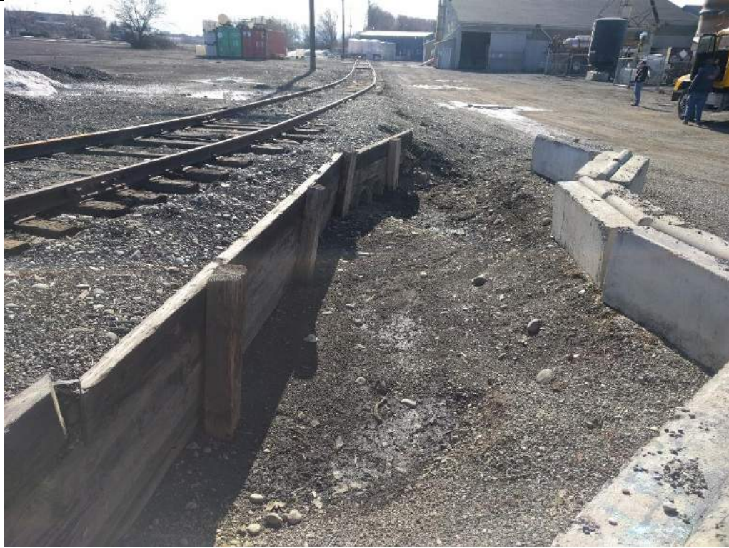
Photograph 13. Culvert adjacent to MW-4, located to the right of the Ecology blocks (looking south). February 2016.
