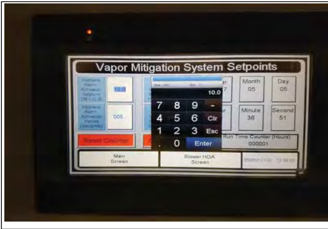
Photo 19: View of the VMS Control Panel - System Setpoints screen with the numeric touchpad active to help program in set point values or date/time values.
