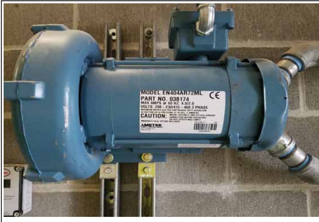
Photo 13: View of the Ametek Rotron EN404AR72ML regenerative blower that induces the vacuum and air flow from the sub-slab recover pipes.
