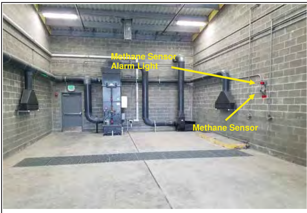
Photo 8: View of room "B" (from plans) looking to the west. Note the methane sensor and associated alarm light on the north wall (right side).
