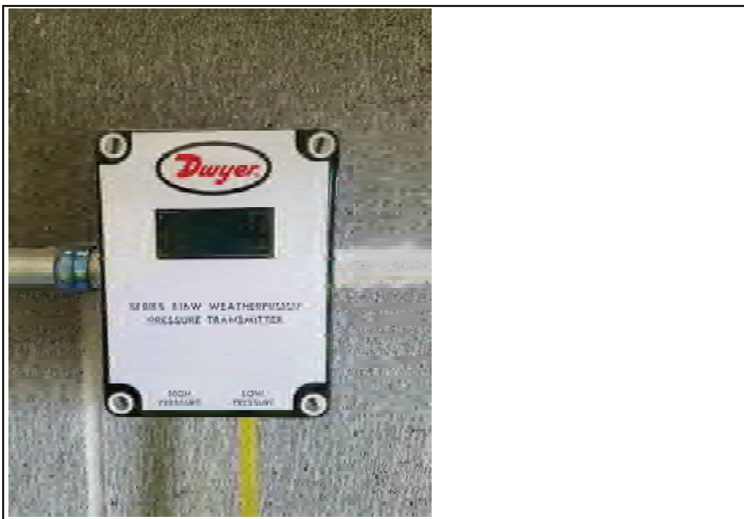
Photo 12: View of Dwyer differential pressure transmitter and screen. Transmitter reads in inches water column vacuum.
