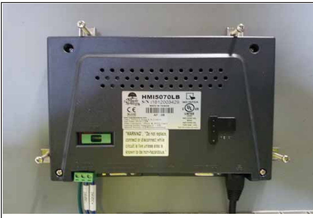
Photo 22: View of the back of the human-machine interface (touchscreen) on the back of the door panel inside the VMS Control Panel.
