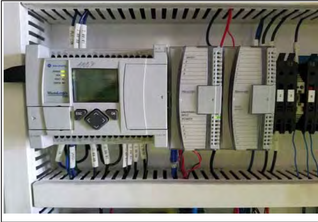
Photo 21: View of the VMS Control Panel Allen Bradley PLC unit (located in upper left of the control panel interior).
