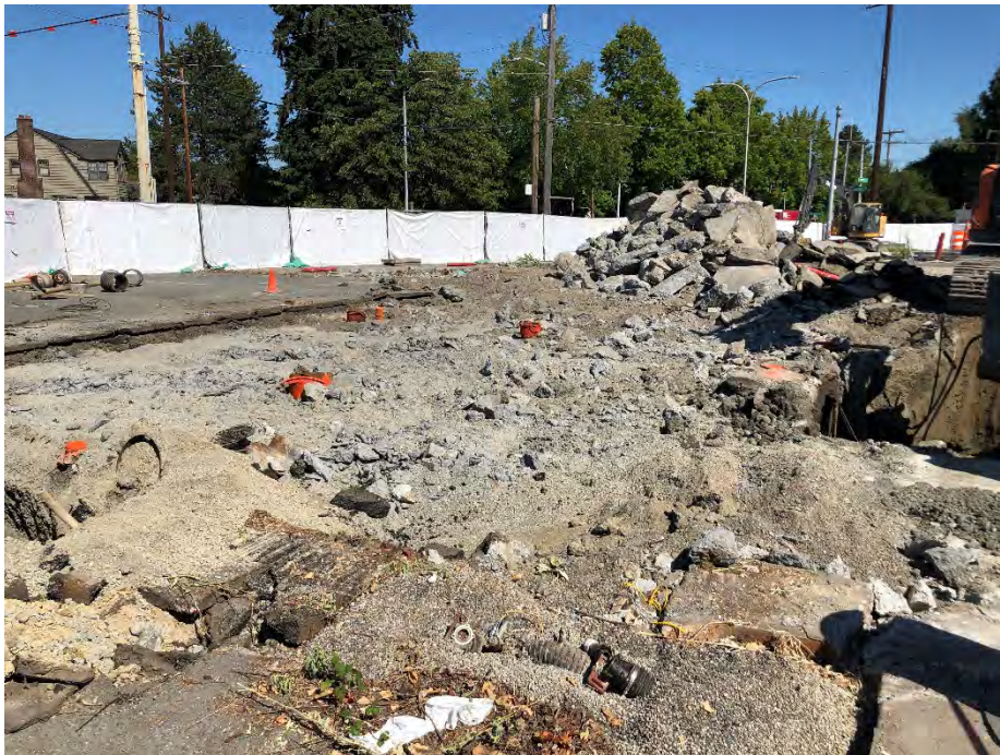
Photo 2. Removal of concrete and asphalt slabs in the northern portion of the Site in location of USTs prior to removal. UST fill ports are painted orange for visibility. July 19, 2021.
