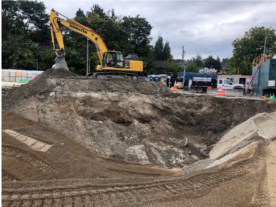
Photo 19. Over excavation of sample location B2. South sidewall and location of sample X5 visible in right of frame. September 21, 2021.
