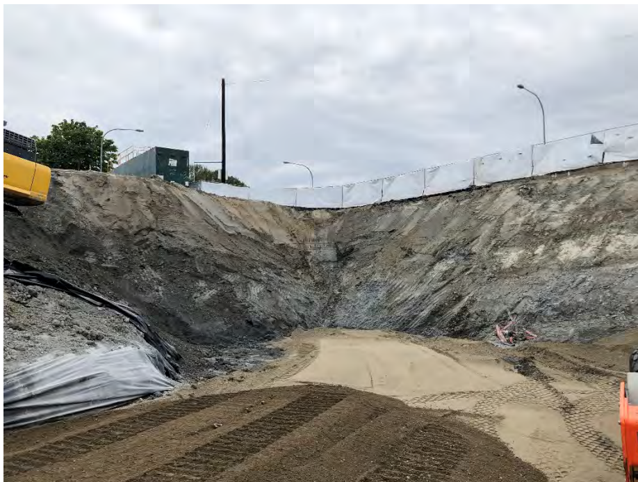
Photo 14. Final extent of August 20-21 over excavation near sample location D1 as seen looking west from bottom of pit. Backfill of Stage 2 excavation has begun, and the first lift of Type 17 aggregate backfill is visible at bottom of pit in foreground of frame. August 21, 2021.
