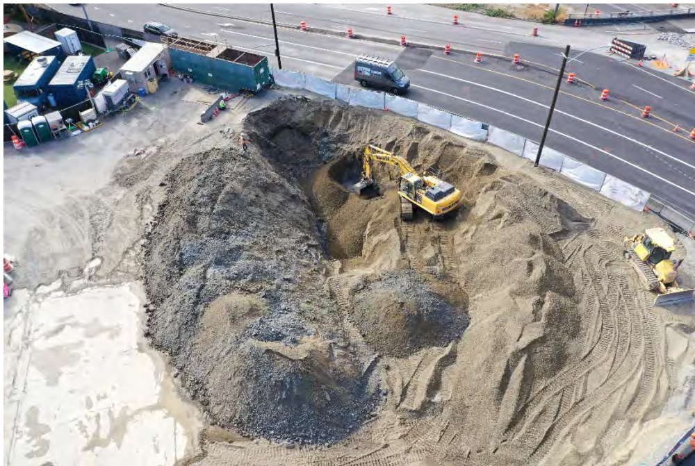
Photo 18. Over excavation west of sample location B2. Majority of Stage 2 excavation backfill complete. Gray contaminated soil pending load out visible in left of frame. September 13, 2021.
