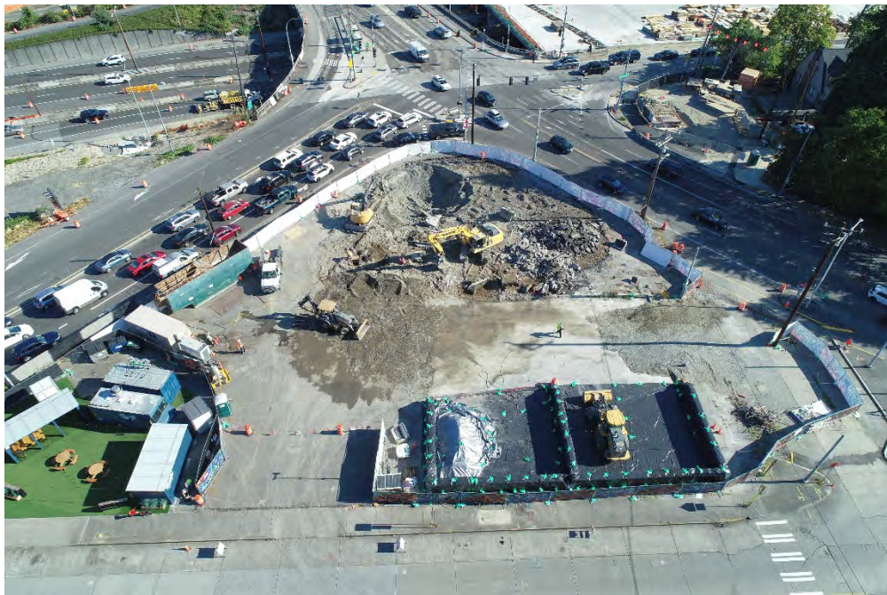
Photo 6. Site following removal of USTs. Excavation from UST removal visible near top of frame. Containment bays for temporary soil storage visible in bottom of frame. July 23, 2021.
