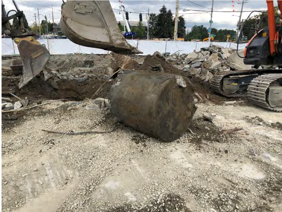
Photo 5. Removal of 500-gallon waste oil UST. UST was formerly filled with concrete slurry. July 21, 2021.
