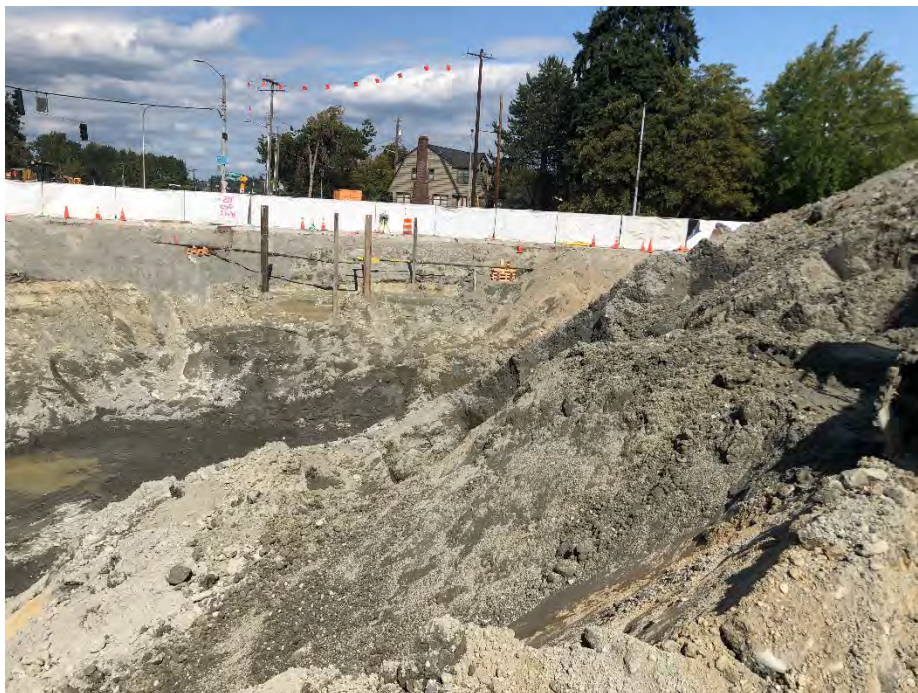
Photo 12. Looking east across excavation. PSE gas line supported-in-place by H-piles visible in center of frame. August 19, 2021.
