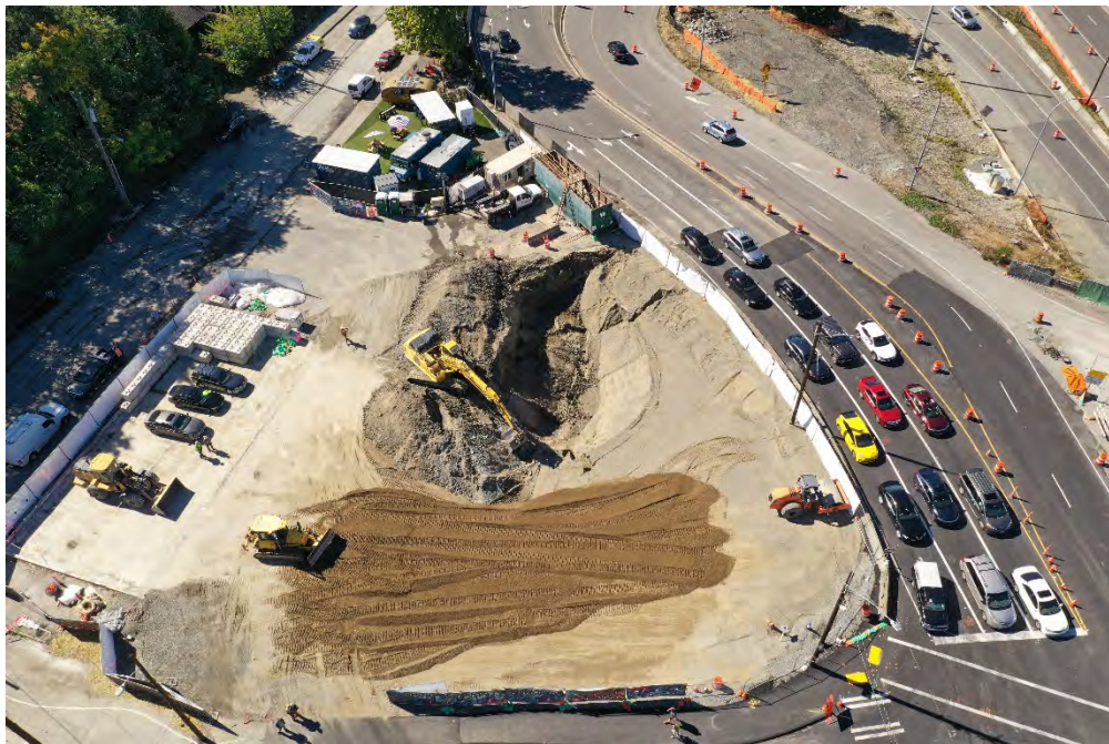
Photo 20. Over excavation of sample location B2. Majority of Stage 1 and 2 excavation backfill complete. Wall casting shadow in center of frame is location of soil sample X5.
