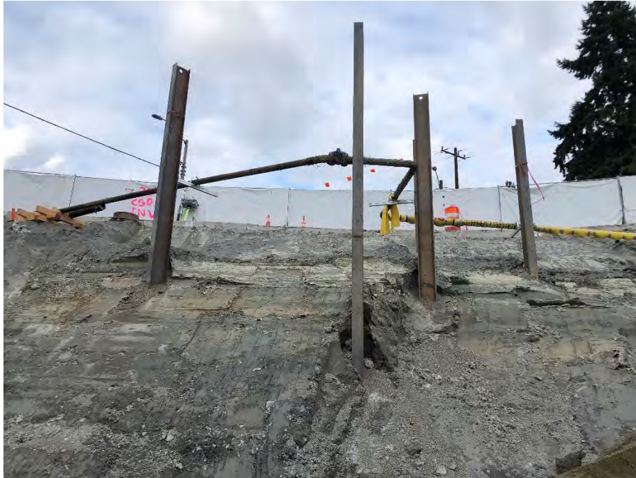
Photo 15. Erosion of soil surrounding westernmost H-pile supporting PSE gas line in place visible in foreground. Further excavation of east wall near sample location D6 deemed unsafe due to concerns regarding further undermining of gas line.
