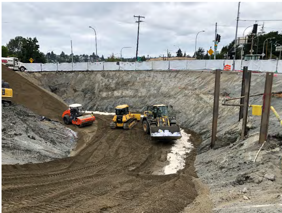
Photo 16. Placement of Oxygen Release Compound (ORC) along northern Stage 2 excavation boundary at a depth of approximately 20 feet below ground surface (bgs). ORC visible as white pellets in backfill along excavation wall prior to mixing with backfill. August 22, 2021.
