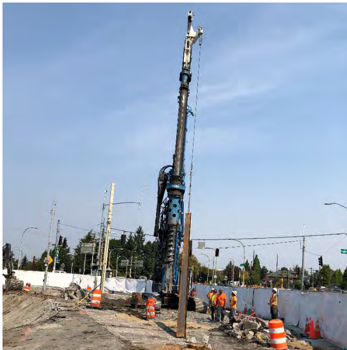
Photo 10. Installation of H-piles in right-of-way following temporary closure of East Montlake Place East for support-in-place of PSE gas line. August 12, 2021.
