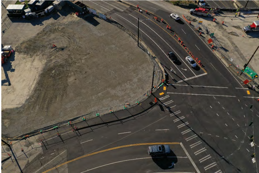
Photo 21. Site as seen looking west following completion of backfill, grading, paving, striping and placement of controlled strength base course for use as staging yard for greater SR520 Project. October 8, 2021.
